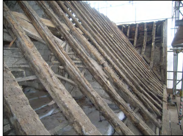
Plate 26: General view of north slope of Block B and side of gabled Block D
