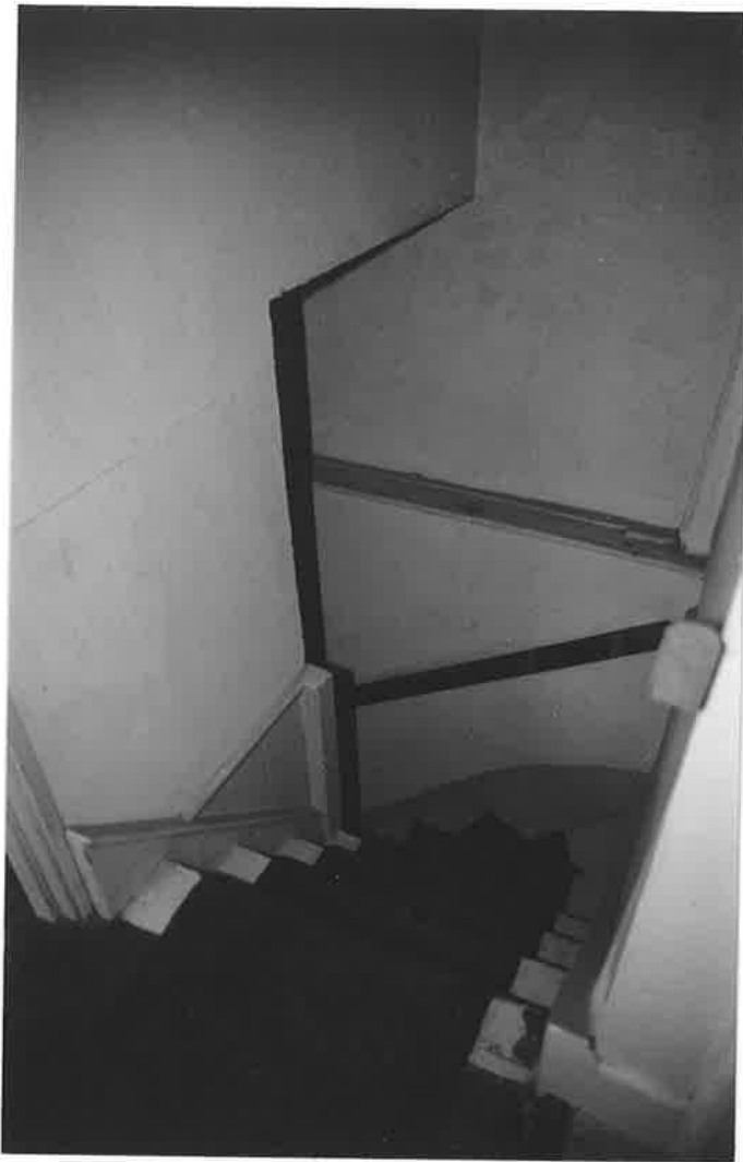
STAIRS, VIEWED FROM BLOCKED-OFF FIRST FLOOR ROOM WITHIN CROSS WING, R70 N30.
