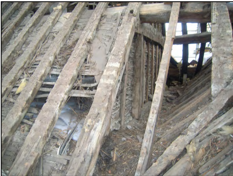
Plate 31: West end of Block B at junction with Block D (from N)
