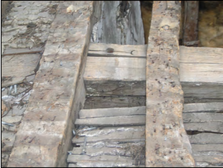
Plate 25: Pegs from scarf in purlin of Block B. North slope. Truss B2
