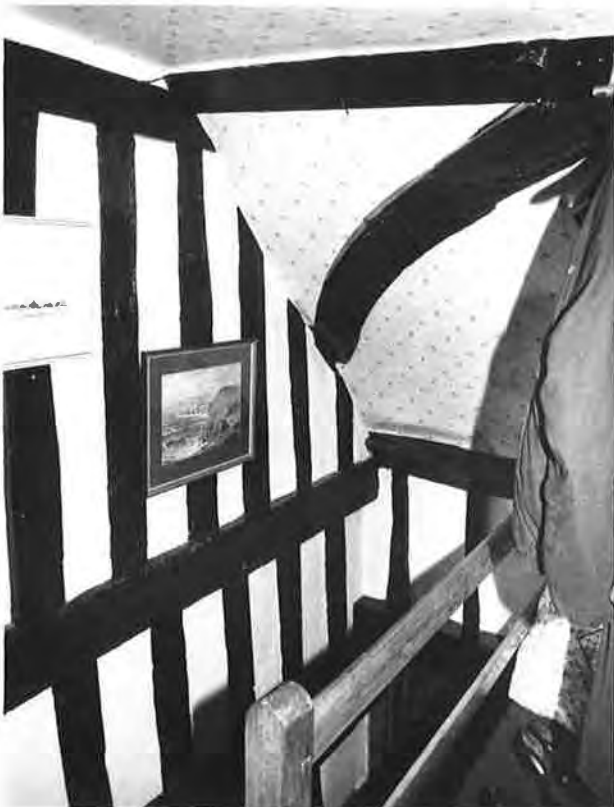
NO. 24. PARTITION BETWEEN STAIRS AND ROOM F, VIEWED FROM LANDING ROOM G. R227 N27.
