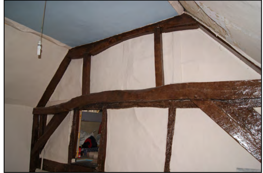
Plate 74: Open truss at west end of Block A adjacent to closed truss of Block B
