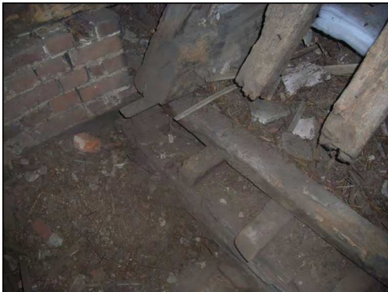
Plate 71: Roof void to west of chimney at north end of Block C.
