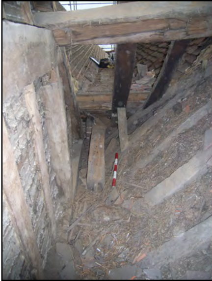
Plate 37: Junction between Blocks B and D with 'floating' wall plate projecting north from Block C
