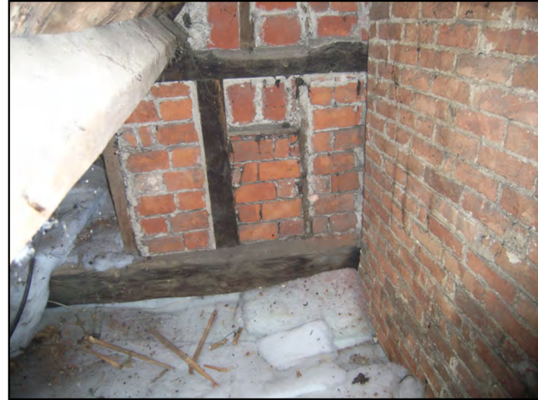
Plate 54: Brick nogging infill at north end of Block C (east side of chimney)
