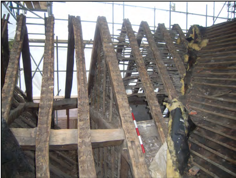
Plate 35: West end of Block B at junction with Block D. From south
