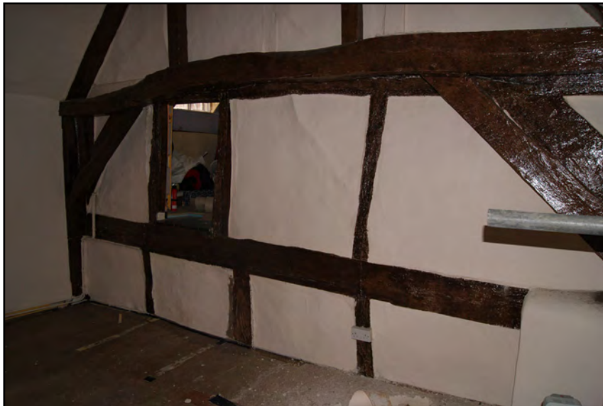
Plate 75: Open truss at west end of Block A adjacent to closed truss of Block B
