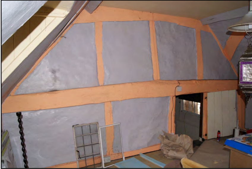
Plate 77: First floor cross frame and truss at east end of Block B
