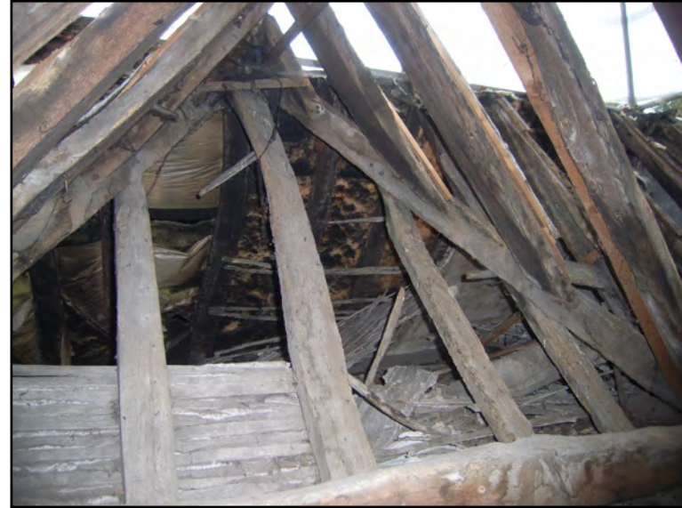
Plate 38: East slope of rafters of Block D overlain by roof of Block D
