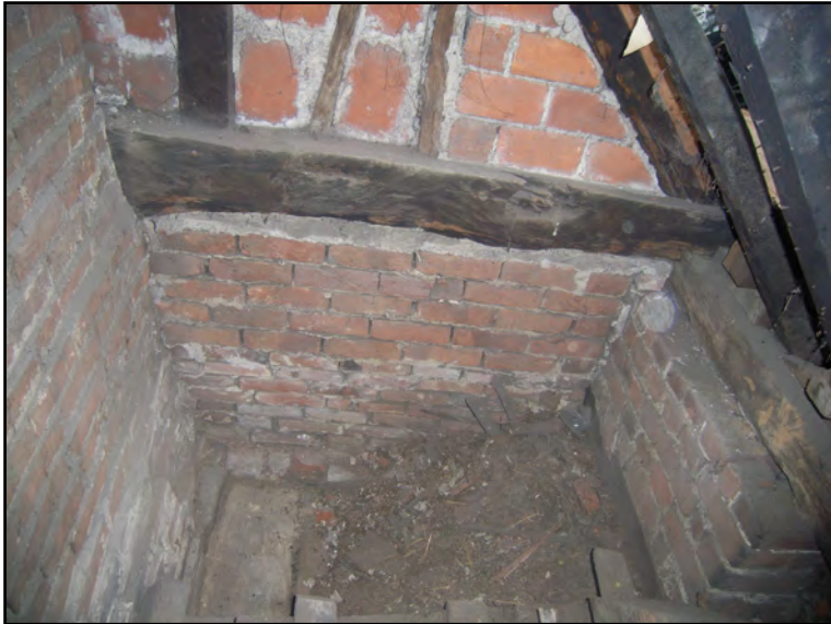
Plate 69: Roof void to west of chimney at north end of Block C. Looking south
