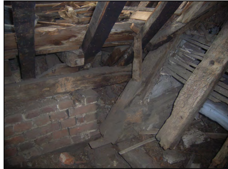
Plate 70: Roof void to west of chimney at north end of Block C. Looking west
