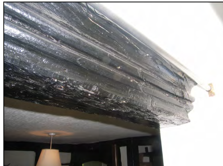
Plate 80: Moulded beam in Block E. Probably formerly faced open hall to west.
