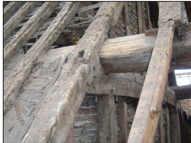
Plate 32: Clasped purlin detail at N end of truss at W end of Block B.
