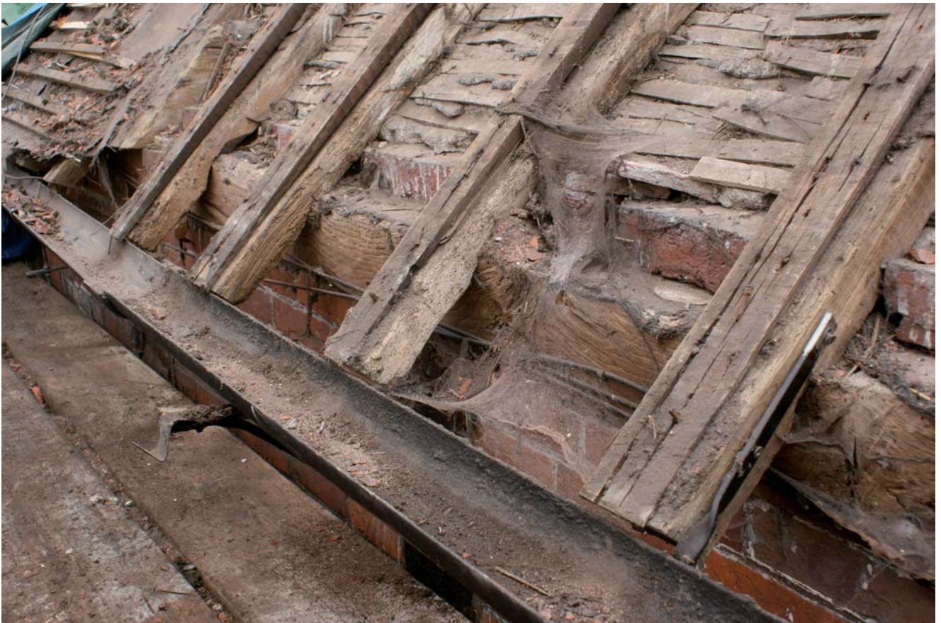
Plate 6: Rafter feet in west slope of southern bay
