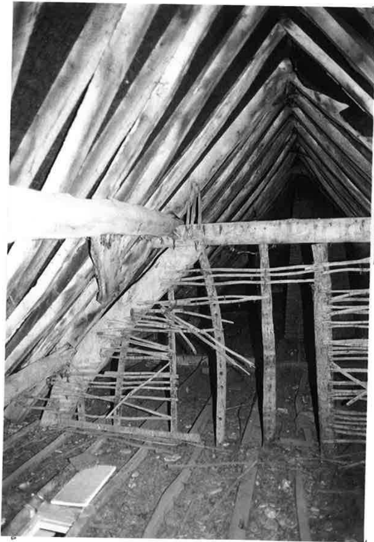
INTERNAL ROOF STRUCTURE LOOKING SOUTH SHOWING REMNANT OF EARLIER CRUCK TRUSS. R. 251 N. 23.
