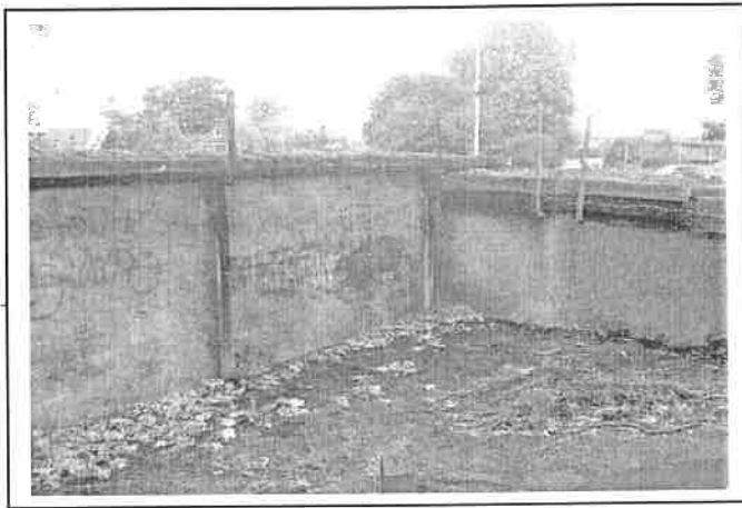
Plate 7: East wall of former mill (to left) and rear face of front wall of former mill house
