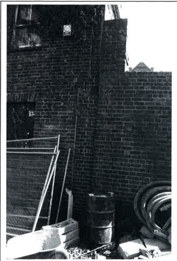
Plate 9: Straight joints at south-west corner of primary building, visible after removal of ivy
