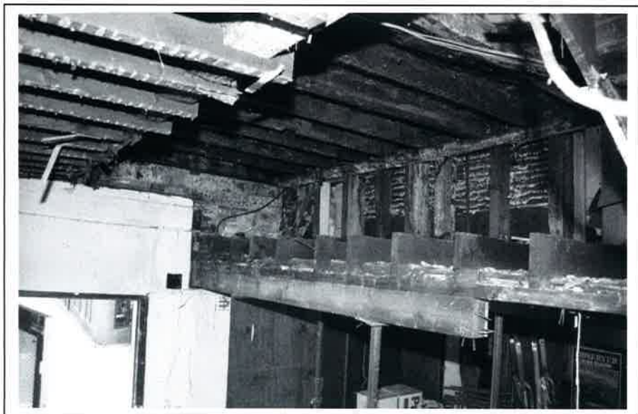
Plate 19: View of low 'cupboard' beneath F2 and accessible from F1 after removal of ceiling
