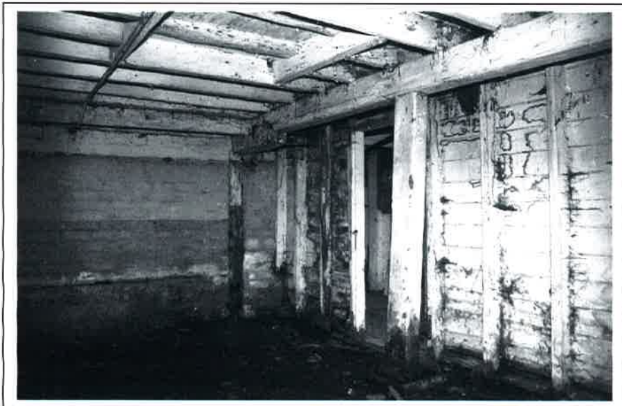
Plate 13: View within C2 from north-east showing trap-door and rough scarf in main beam adjacent to secondary brick cross-wall
