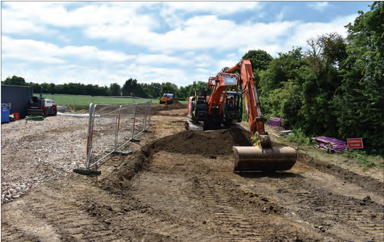
Plate 8: Topsoil stripping at the eastern end revealing an area of disturbance 7, looking west
