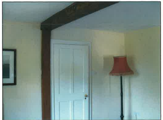
Plate 10: Dining room: wall proposed for removal
