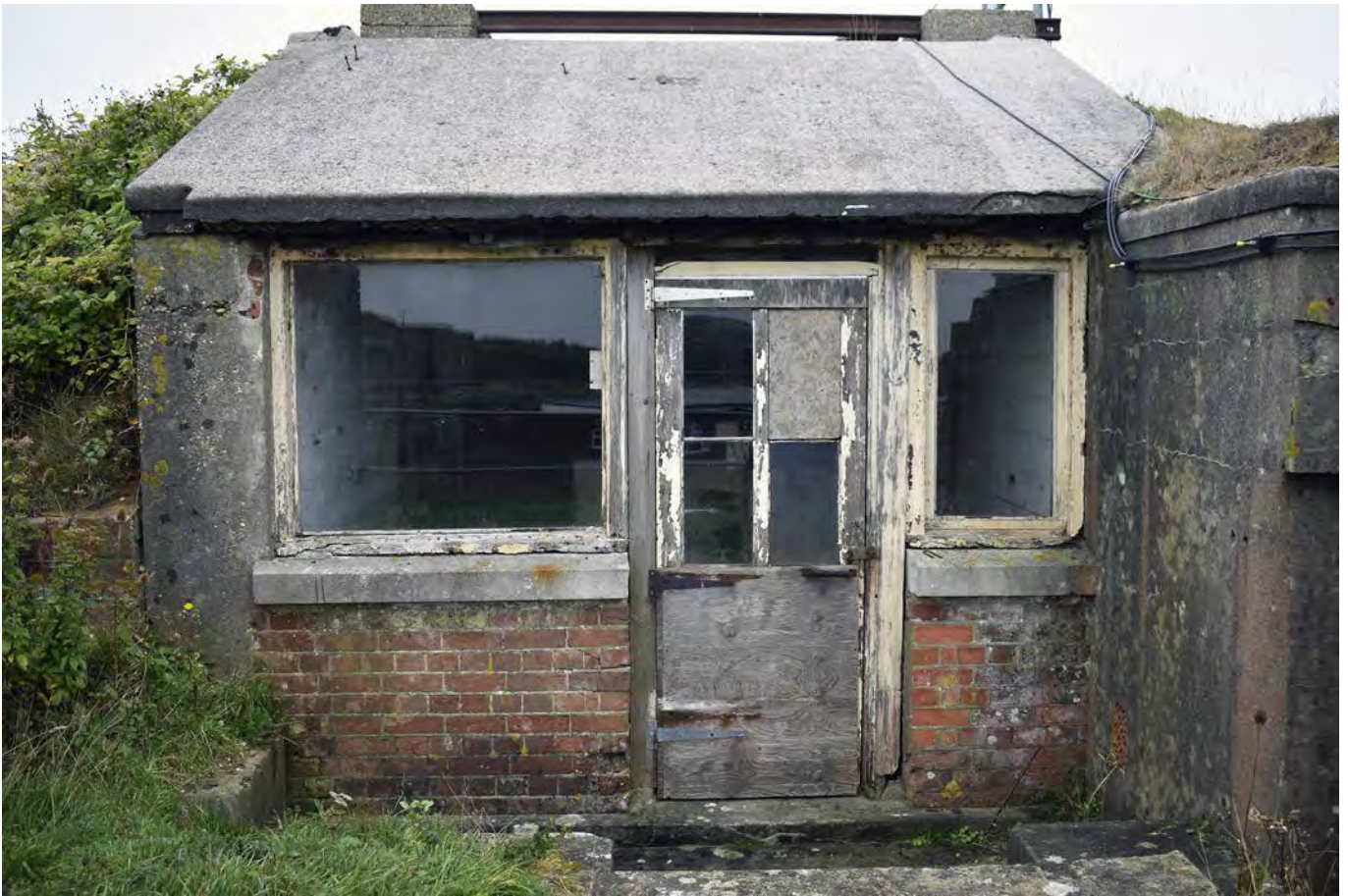
Plate 53: Position Finding Cell, external view
