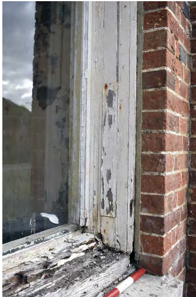
Plate 8: Bay A, opening A3, showing deteriorated sill
