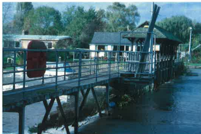
Plate 8: South-west view of east paddle rack
