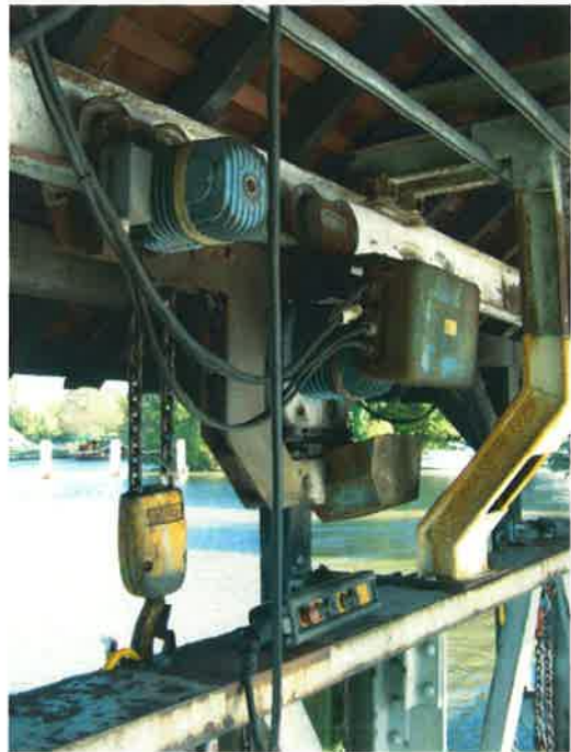
Plate 14: North-east view of buck gate weir electric motor
