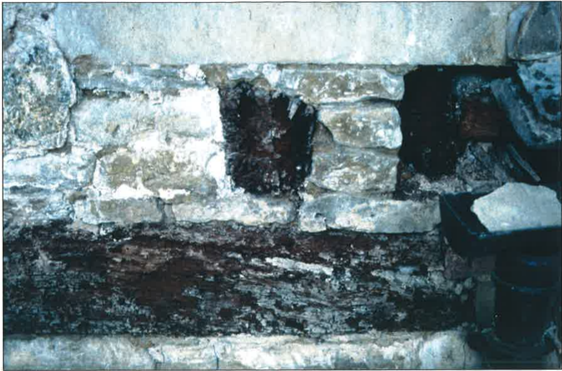
Plate 20: West elevation second floor showing exposed timbers
