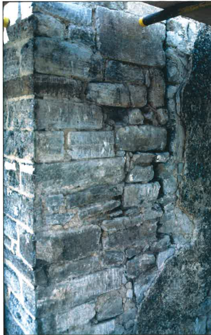
Plate 13: East elevation, second floor showing break in stonework
