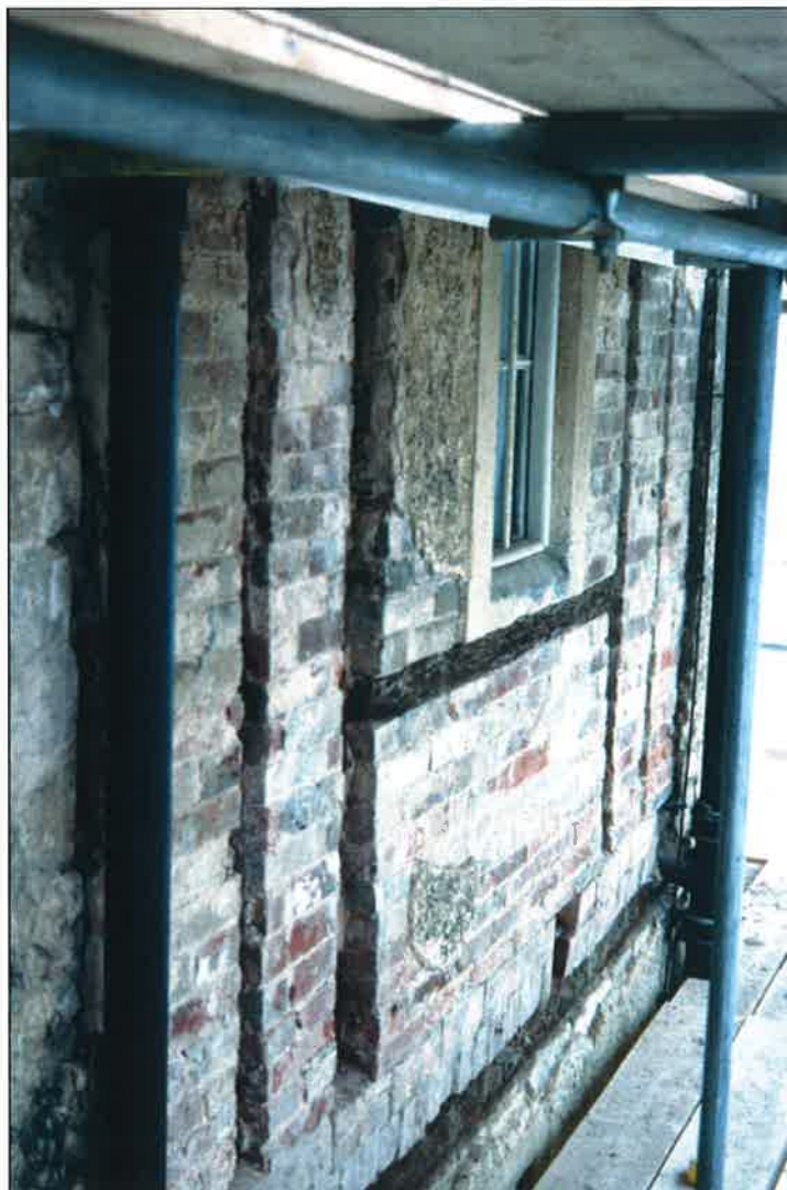
Plate 16: West elevation, first floor showing red brick repair
