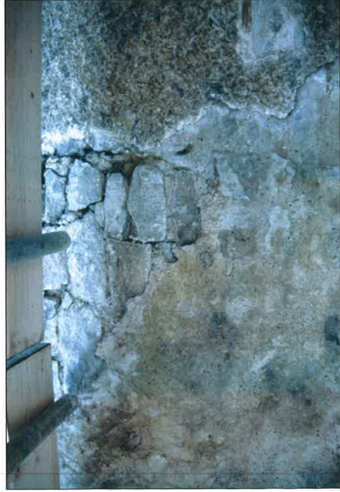
Plate 3: North elevation, first floor showing break in stonework at west end.
