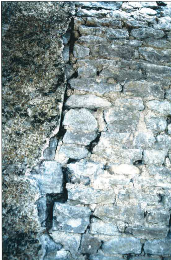
Plate 6: North elevation, second floor showing break in stonework
