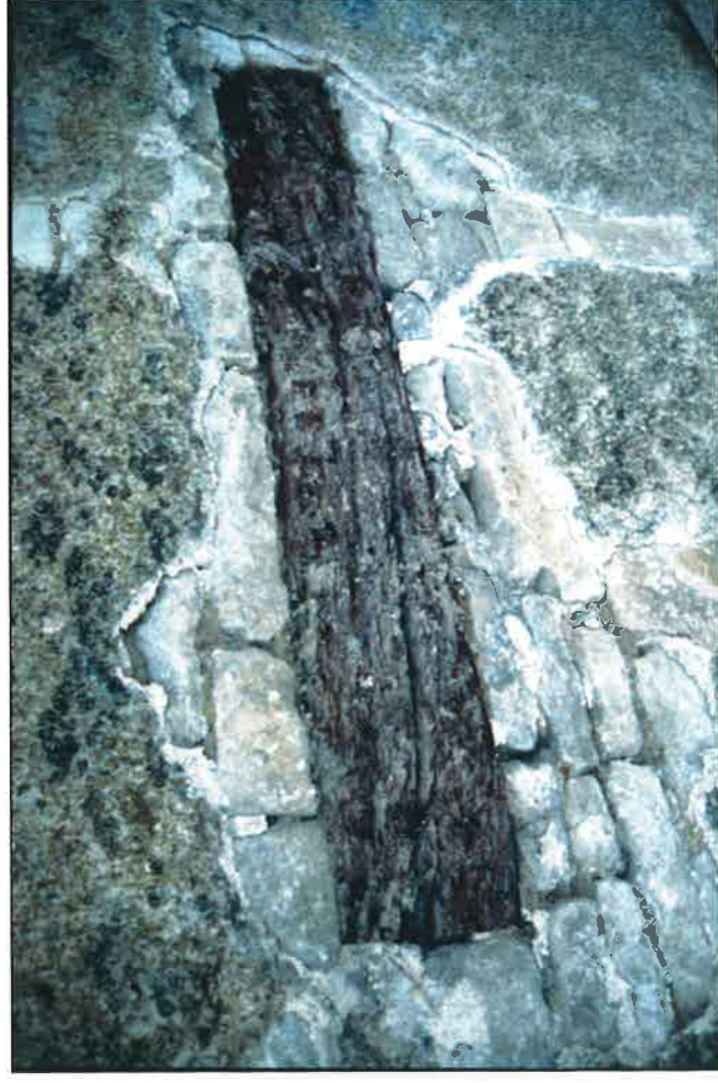
Plate 4: North elevation, first floor showing exposed timber.
