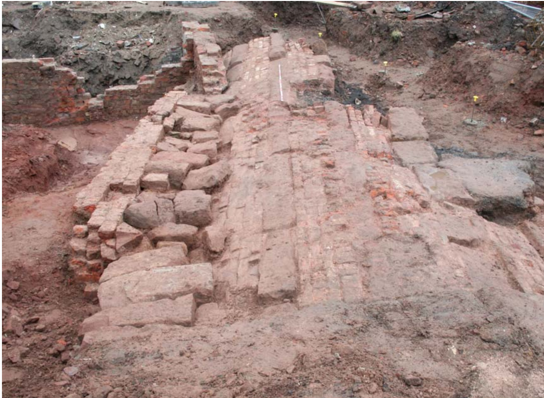
Plate 10: West-facing view across the collapsed arch of Tunnel 1 ( I25 ) showing the 'composite style' of construction using brick and sandstone I24
