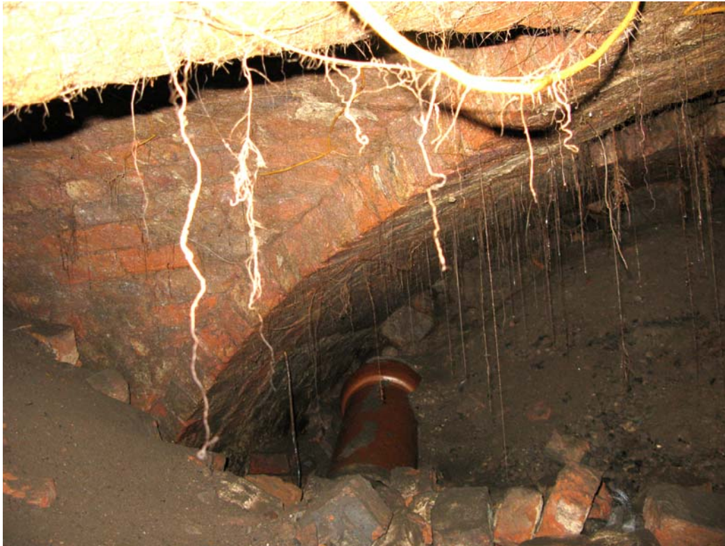
Plate 14: East-facing shot inside Tunnel 1, 125 , showing the interface with Tunnel 2, 176 , to the left of the picture
