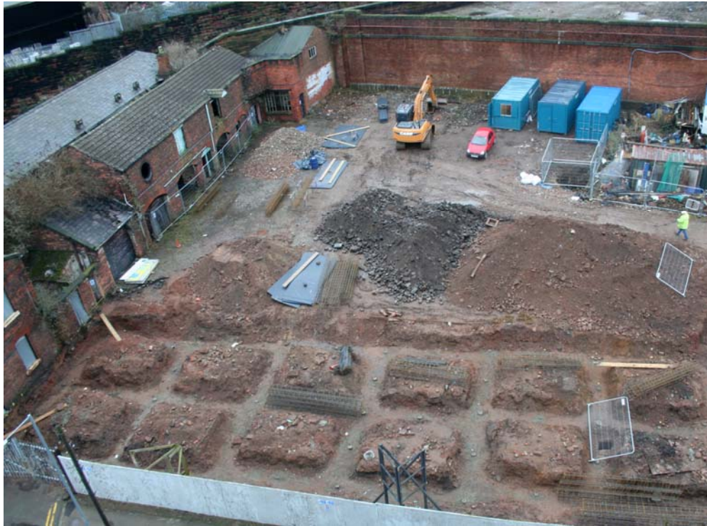
Plate 1: East-facing aerial view across the stable yard during the watching brief investigations
