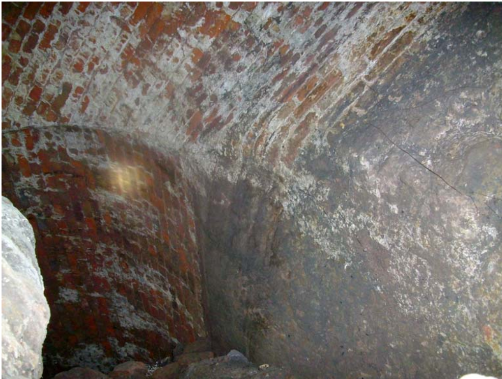
Plate 30: Interior view of vaulted Tunnel 4, 300 , accessed via the Triple Decker section of Tunnel network
