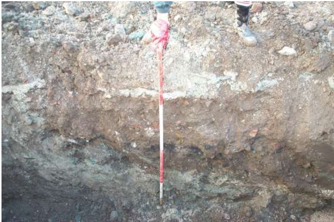
Plate 4: West-facing Section of sewage trench detailing contamination
