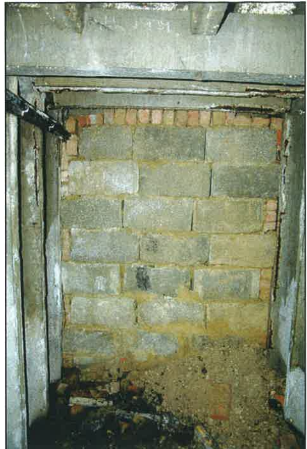
Plate 3: Northern shelter, infilled entrance.
