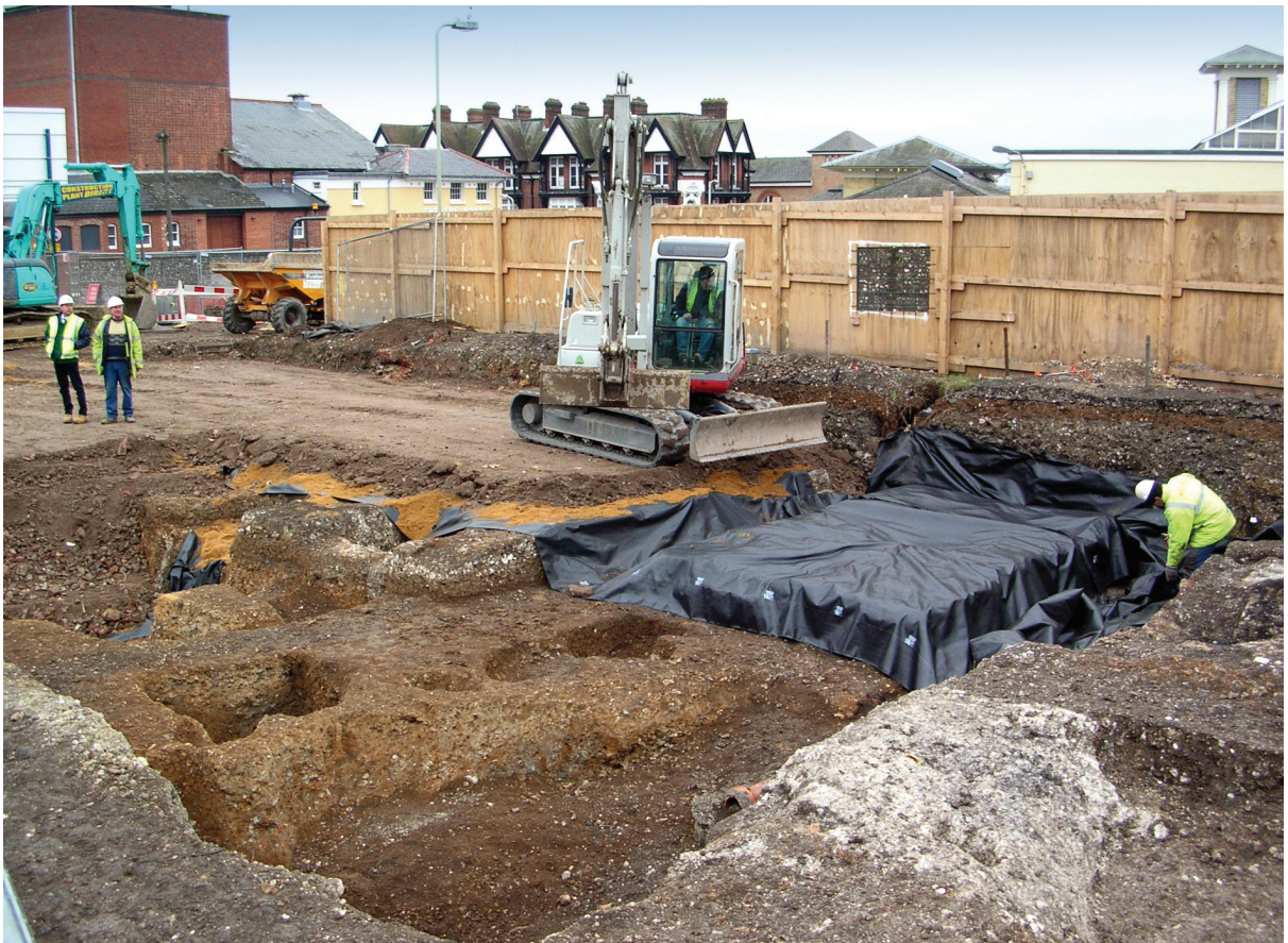
Plate 1.5 View looking north-east showing the process of preservation in situ of deposits along the east side of Staple Gardens frontage on the Northgate House site
