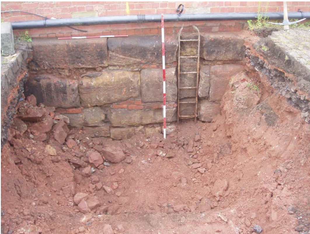
Plate 6: Trench 402, showing south wall of Manchester Dock, 3053 , below the GWR building, looking south
