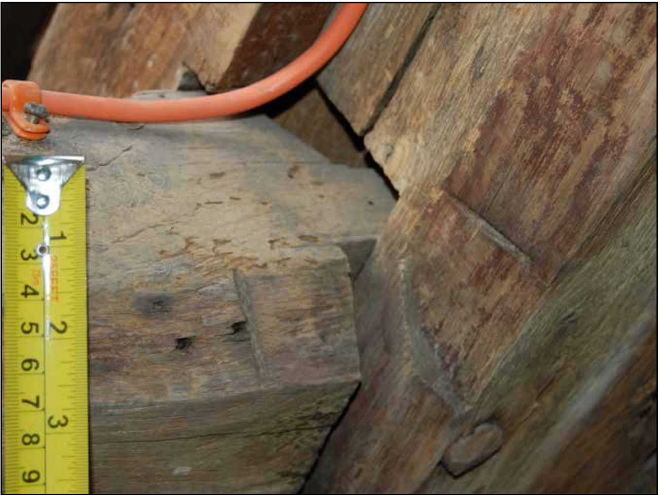
Plate 67: Detail of carpenter's marks on the west principal rafter and purlin of Truss 1, Roof 2
