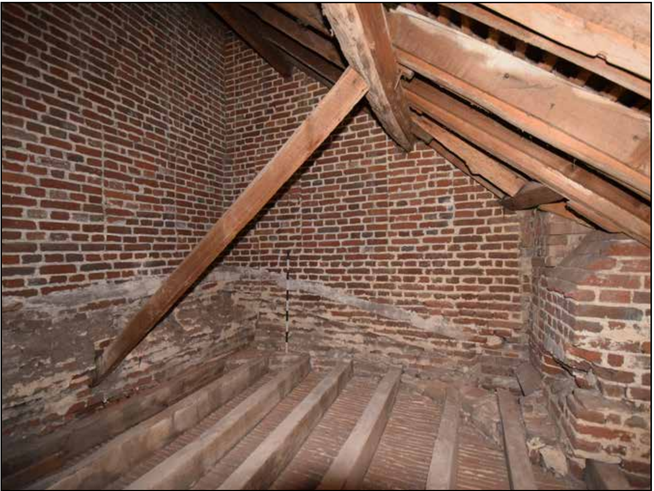
Plate 77: General view of east space, Roof 4, showing lower roof structure, looking north east
