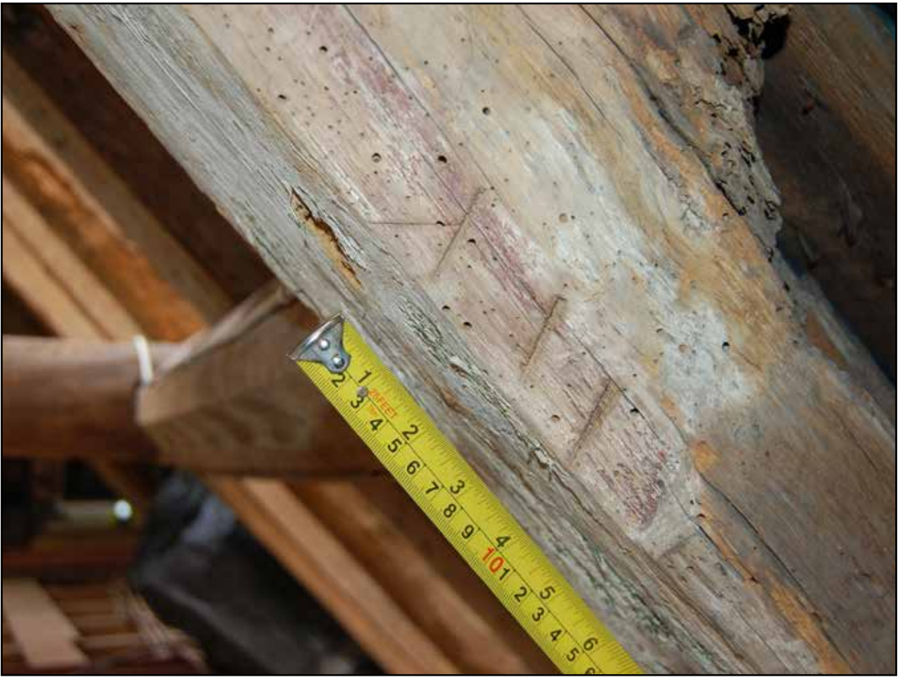
Plate 69: Detail of carpenter's marks on the east principal rafter of Truss 3, Roof 2
