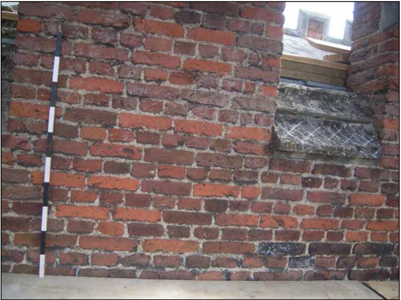
Plate 9: Mixture of Brick Type B and Brick Type V on Base Court parapet
