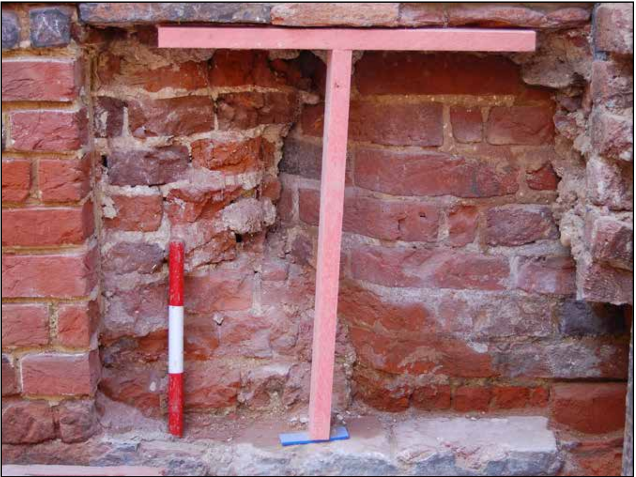
Plate 15: Exposed Daubeney turret in the ground floor of Clock Court East Facing Elevation – Part 1
