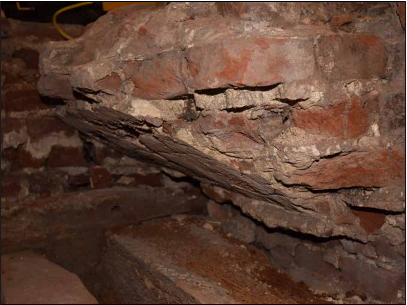
Plate 41: Roof 4 detail of vault like structure, south east corner of west space
