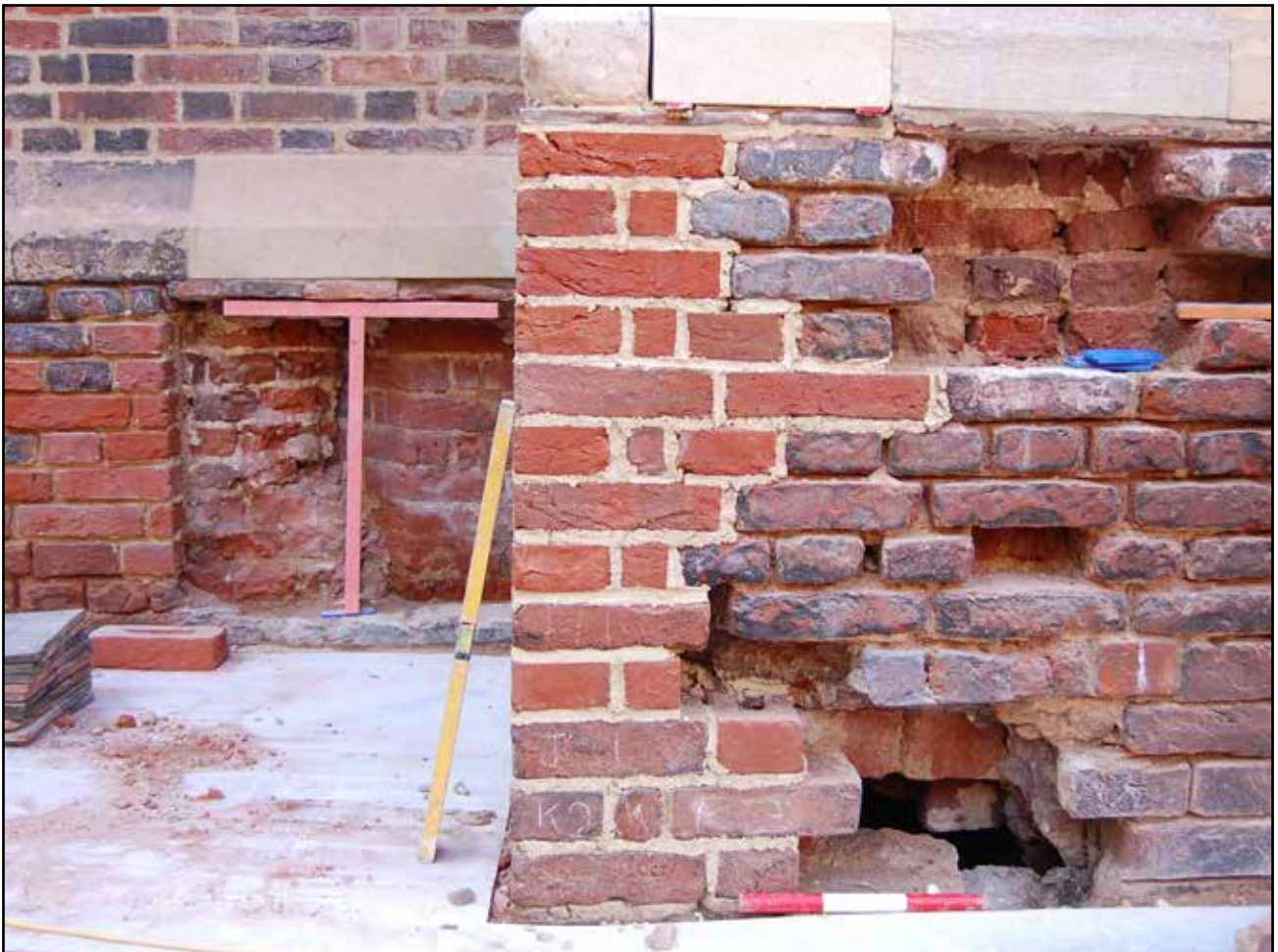
Plate 20: Opening into vault in relation to exposed Daubeney turret in the ground floor of Clock Court East Facing Elevation – Parts 1 and 2, looking west
