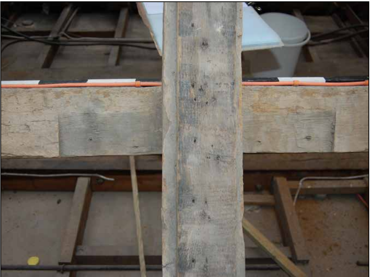
Plate 58: Trenches for wind braces in the east purlin of Bay 1, looking west
