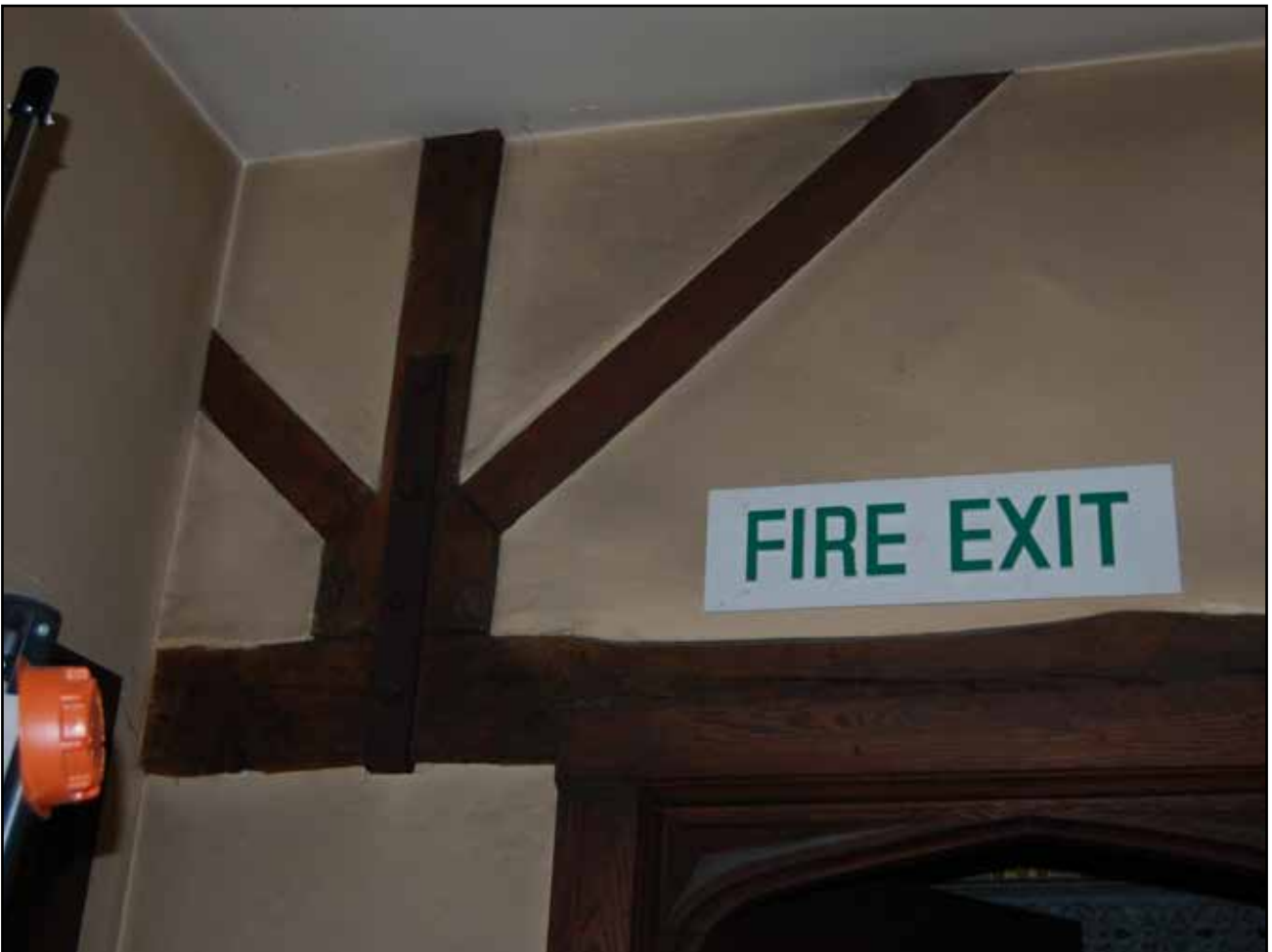
Plate 80: Second Floor room under Roof 2 showing 20th century support under Truss 3, looking south
