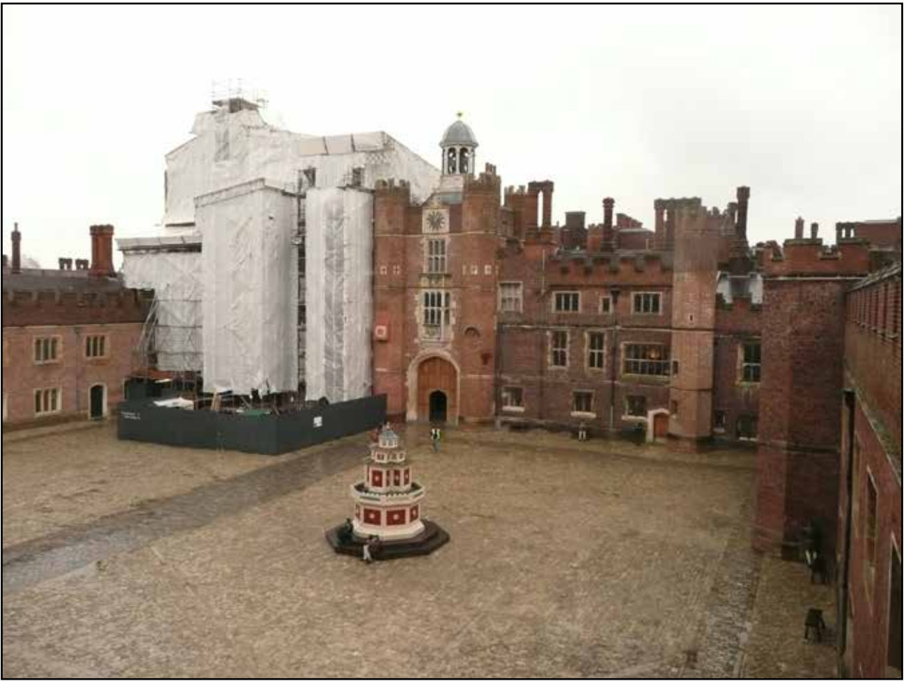
Plate 1: General view of west facing elevations of Base Court, looking north east
