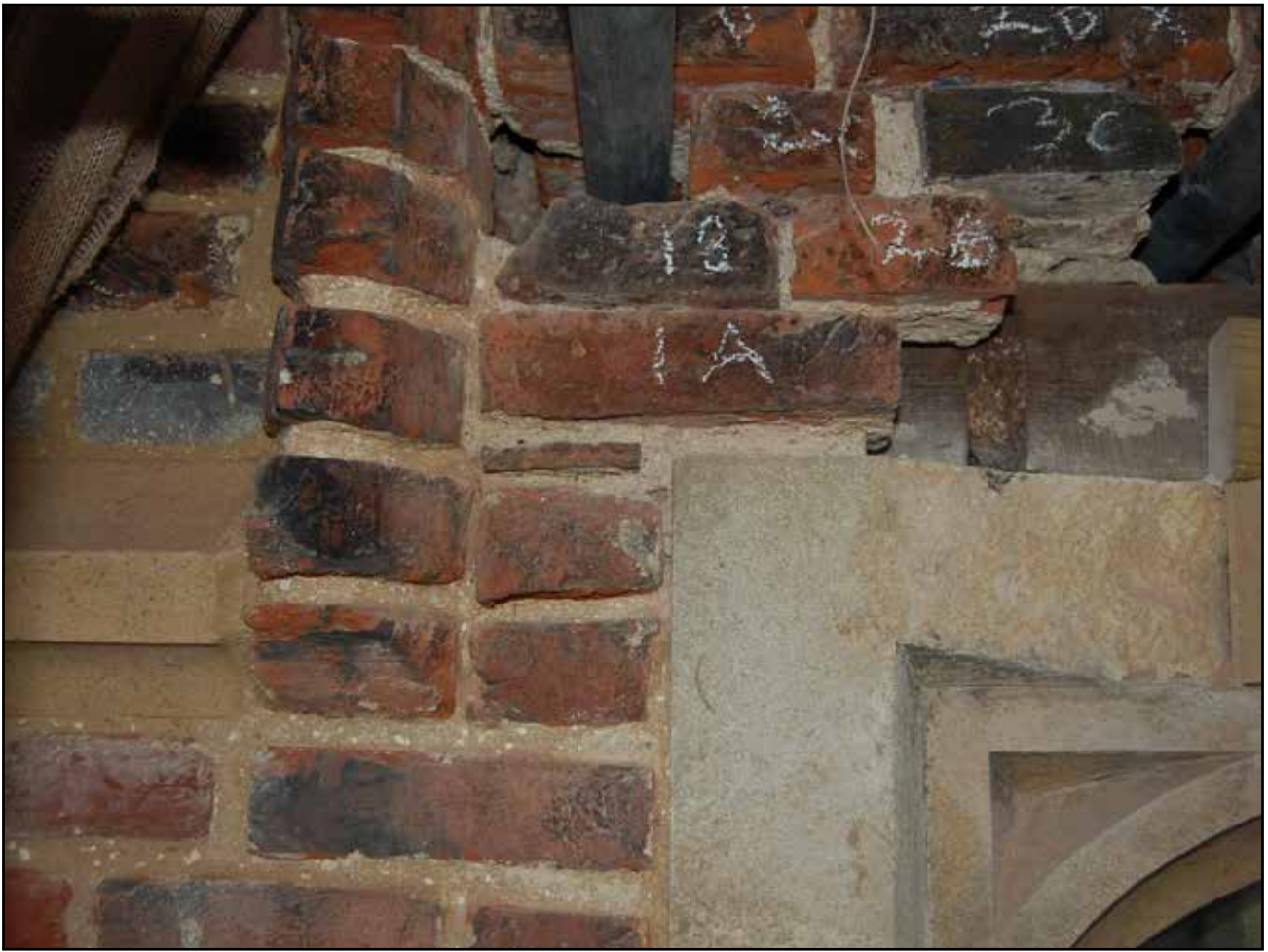
Plate 7: Base Court - West facing Elevation Part 1, Second floor hood mould, looking east
