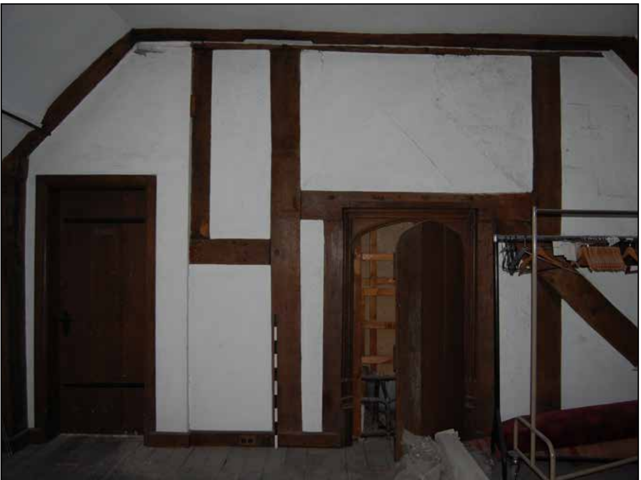
Plate 78: Second Floor room showing dividing wall under Truss 3 of Roof 1 and Truss 1 of Roof 2, looking north
