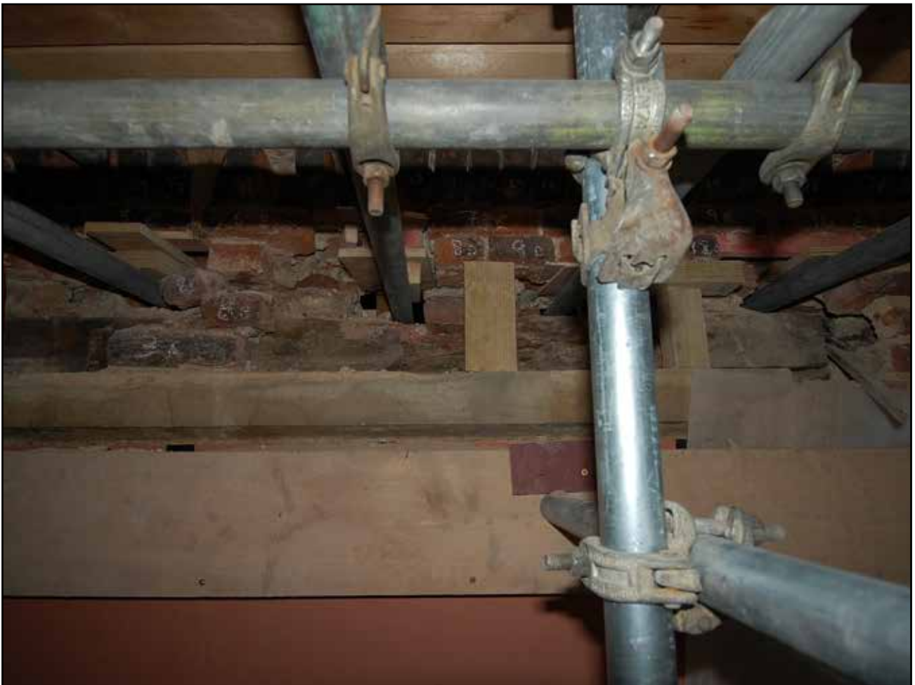
Plate 82: Exposed lintel under brick hood mould in Second Floor of Base Court – West Facing Elevation, Part 1
