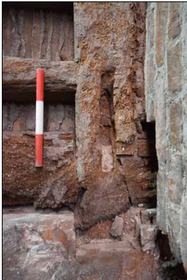
Plate 76: Dove tail joint in north west corner of lower roof structure, west space, Roof 4
