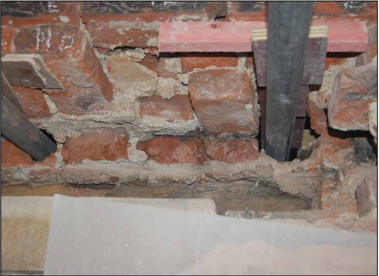
Plate 83: Exposed brickwork behind lintel under brick hood mould in Second Floor of Base Court – West Facing Elevation, Part 1
