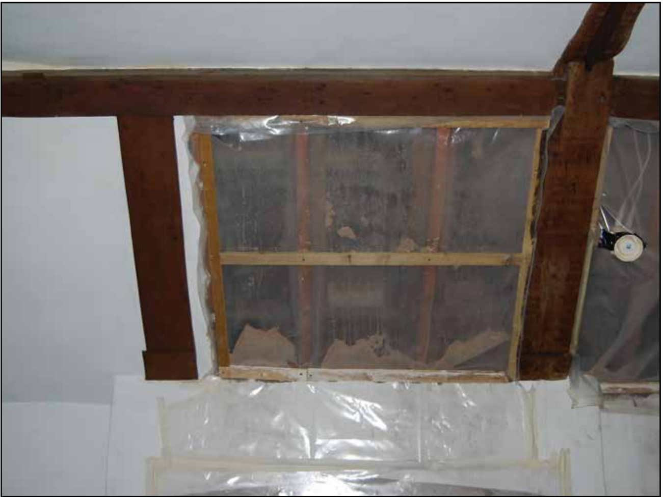
Plate 79: Second Floor room under Roof 2 showing exposed principal rafter feet, looking east
