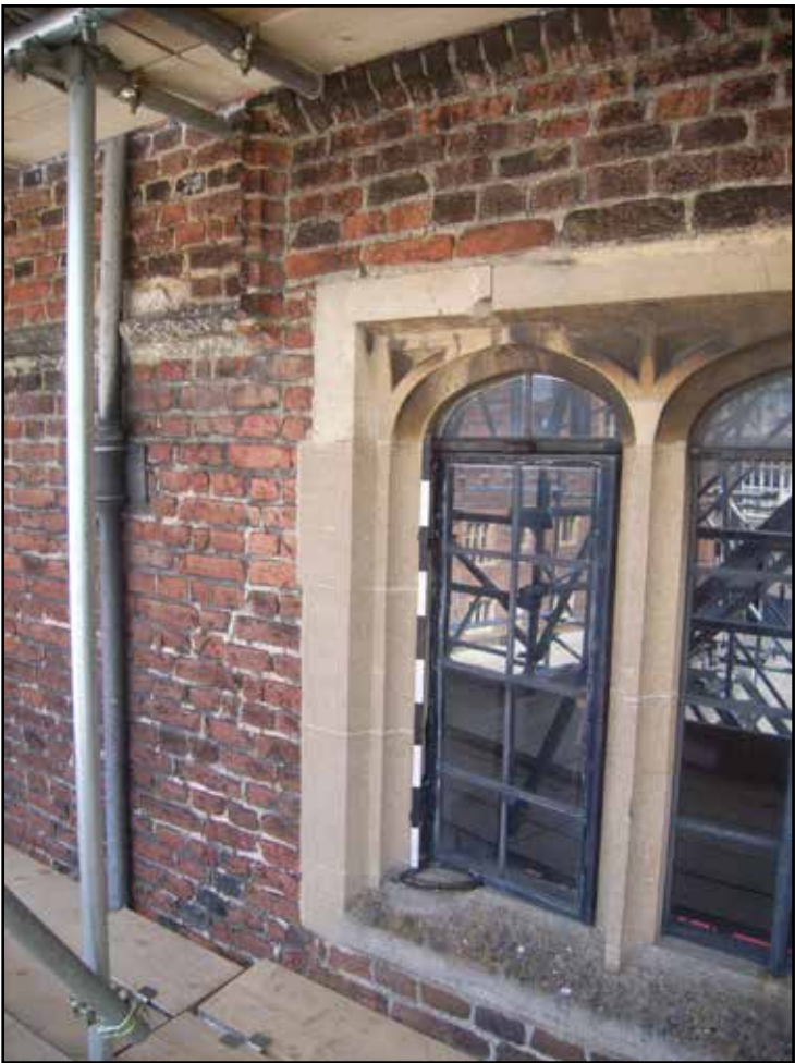
Plate 6: Base Court - West facing Elevation Part 1, Second floor hood mould, looking east
