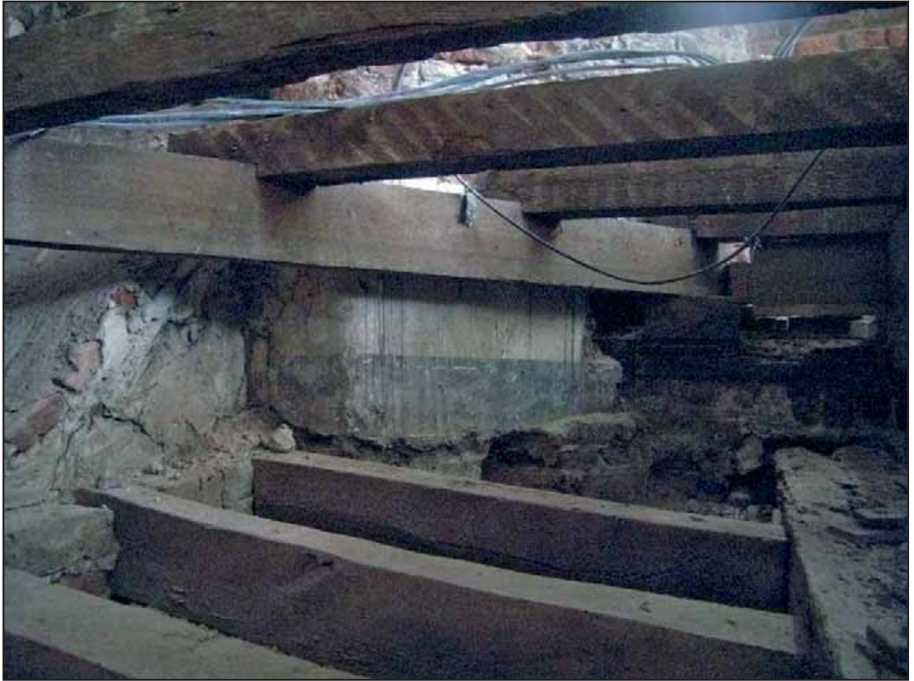
Plate 19: Buttery Return Wall showing plaster and impression of skirting on north face, looking south west
