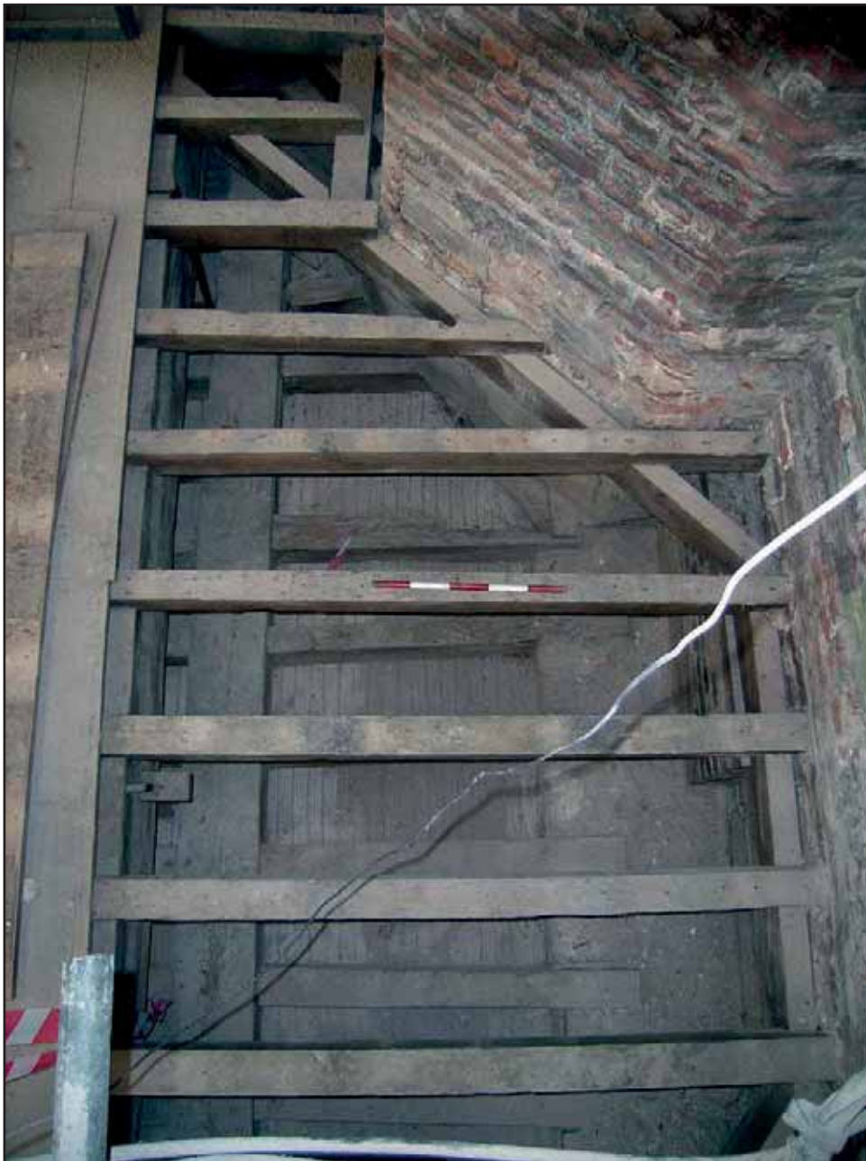
Plate 33: The south end of the Flat Roof where it meets Turret 16, from above
