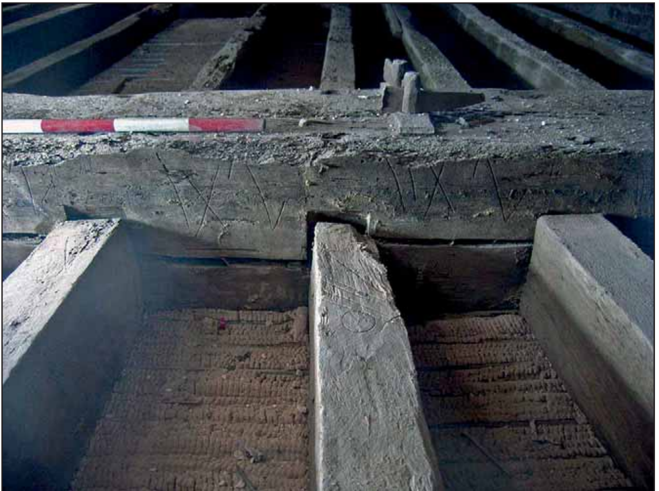
Plate 30: Carpenter's marks on the south side of Tie Beam 3 and its joists, the Flat Roof, looking north
