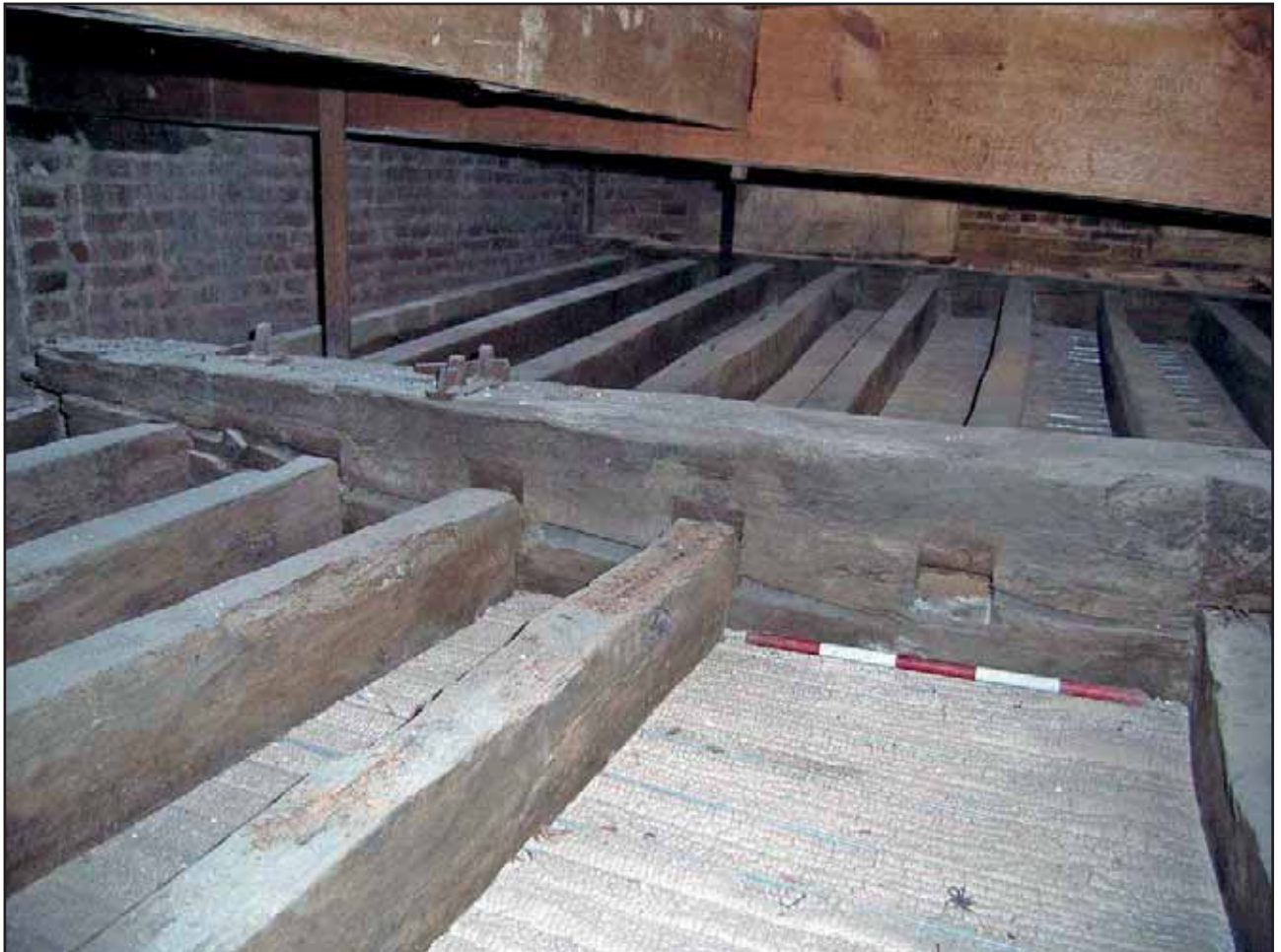
Plate 28: The Upper and Lower structures of the Flat Roof, looking south east
