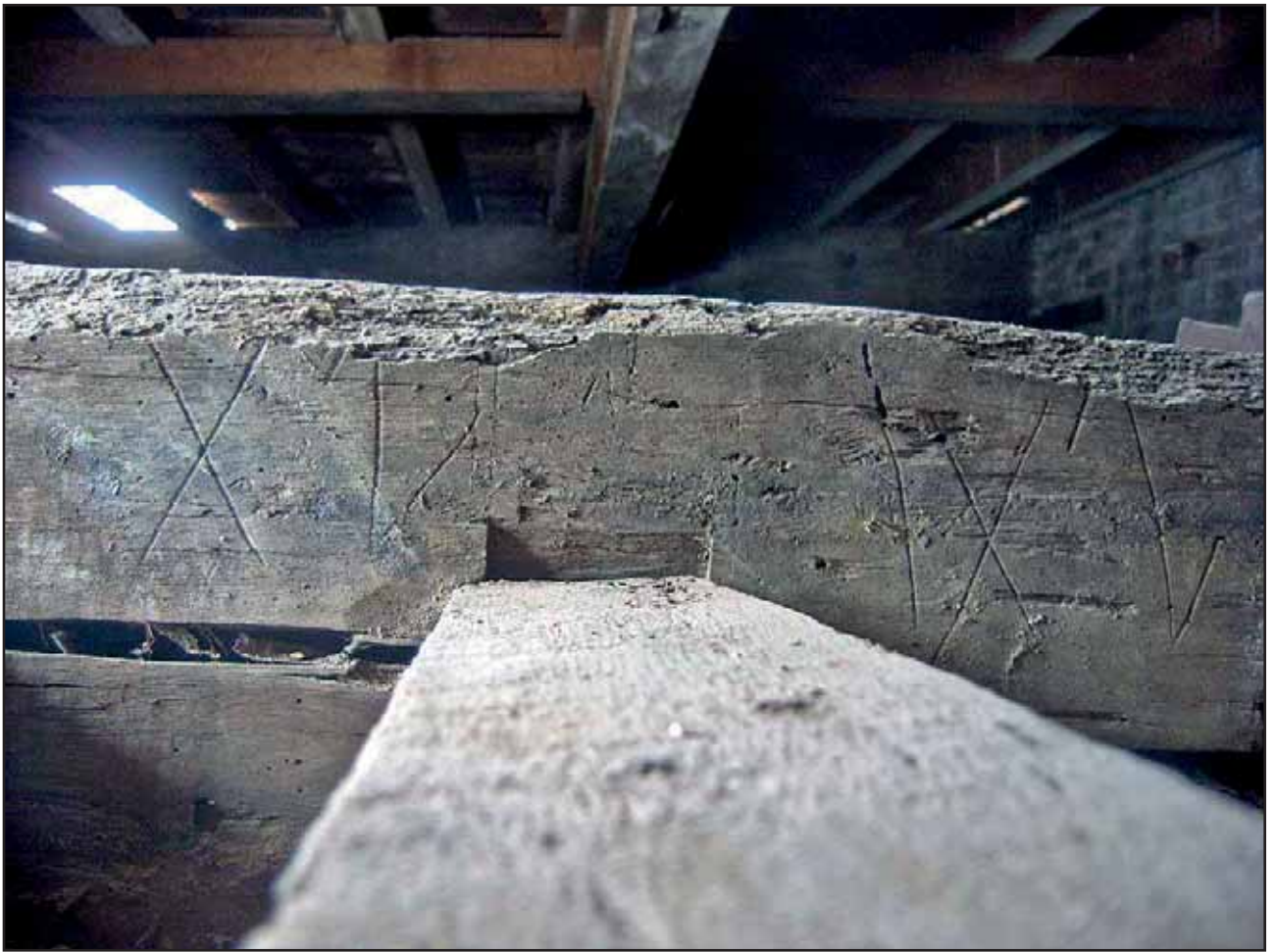
Plate 29: Carpenter's marks on the south side of Tie Beam 3 and its joists, the Flat Roof, looking north
