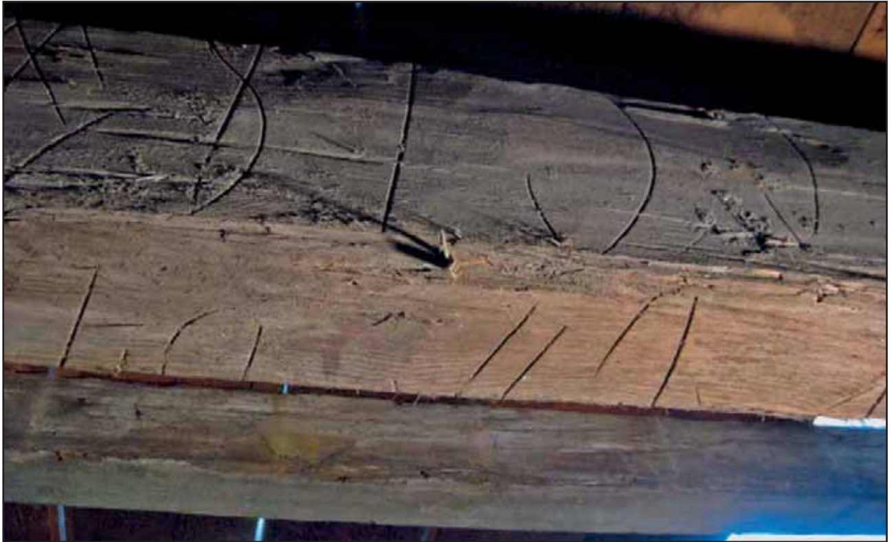
Plate 35: Baltic Marks on the east and under side of joist in Bay 2 of the Upper Structure of the Flat Roof
