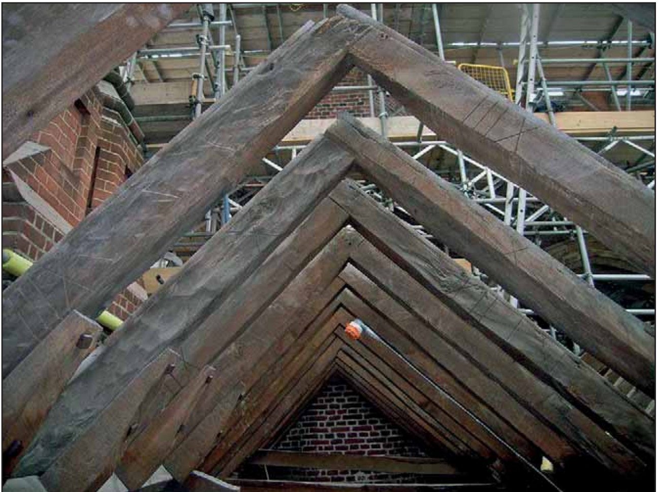
Plate 26: Common rafters of Bay 2 of the west side of the Main Roof, looking north
