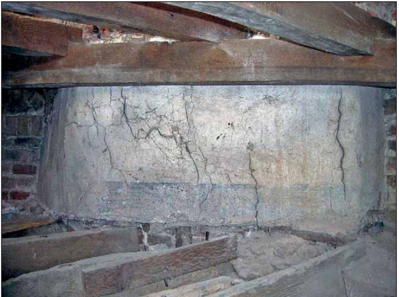
Plate 20: Buttery Return Wall showing plaster and impression of skirting on north face, looking south east
