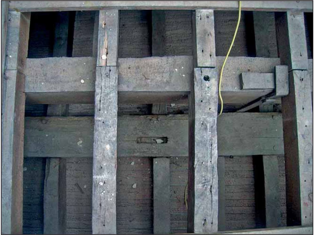
Plate 27: View from above of the Upper and Lower structures of the Flat Roof
