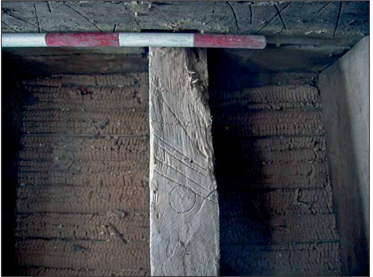
Plate 31: Carpenter's marks on the south side of Tie Beam 3 and its joists, the Flat Roof, looking north
