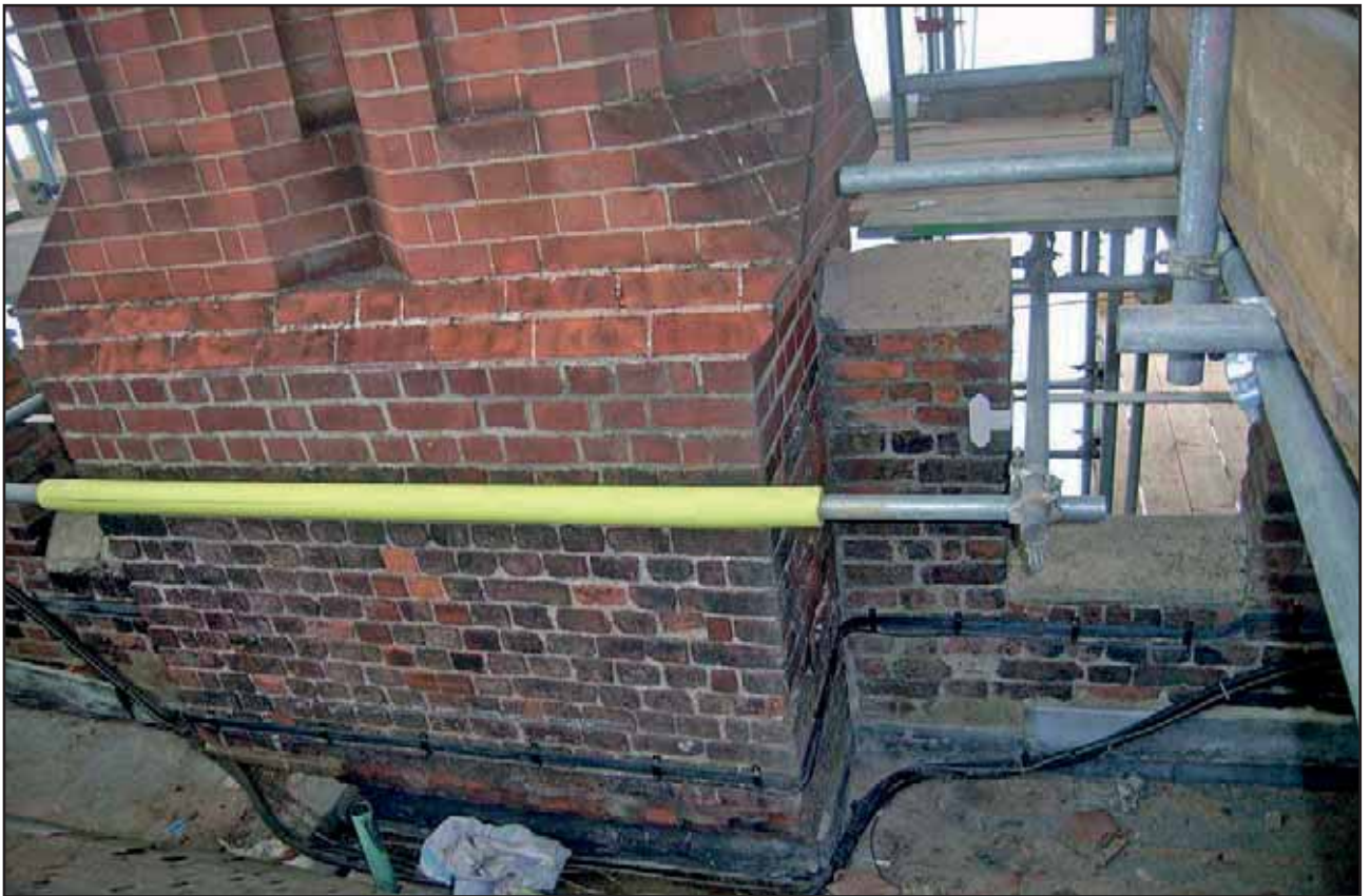
Plate 9: Internal parapet and chimney stack of West facing Elevation Part 3, Base Court, looking south west
