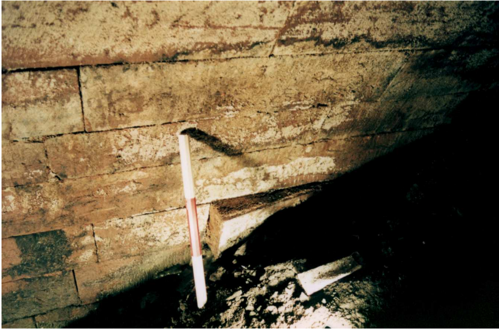
Plate 11 Dislodged block on the north side of Tunnel 10
