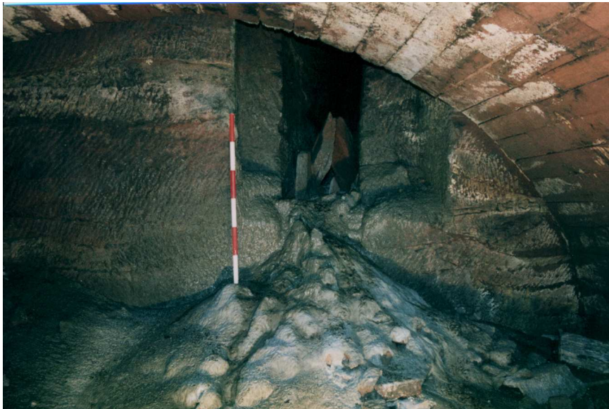
Plate 8 Interior of Tunnel 10, southern passage entrance, taken following the piling – looking east
