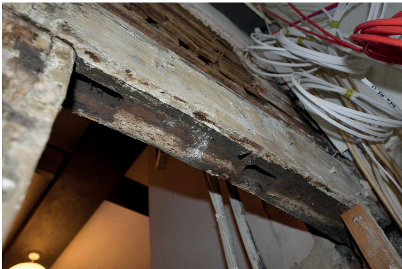
Plate 6: Empty mortices to underside of rail in frame
