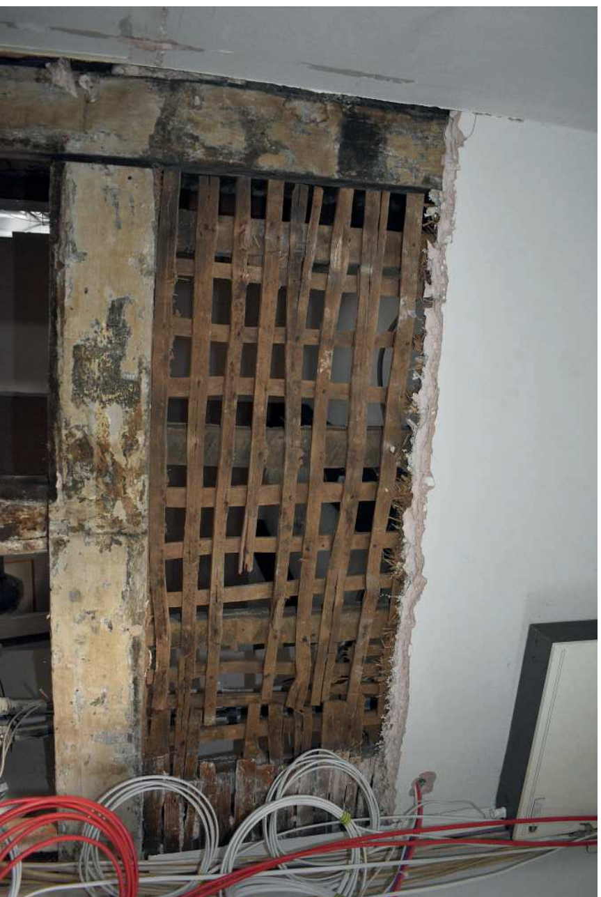
Plate 4: laths to east side of exposed frame
