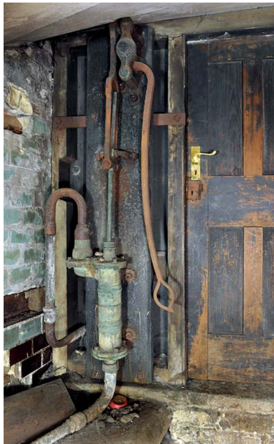
Fig 84a (left) Nos 11-12 Blomfield Street: The hand crank for hydraulic lift found below the geometric staircase
