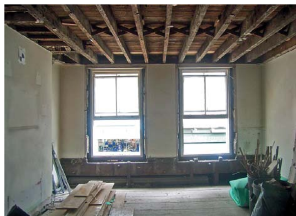
Fig 19 View of the first floor of No. 94 Dean Street, looking east towards the street
