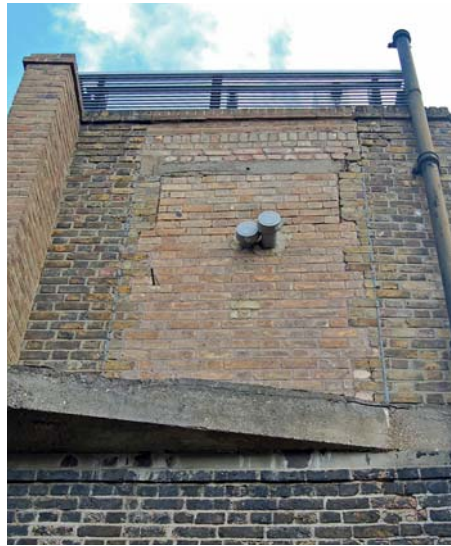
Fig 62 Nos 8-9 Hayne Street: left) the street frontage, right) detail of the rear of the building showing blocked doorway and the remains of the bridge constructed by the Great Western Railway to link to the back of No. 4 Lindsey Street
