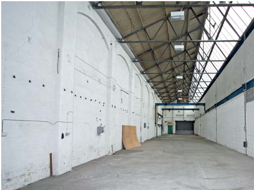
Fig 77 The former East London Soap Works, Bow; interior of a factory building with evidence of travelling crane rails
