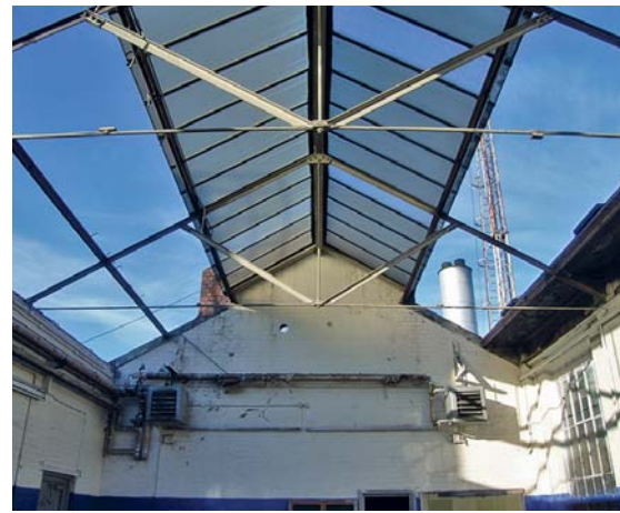
Fig 63 Simple and lightweight: the roof to the southern sand furnace house. Although both the sand house and engine shed were present when the depot opened in 1906 the sill on the engine shed window to the right of the photograph suggested that the sand house was an afterthought
