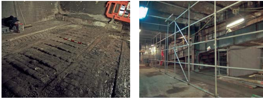
Fig 84 The remains of the London Street milk ramp (with stone sett surface) prior to removal
