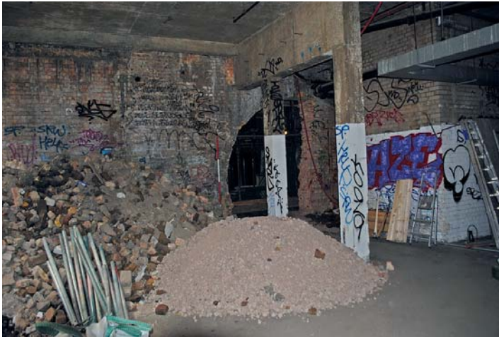
Fig 89 The brick-built structure beneath No 3 Lindsey Street included a blocked-up archway which originally led to the railway sidings
