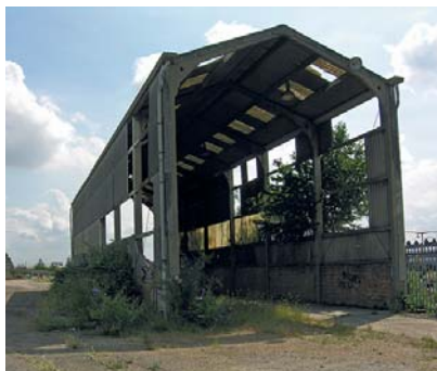
Fig 126 A 1970s goods shed at Plumstead Goods Depot shortly before its demolition in 2012
