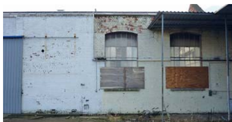
Fig 52 The north wall of one of the depot's two sand houses was formed from the south wall of the engine shed. It survived in fragmentary form until 2011
