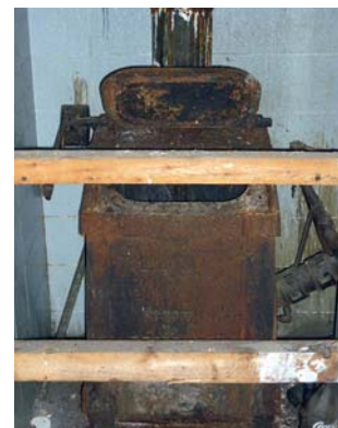
Fig 122 An interesting feature of the New Amenity Building was an incinerator set into a recess in the wall of the main first-floor office. This had been fabricated by Heenan and Froude of Worcester, and was labelled a 'Horsfall No 5 Destructor'
