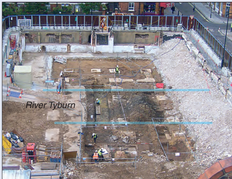
Fig 26 The buried course of Tyburn River revealed by a black silt fill exposed during Crossrail excavations at Bond Street
