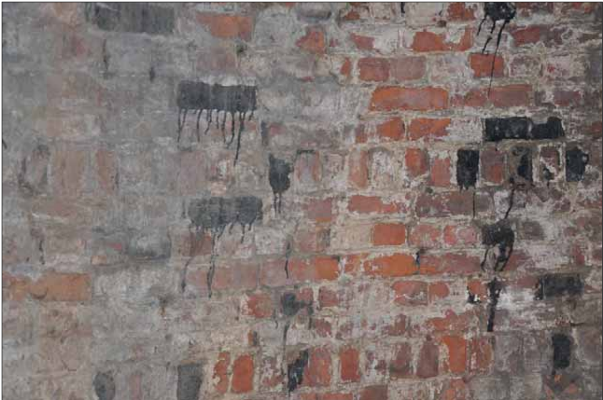
Plate 25: Remains of whitewashing on ground floor walls
