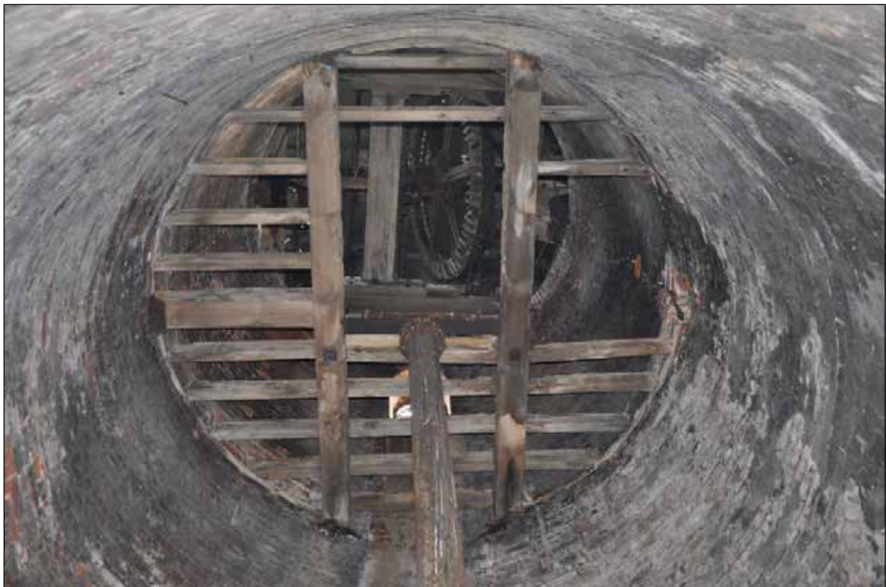
Plate 26: Remains of first and second floor timber floor structures
