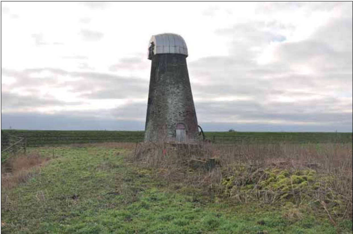
Plate 24: Remains of brick structure just north of the mill, from the north
