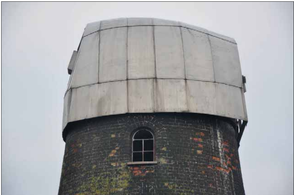
Plate 22: Aluminium cap roof replacement and south-east side window to the third floor, from the south-east
