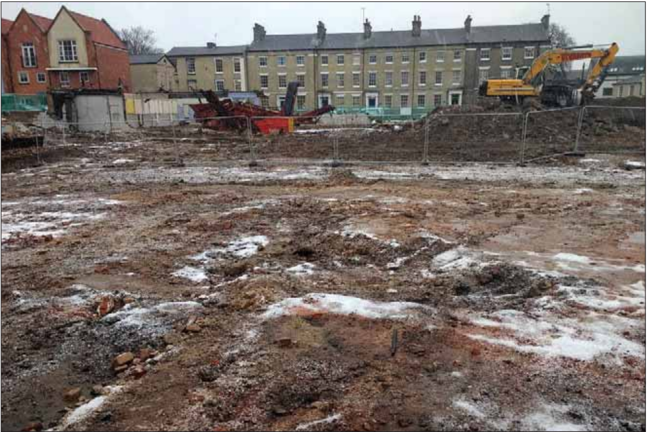
Plate 3: Northern extent of the development site, looking east towards Lower Brook Street
