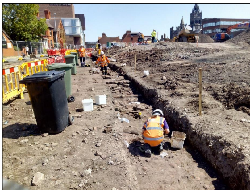
Plate 1: The surface-water drainage trench on the south side of Hunter Street, looking east
