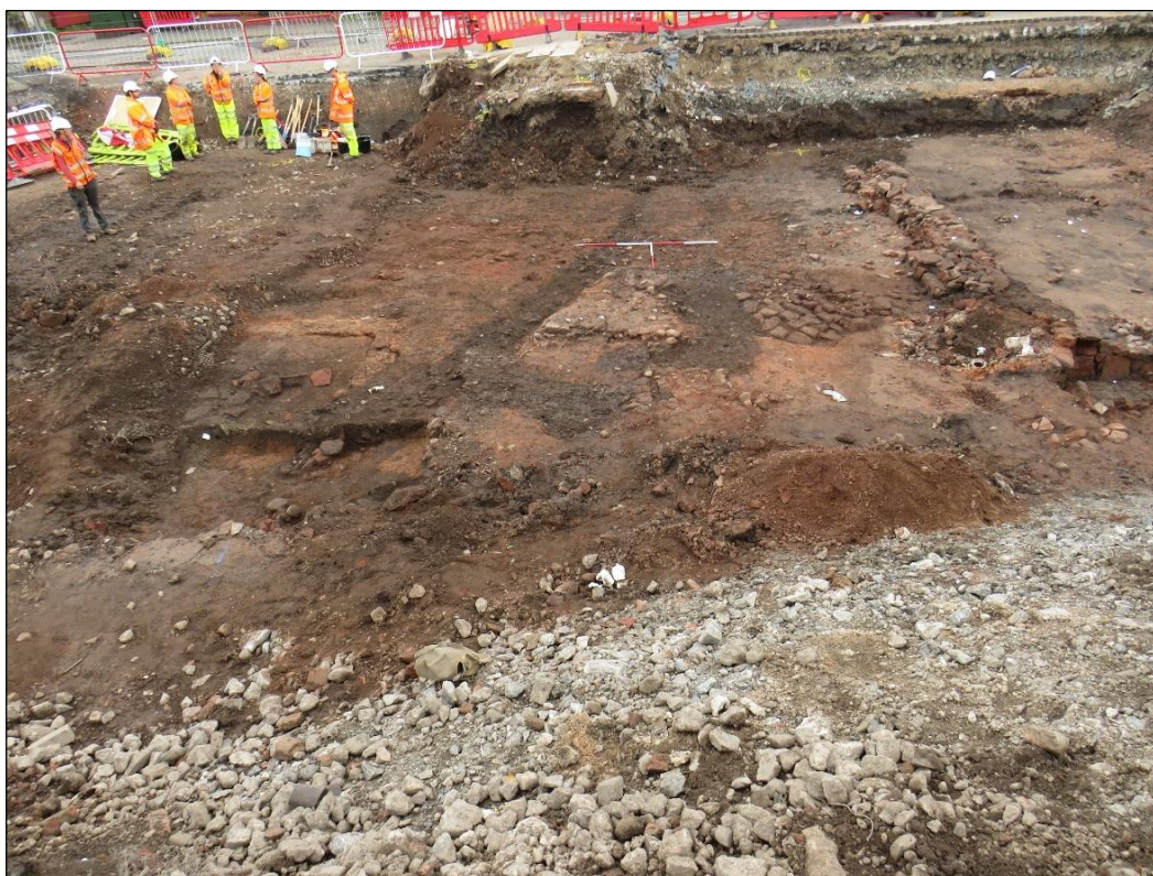
Plate 3: Period 2: excavation of the lower foundation pile mat for the new market and cinema, looking north, showing the north-east corner of a potentially early second-century phase of barrack 801 (left), as an L-shaped foundation ( 522 )
