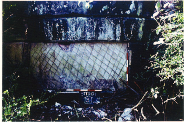
Plate 13: Blocked window/light well at SW corner of Orangery
