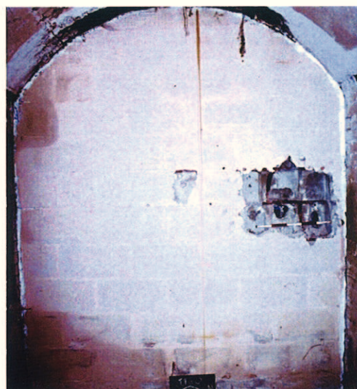
Plate 12: Blocked corridor at west end of Orangery
