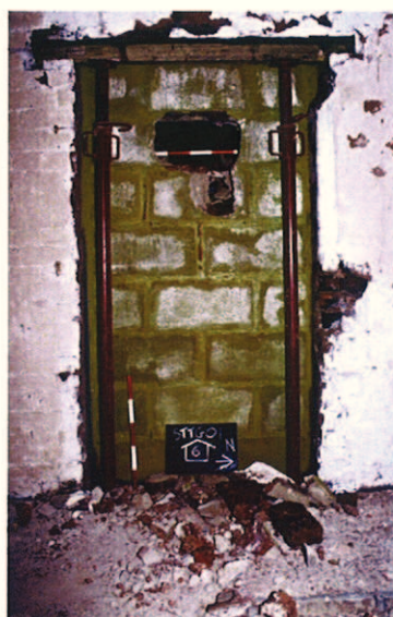
Plate 11: Smaller blocked entrance at west end of Orangery
