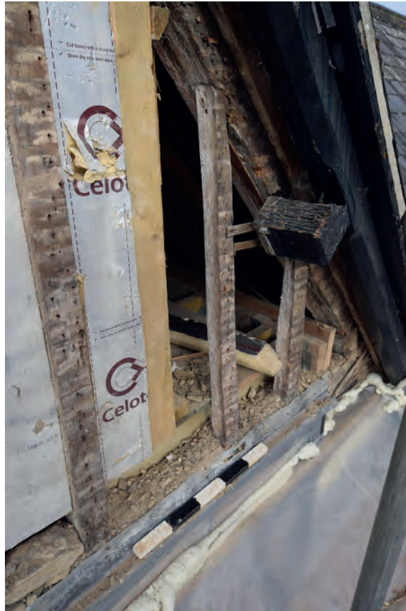
Plate 7: Fake purlin on the gable of Nos. 1-2
