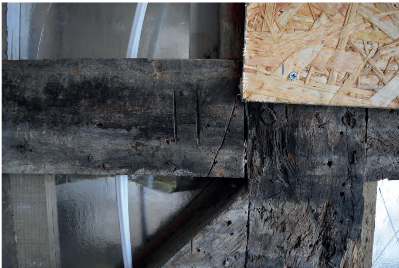
Plate 3: Carpenters' mark on the south elevation of Nos. 1-2 at first floor level
