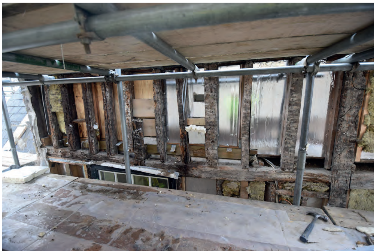
Plate 18: East elevation of Nos. 1-2 with truncated post above first floor window
