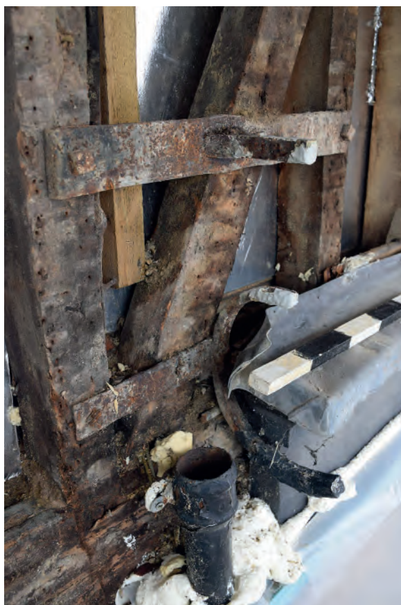
Plate 43: Truncated gas lamp bracket between the ground and first floors of No. 4
