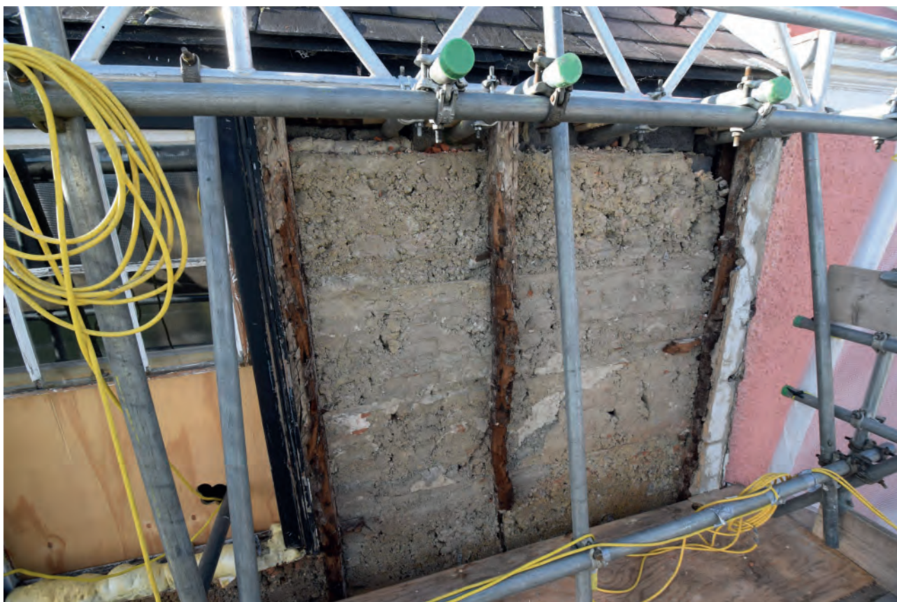
Plate 54: Imprints of lost rails of No. 7 on concrete
