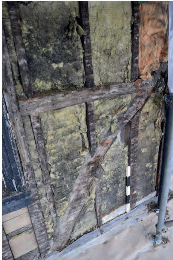
Plate 8: Northern brace on the east elevation of Nos. 1-2 at first floor level
