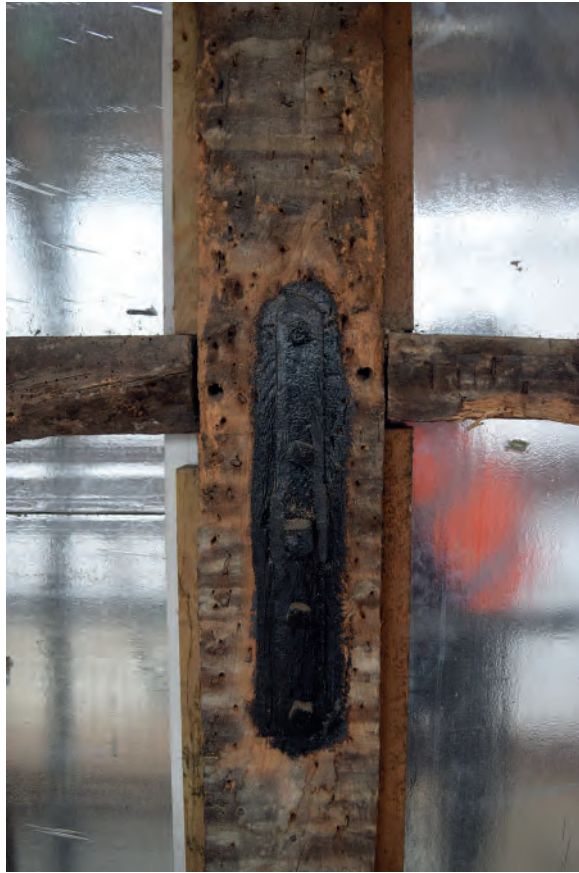
Plate 5: Strap and carpenters' mark on east elevation of Nos. 1-2 at first floor level
