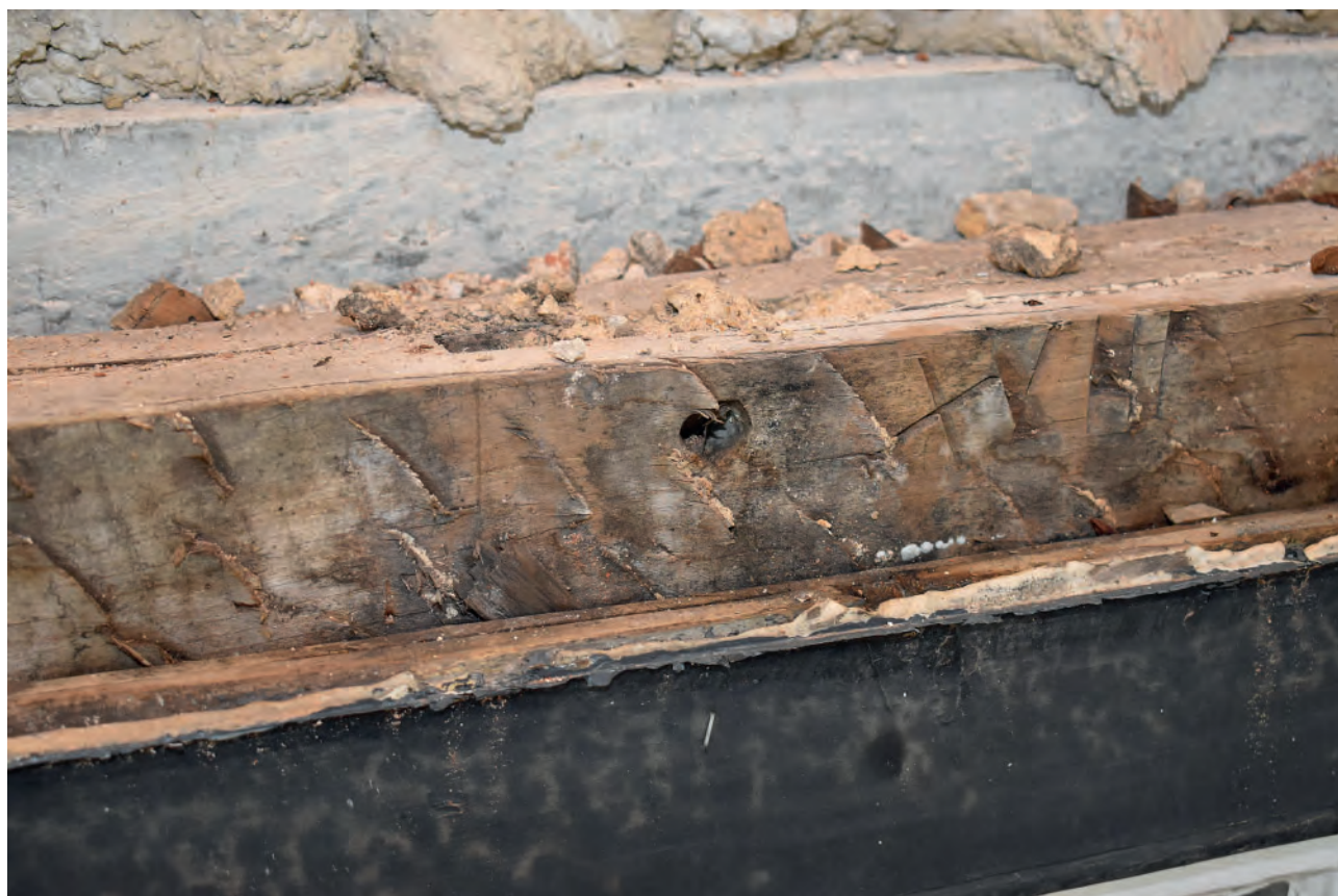
Plate 62: Peg hole, mortise and carpenters' mark above first floor north window of No. 7
