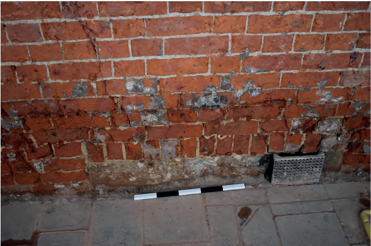
Plate 52: Block coal chute or cellar light on the northern side of Nos. 5-6
