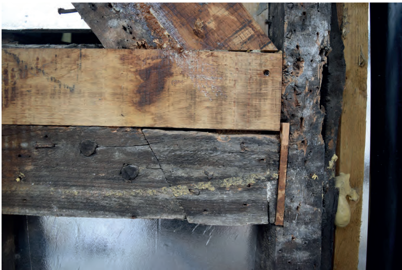
Plate 31: Scarf joint at northern end of rail on first floor of No. 3
