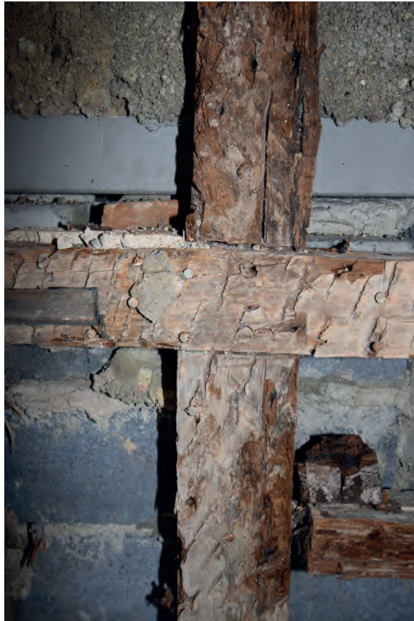
Plate 57: Scouring and nails on the framing of No. 7
