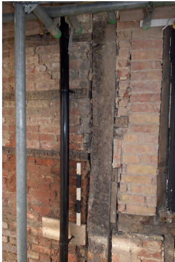
Plate 42: Rough brickwork between Nos. 3 and 4
