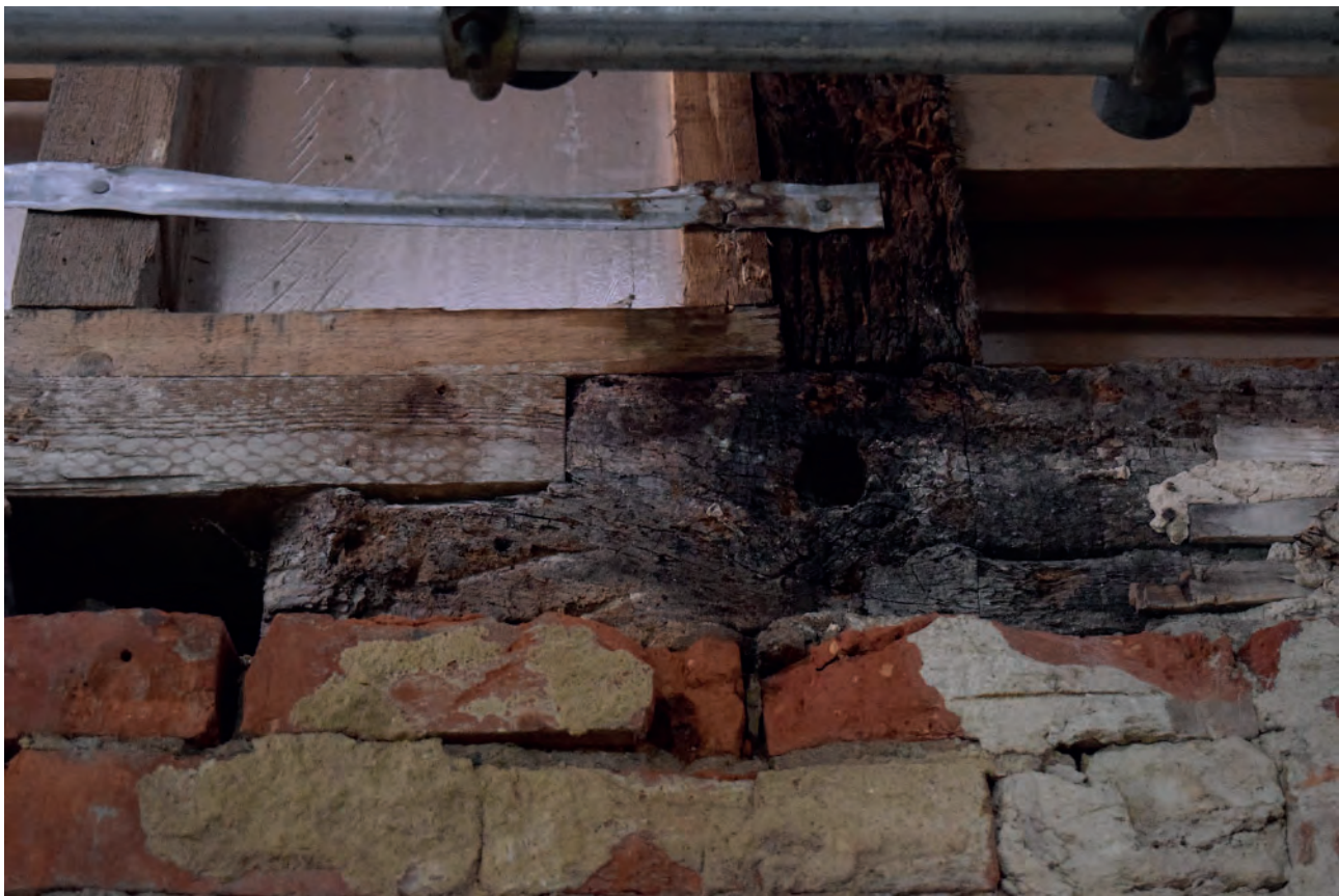
Plate 25: Peg hole and half lap joint above ground floor window of Nos. 1-2
