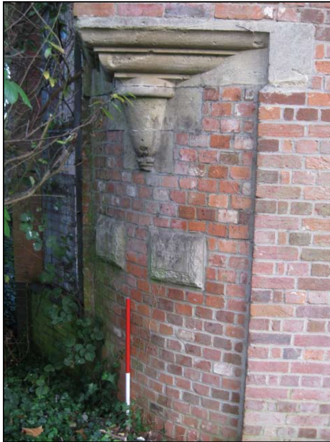
Plate 4: Corner feature on left side of south face of gable wall
