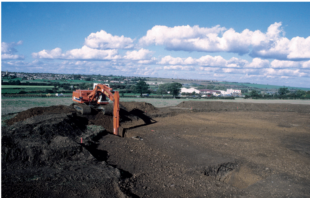
Plate 3.1 Machine excavating a section in the Iron Age site looking north-west across the Nene Valley
