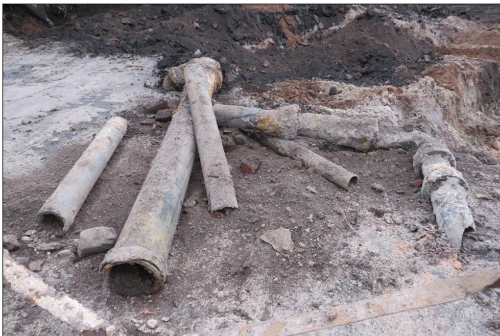
Plate 11: Example of metal piping found during excavations, most likely belonging to the flue system running west away from chimney base 206 (no scale)
