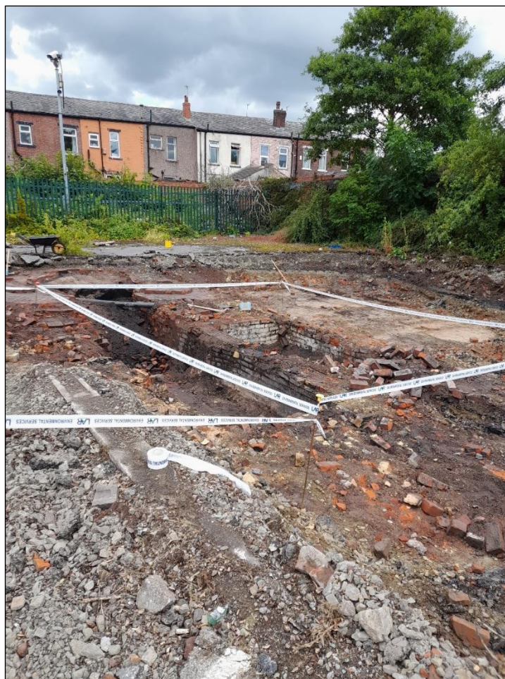
Plate 6: Areas of asbestos contamination in Trench 2
