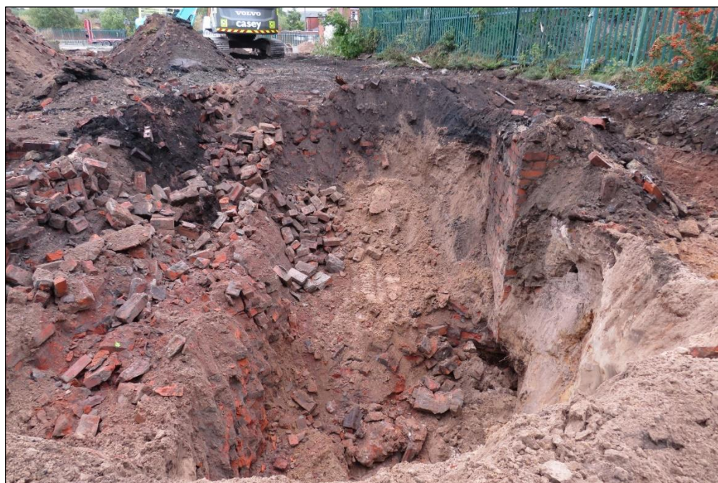
Plate 7: Excavated area following removal of chimney base 206, depth in excess of 3m (no scale)
