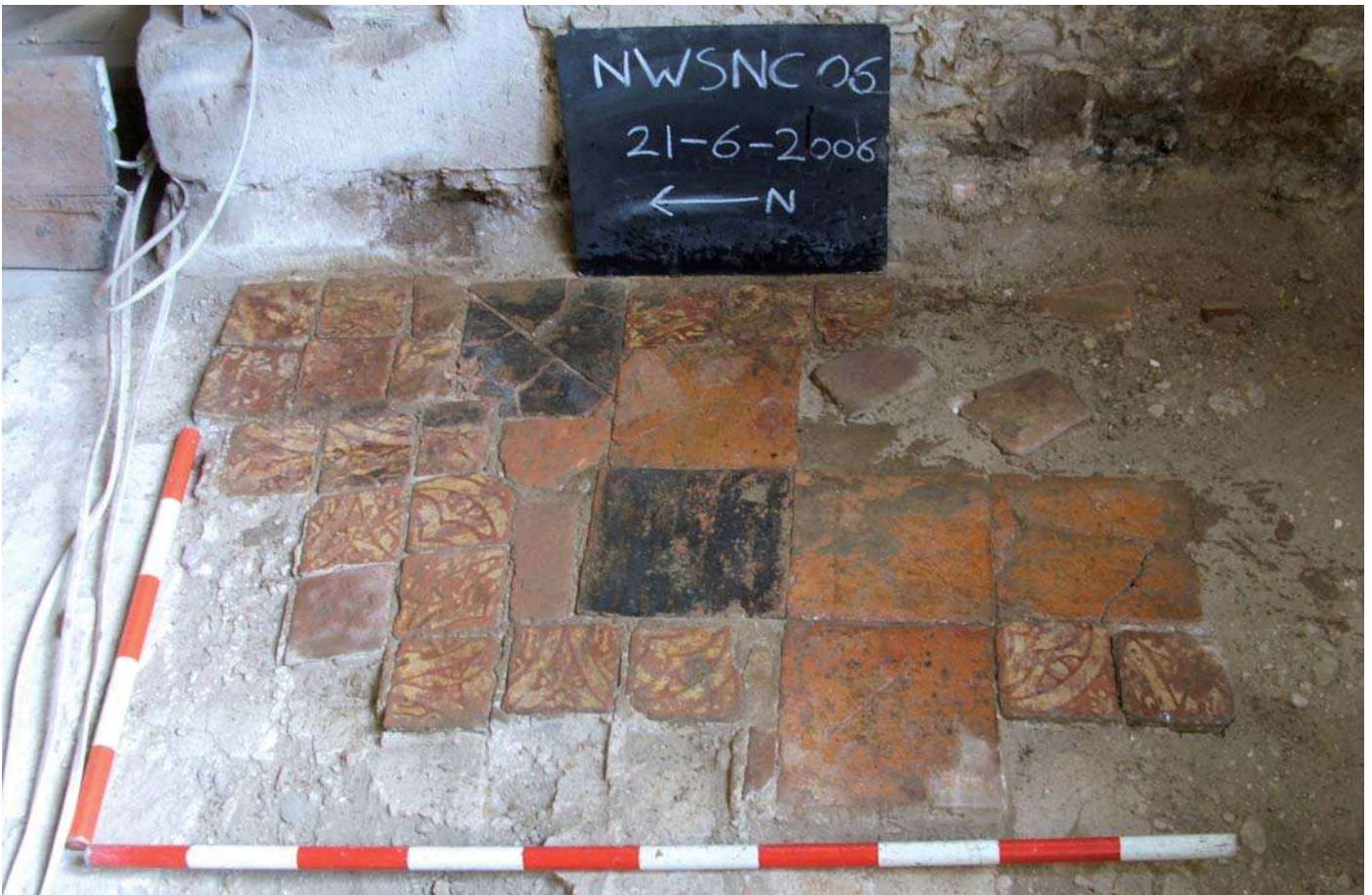
Plate 10: Remnant of tiled floor at east end of south side of nave (looking east, 1m and 0.5m scale)
