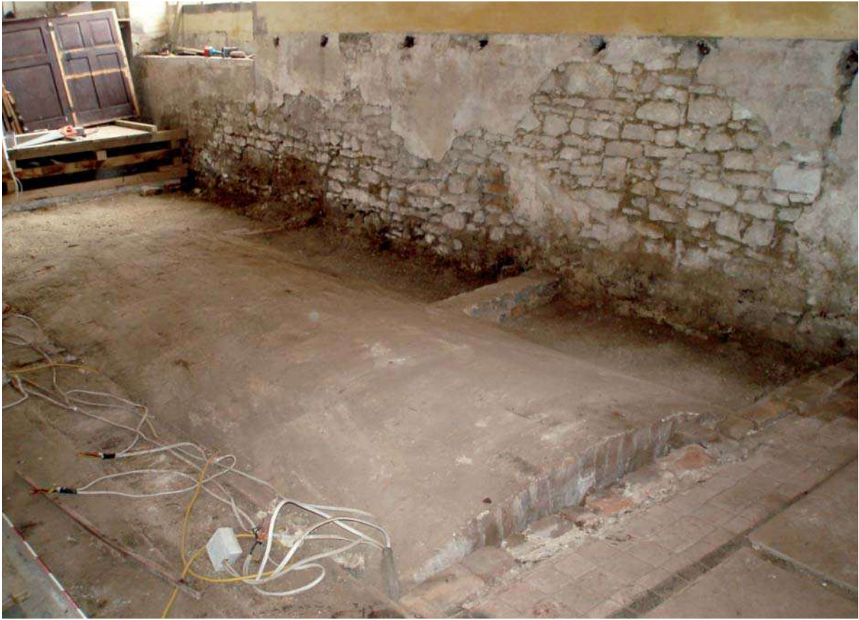
Plate 15: South wall of Nave after pews removed with burial vault to north (looking south-east)
