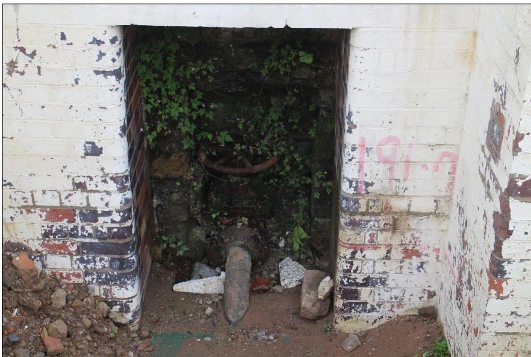
Plate 4: Opening in lower part of retaining wall for valve to reservoir, looking south
