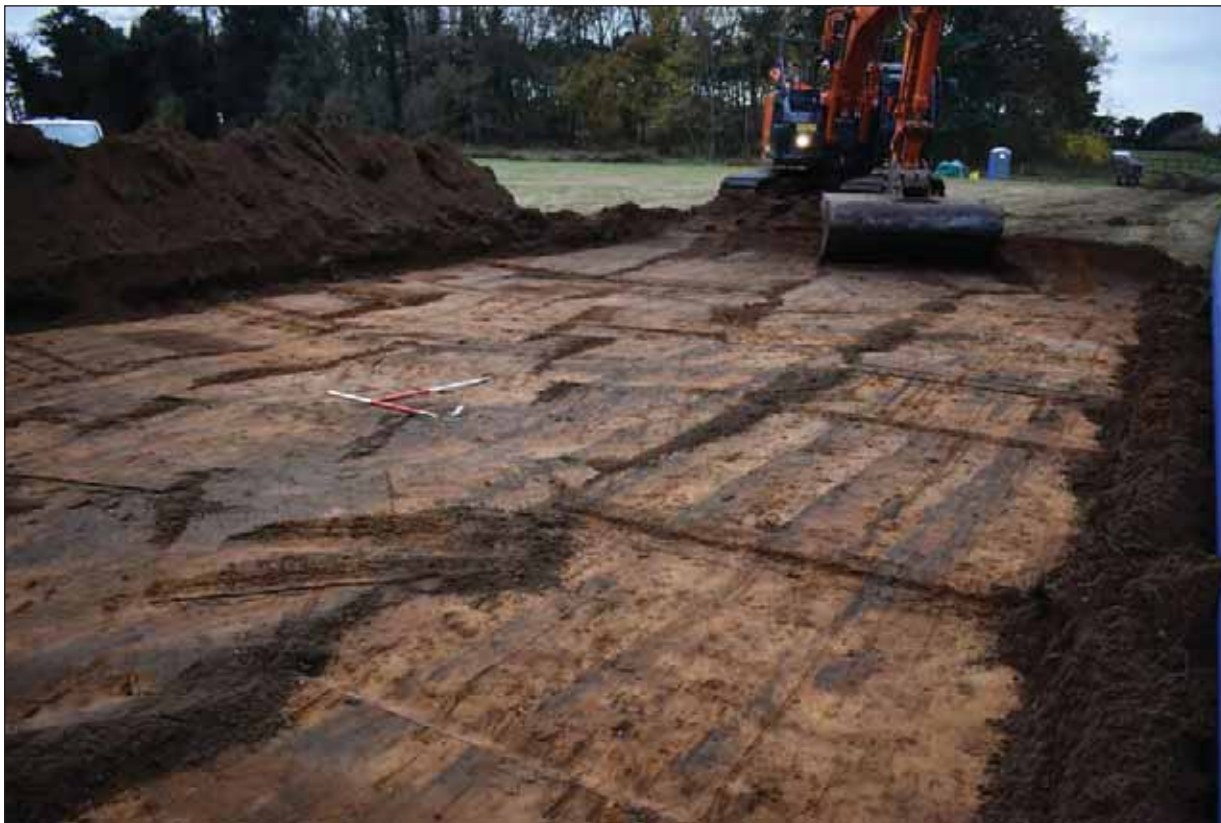
Plate 17: Area 7: General view of machine stripping of topsoil along the pipeline easement
