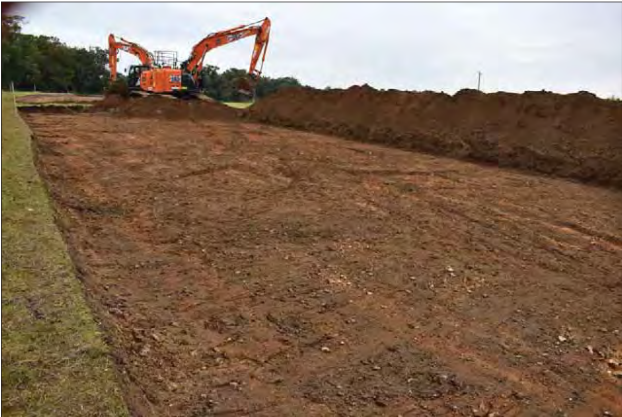
Plate 15: Area 2: General view of machine stripping of topsoil along the pipeline easement
