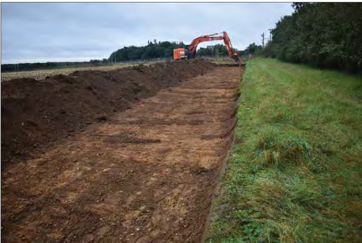
Plate 16: Area 3: General view of machine stripping of topsoil along the pipeline easement
