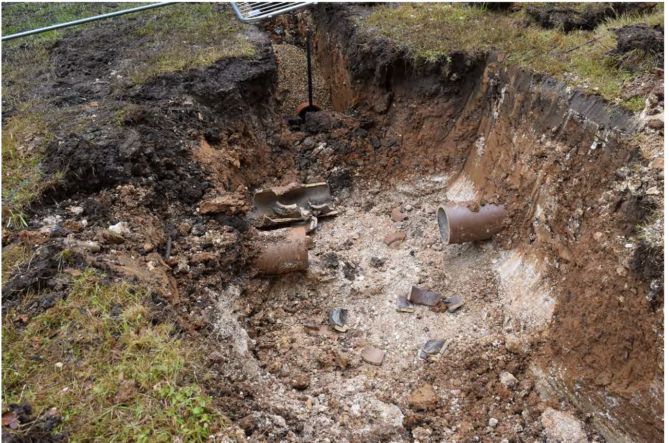
Plate J.14: Pipe exposed in excavations in Rushy Valley [J.104], looking west
