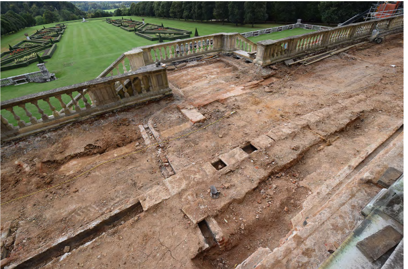
Plate F.27: Area of terrace immediately in front of mansion during works, looking south-west
