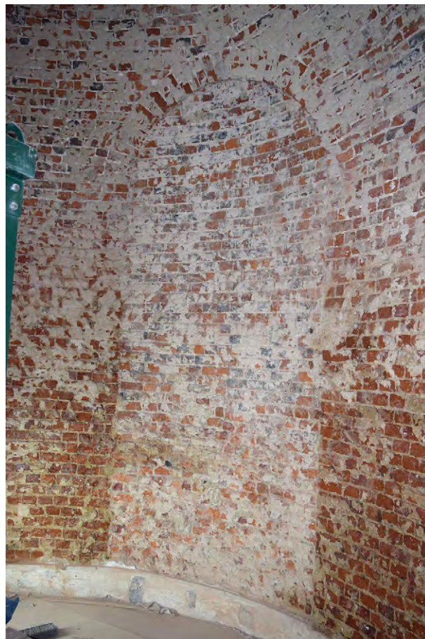
Plate D.14: Blocked archway [D.1.8] in east wall of Inner Sounding Chamber
