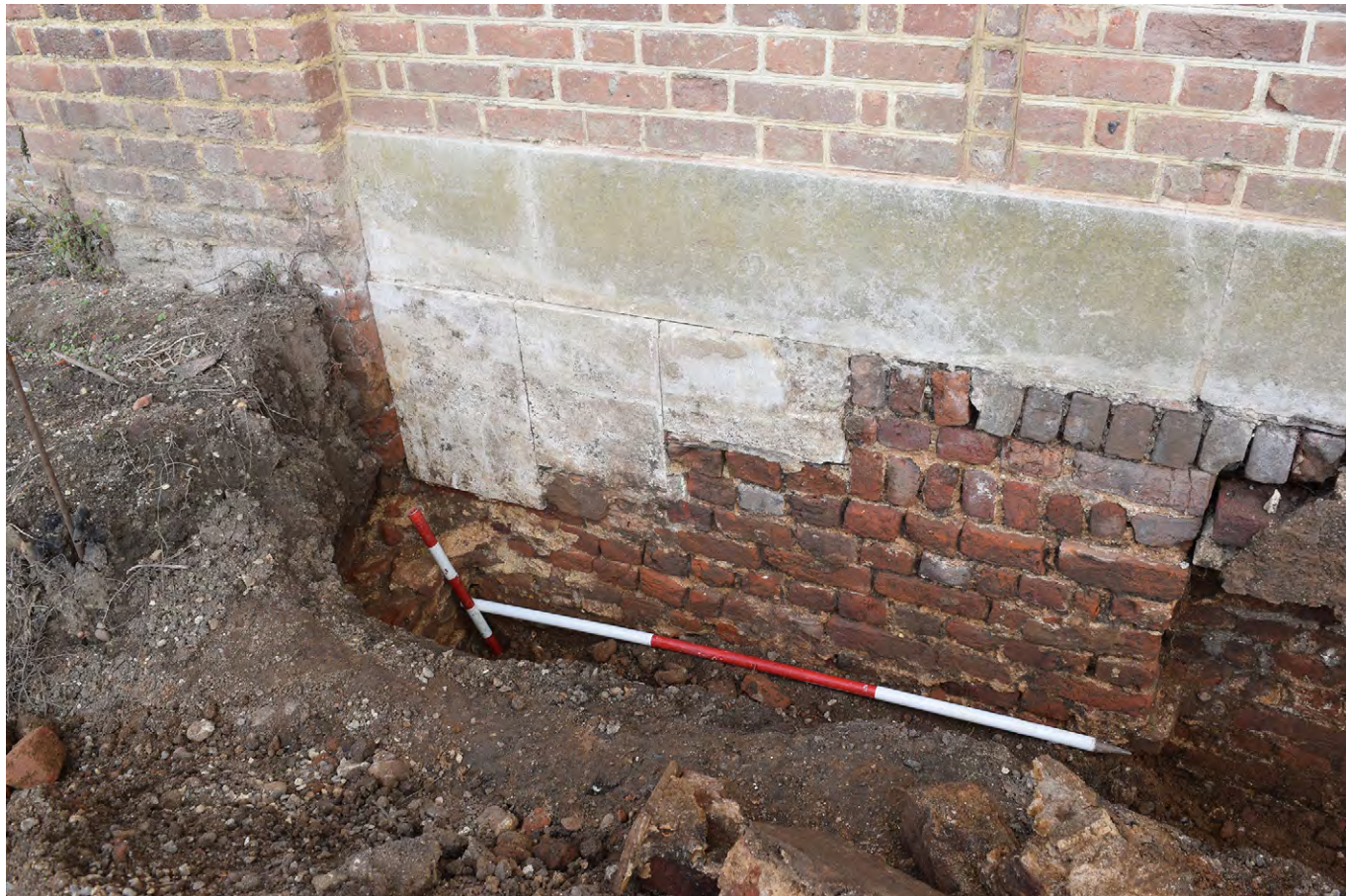
Plate C.47: Evidence of former steps in south face of East Fernery, looking north
