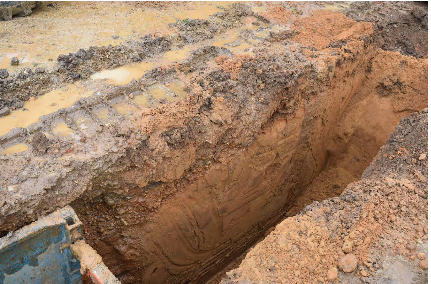
Plate G.4: Large area of pure sand in main trench [G.100] in front of East Fernery Water Tank, looking north-east
