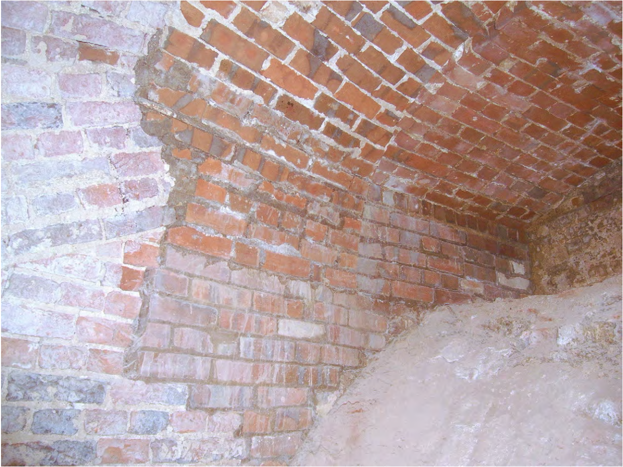
Plate D.11: Rebuilt brickwork towards top of eastern light well, looking south-east
