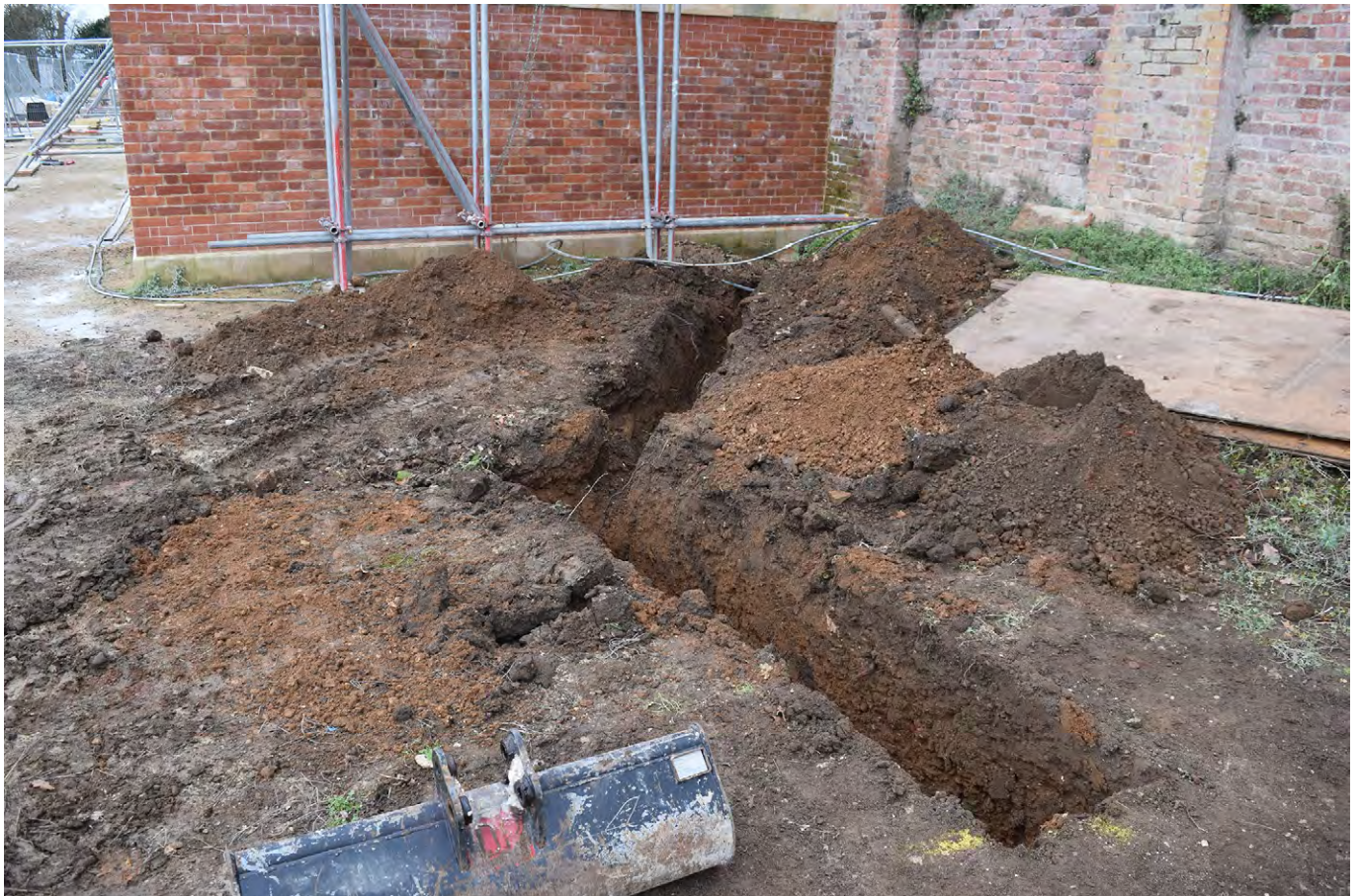
Plate G.21: Temporary soakaway trenches dug to east of staircase [G.115], looking north-west
