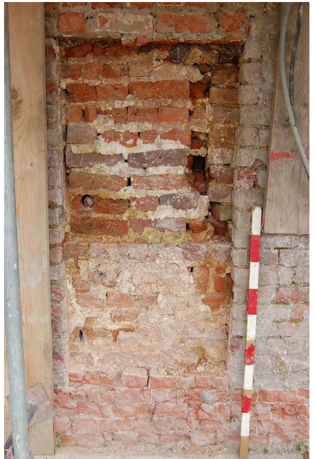
Plate A.65: Hidden brickwork exposed by removal of central pilaster to east side of stairs
