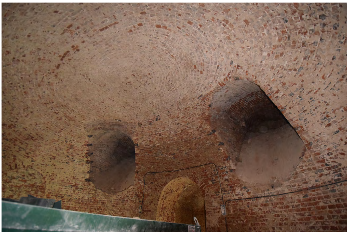
Plate D.10: The two former light wells in Inner Sounding Chamber, looking south-east
