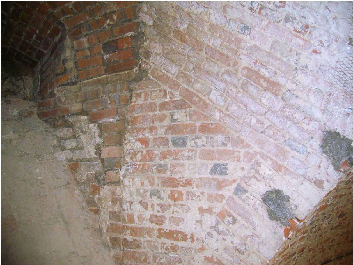
Plate D.12: Rebuilt brickwork towards top of eastern light well, looking west
