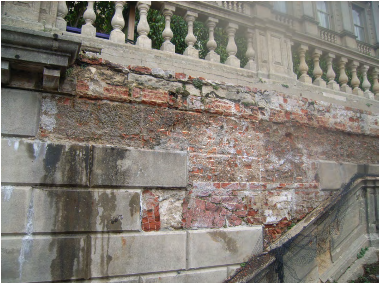
Plate B.12: Area on west side of stairs where rustication removed
