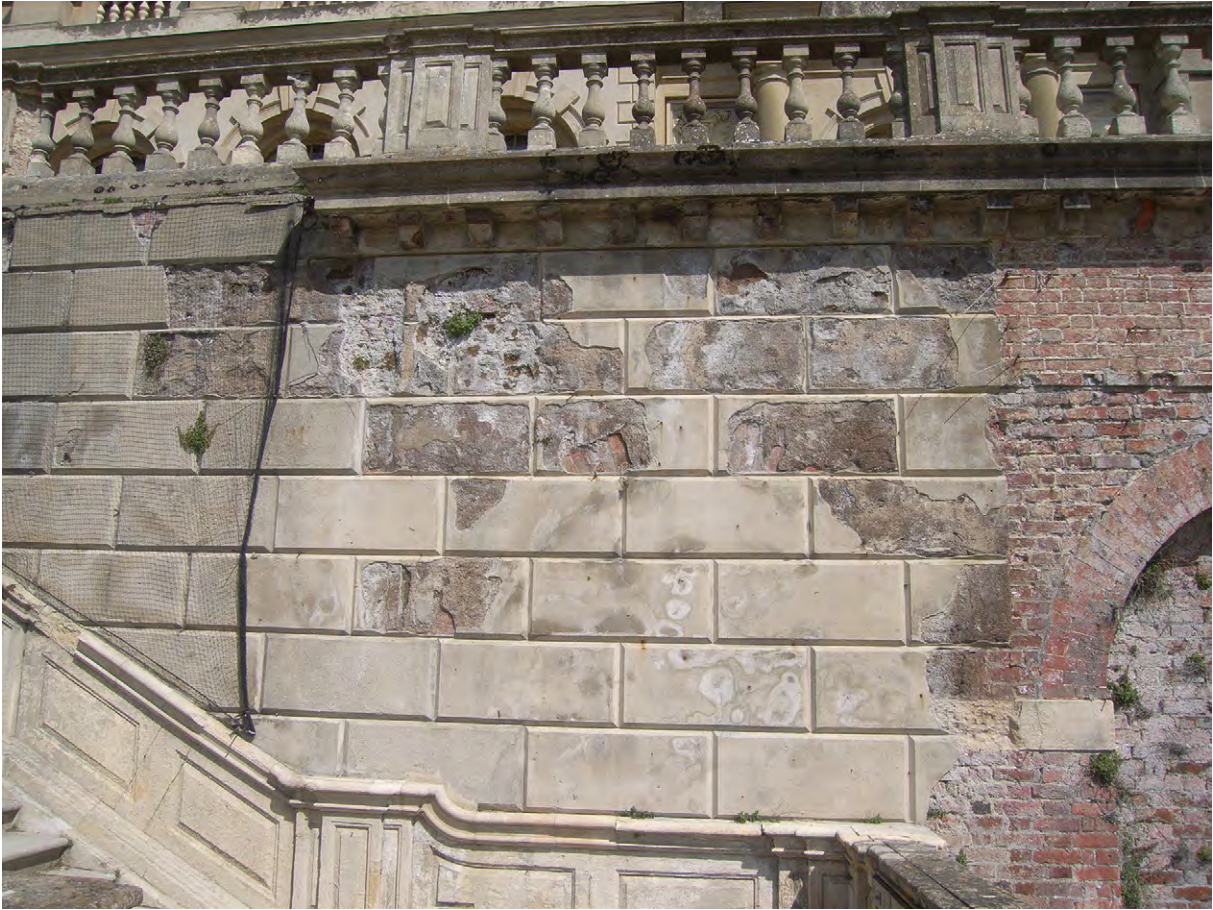
Plate B.7: Rustication behind east side of stairs
