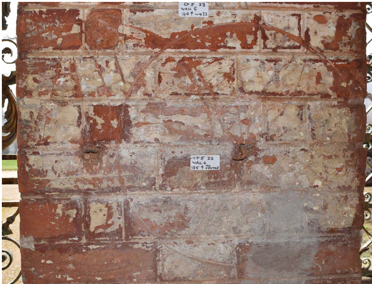
Plate C.30: Circular marks on south wall inside East Fernery [C.2.1], looking south to east of doorway
