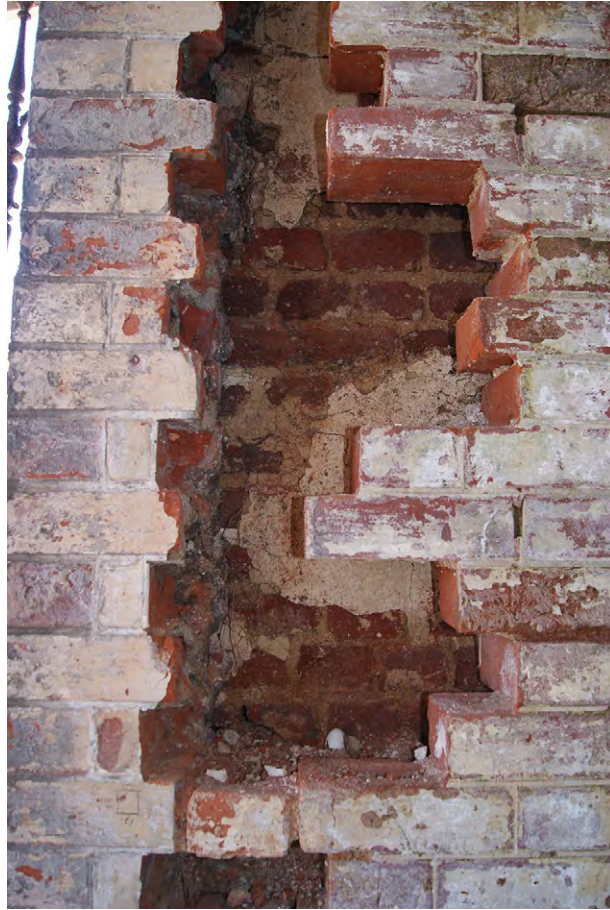
Plate C.18: Area of removed bricks with older plastered face behind west wall of West Fernery
