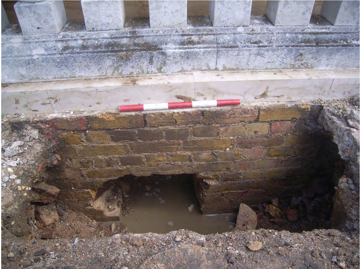
Plate I.3: Brickwork beneath balustrade to north of West Lawn, in trench [I.102], looking north
