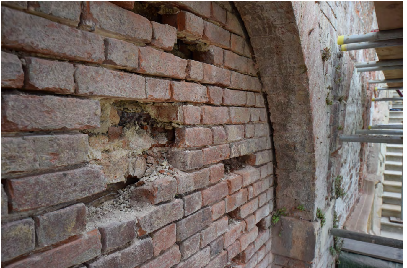
Plate B.20: Isolated bricks removed from blind arcade (Arch 9)
