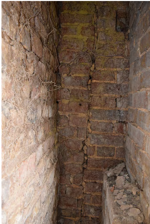
Plate E.2: Structural cracks in void between blind arcade skin and West Barrel Vaulted Chamber, looking west
