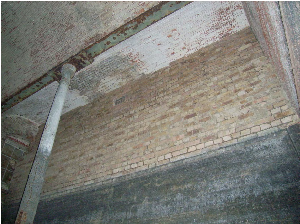
Plate C.41: East Fernery Water Tank (note brick infill in vault [C.4.3], looking north-east
