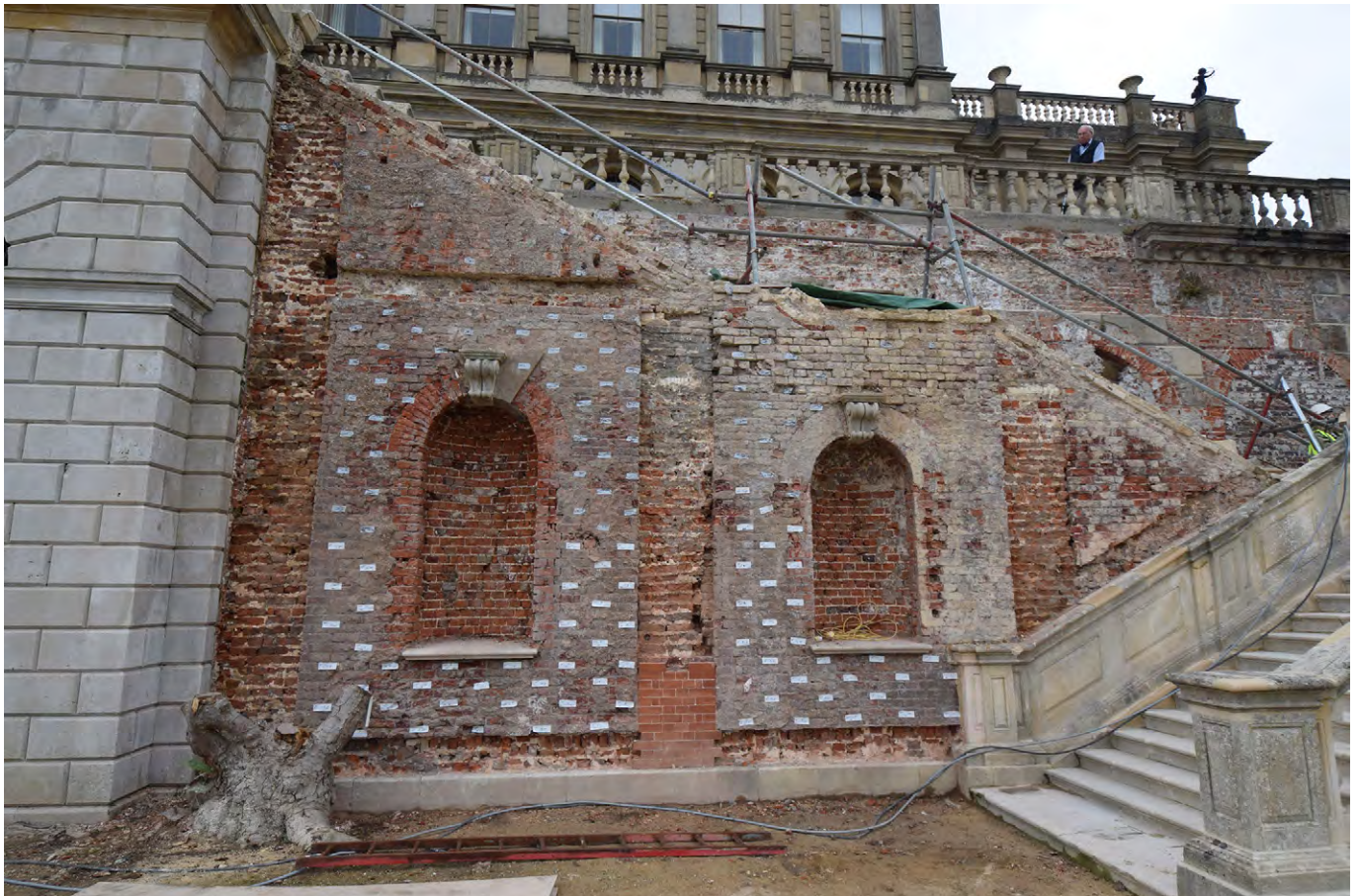
Plate A.42: East side of stairs after removal of render and pilasters
