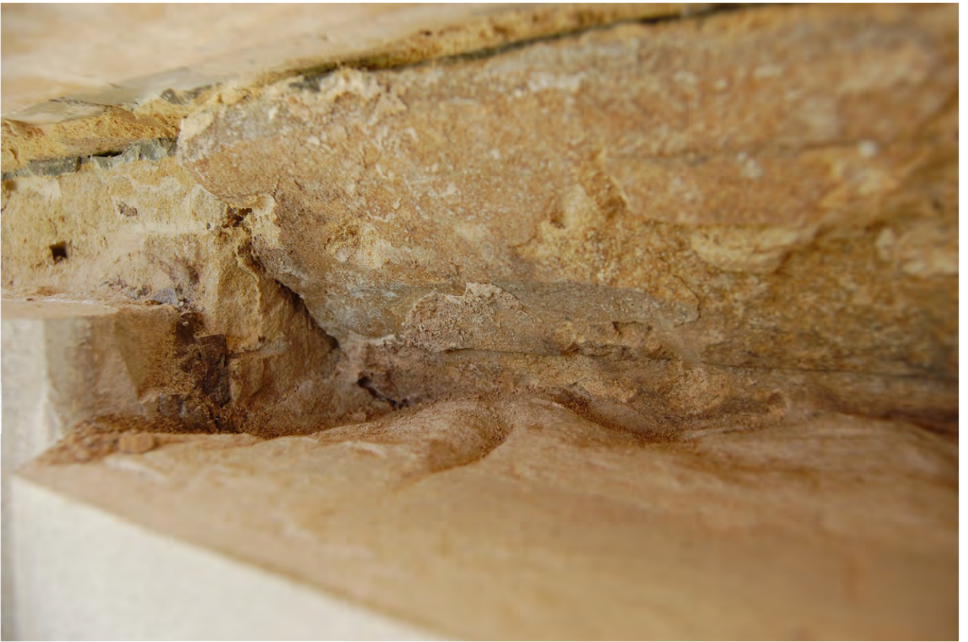
Plate A.63: Detail of exposed fragment of cornice [A.5.1]
