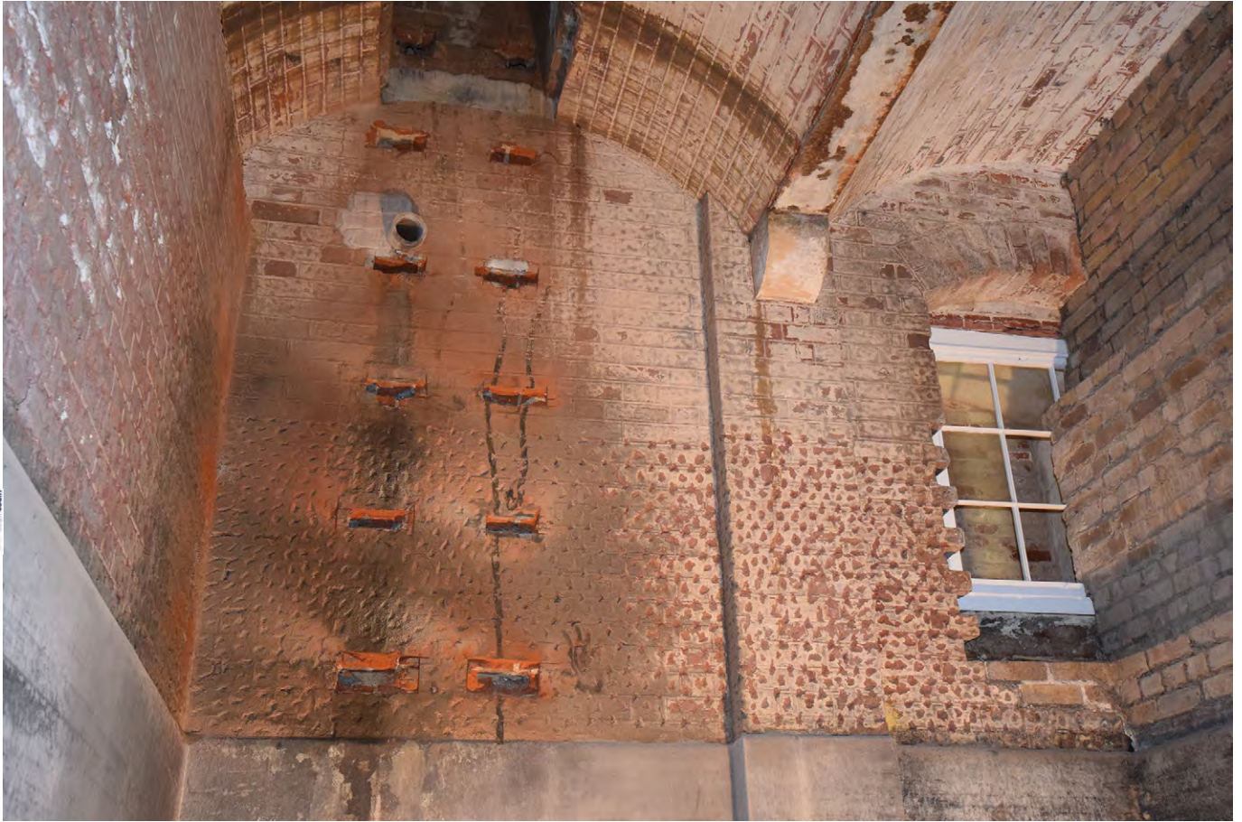
Plate C.40: North wall in East Fernery Water Tank
