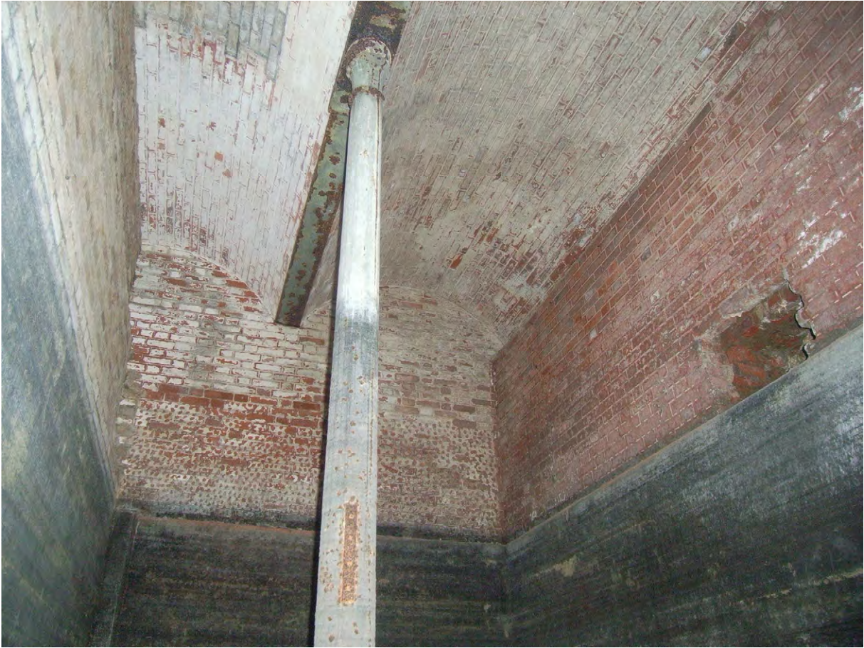
Plate C.36: West Fernery Water Tank (looking north)
