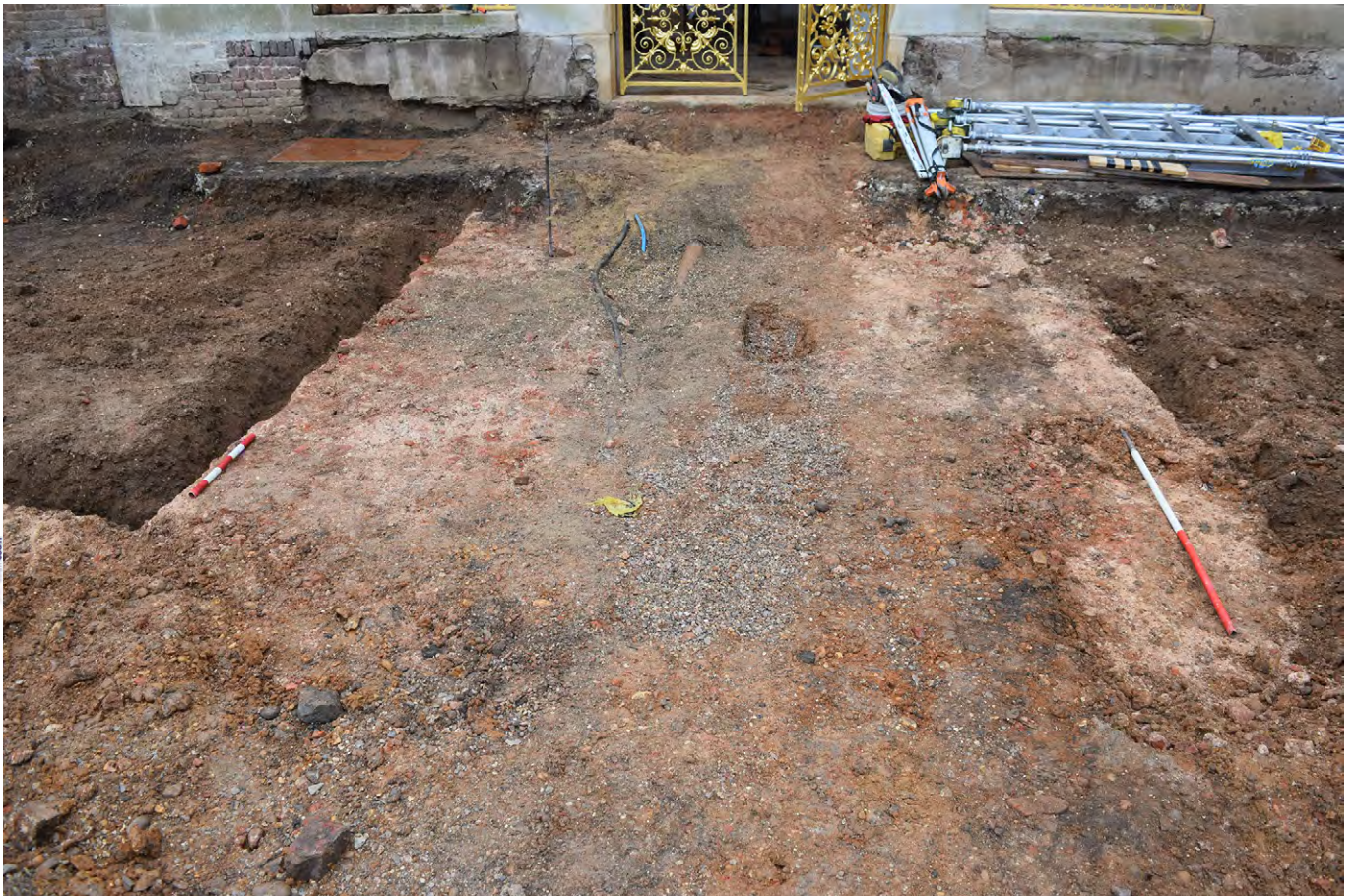
Plate G.24: Trace of brick base exposed in front of East Fernery [G.119.1], looking north
