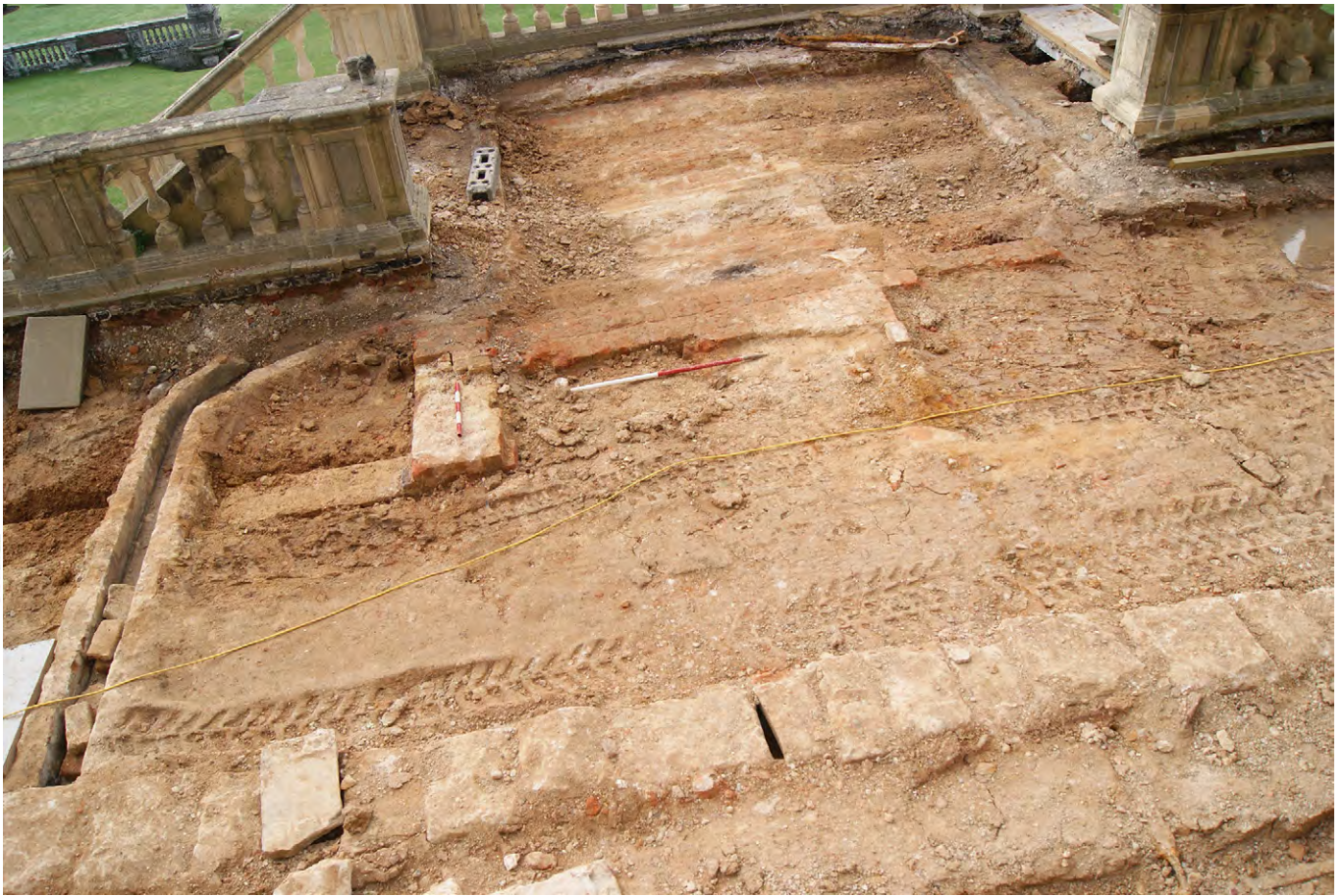
Plate F.28: Area of terrace immediately in front of mansion during works, looking south
