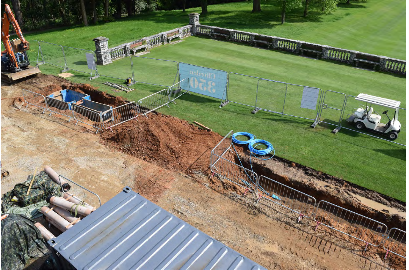
Plate G.7: General view from above to main trench [G.100], looking south
