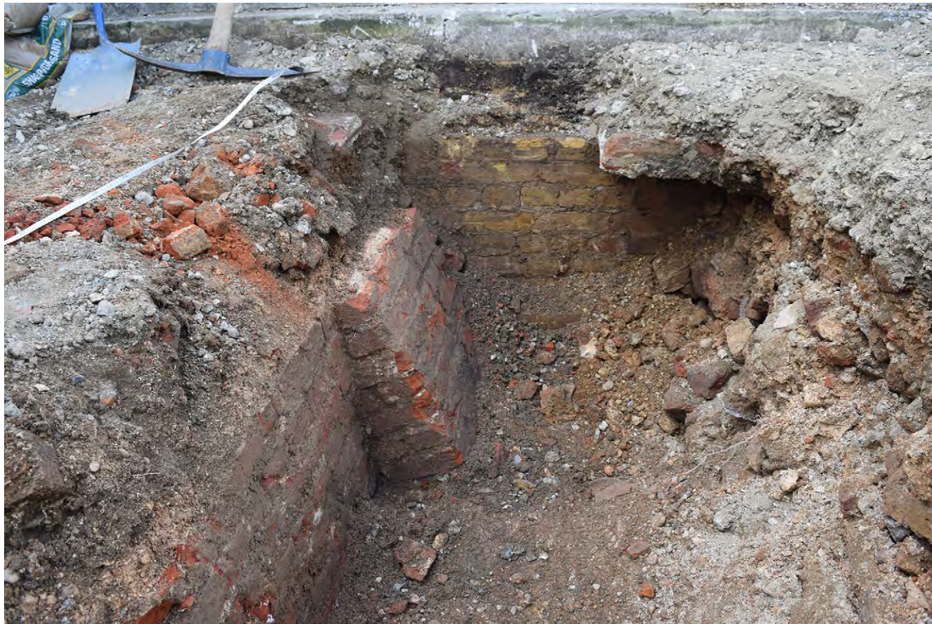
Plate F.11: Western end of former north wall of terrace. Buttress [F.1.9] exposed and later yellow brick-work forming retaining wall between terrace and pavilion, looking west
