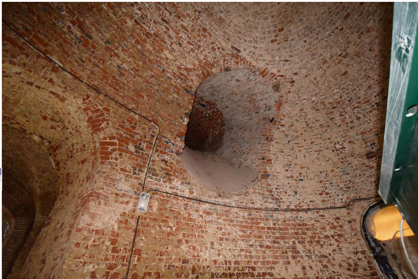
Plate D.9: Former light well on western side of Inner Sounding Chamber, looking south-west
