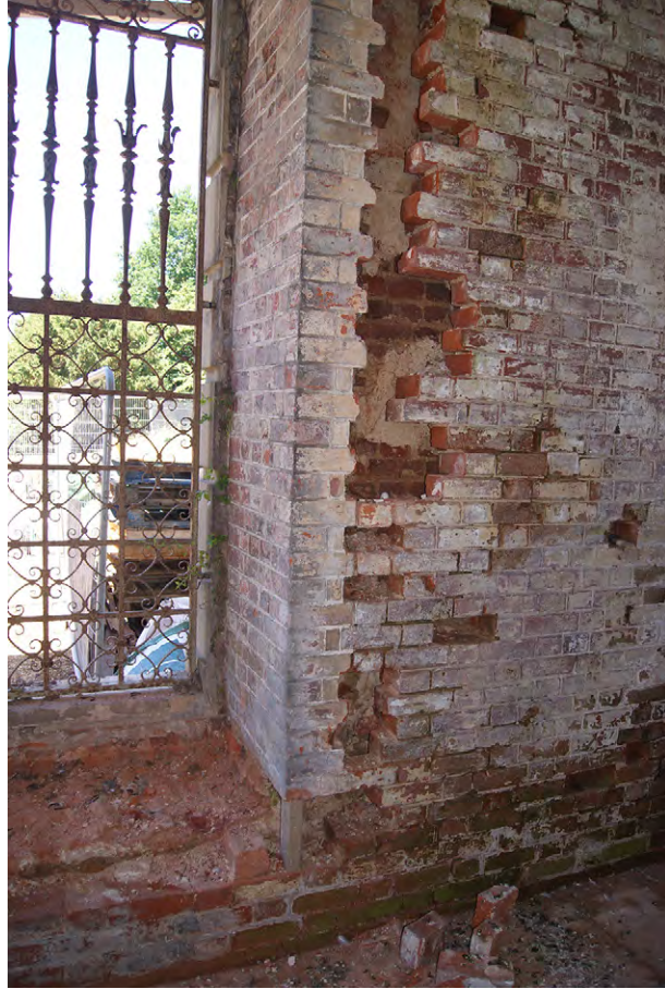
Plate C.16: Bricks removed from internal face of west wall in West Fernery, looking west
