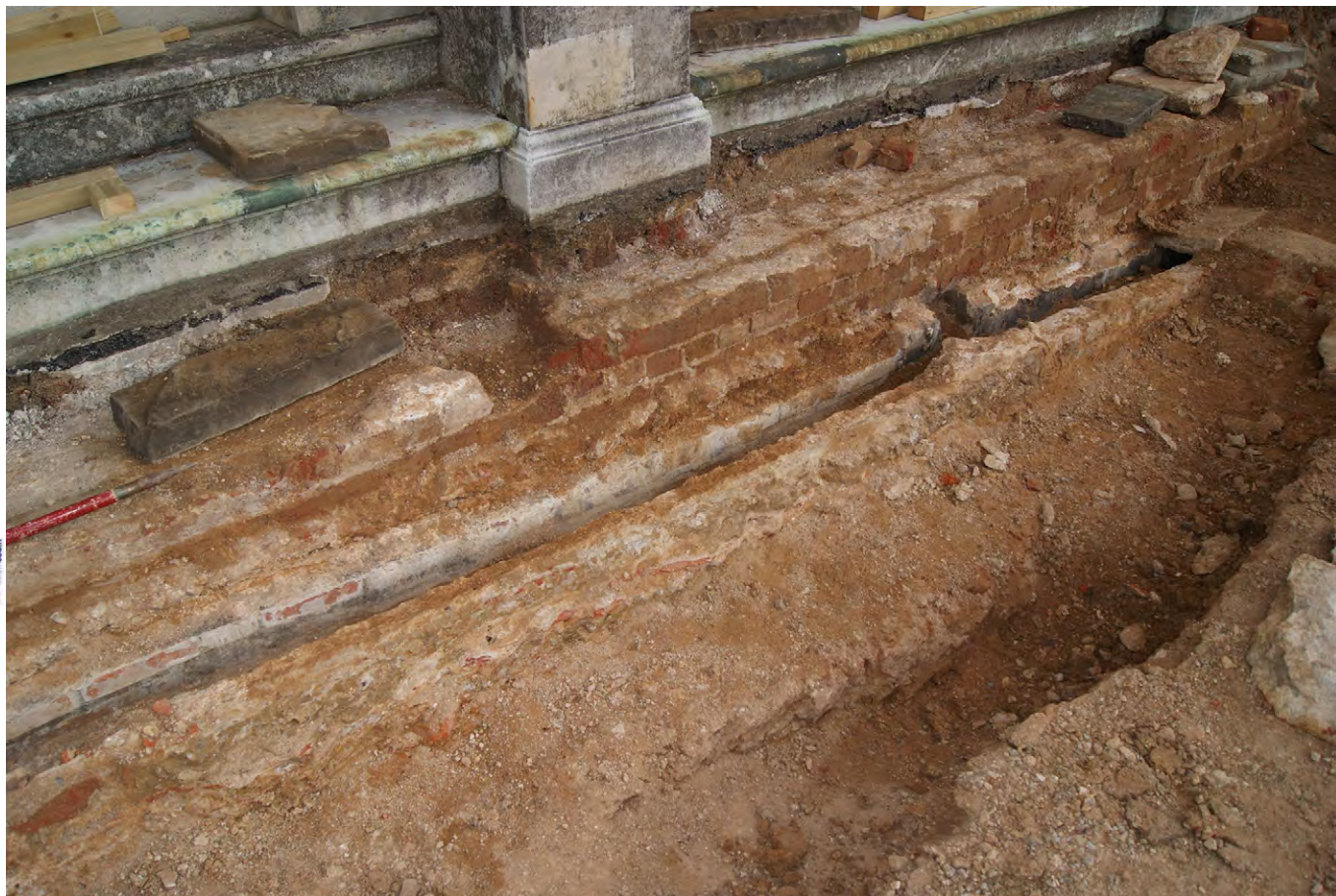
Plate F.52: Drains in front of mansion after removal of brick capping, looking north-east
