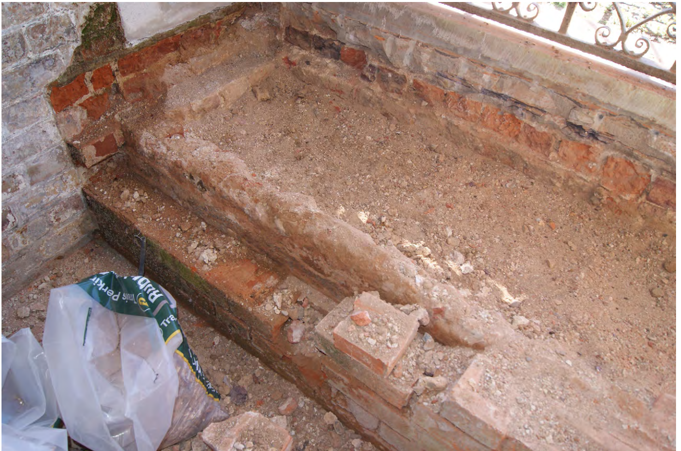
Plate C.19: Exposed base of wall beneath window in West Fernery, looking south
