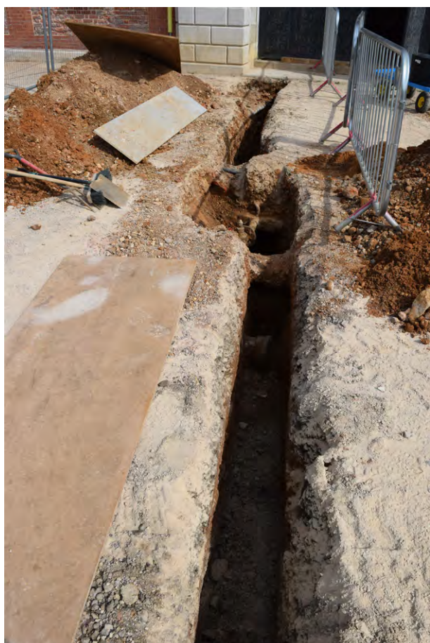
Plate G.57: Trench in front of portico with various service pipes and vavles [G.122]
