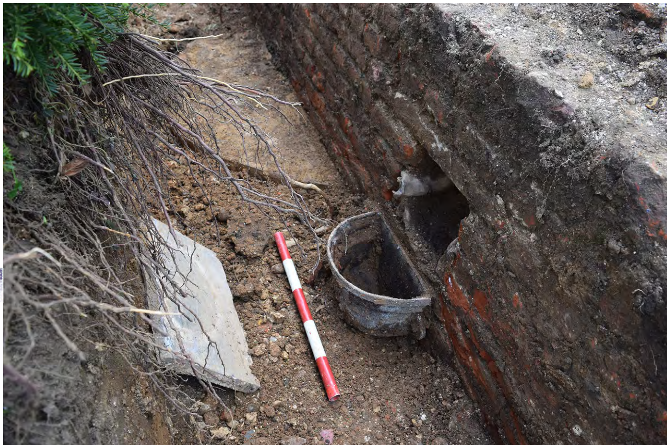
Plate F.12: Drainage hopper [F.1.11] in former north wall of terrace, looking south-east
