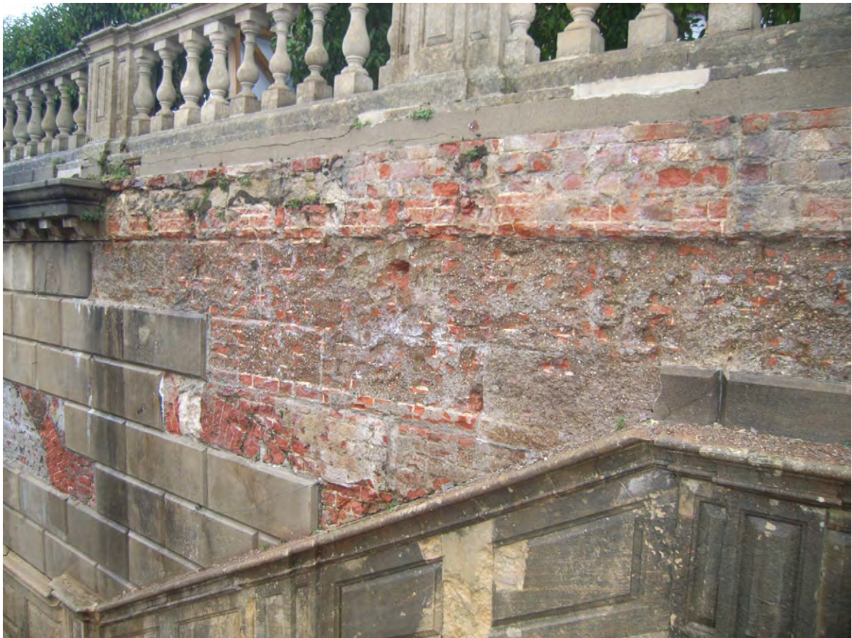
Plate B.13: Areas on west side where rustication removed (note B.2.3, B.2.1)
