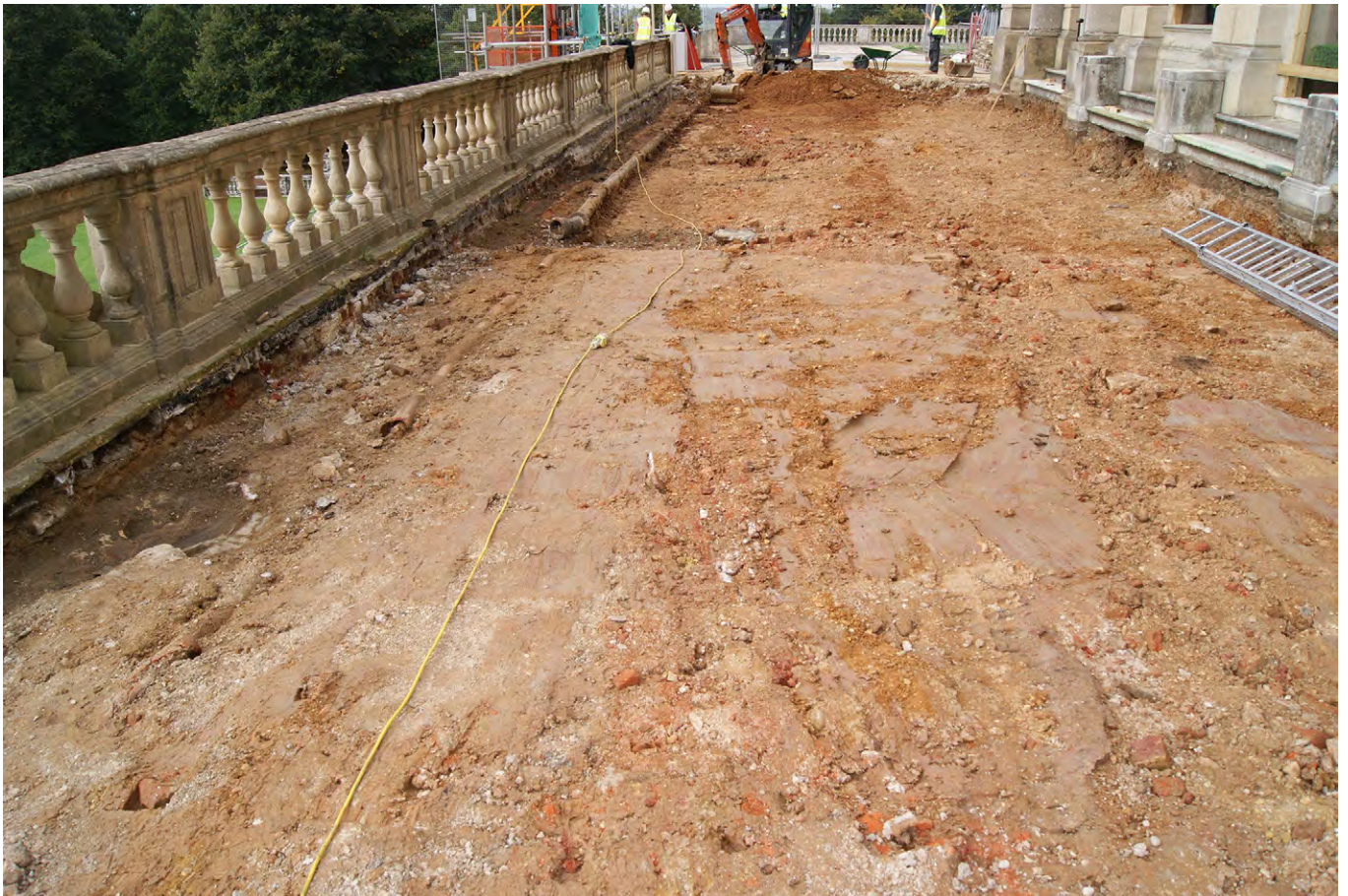
Plate F.16: Central part of terrace looking west after removal of paving and upper loose fill. (note clay pudding)
