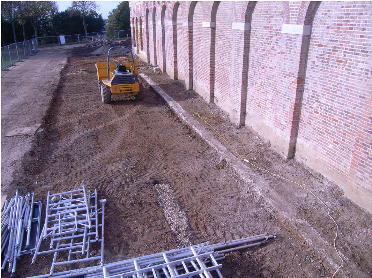
Plate G.39: West side of Blind Arcade with exposed limecrete edging in front [G. 119.3], looking west
