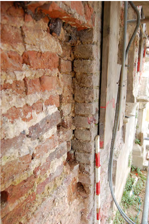
Plate A.64: Detail after removal of central pilaster to east side of staircase
