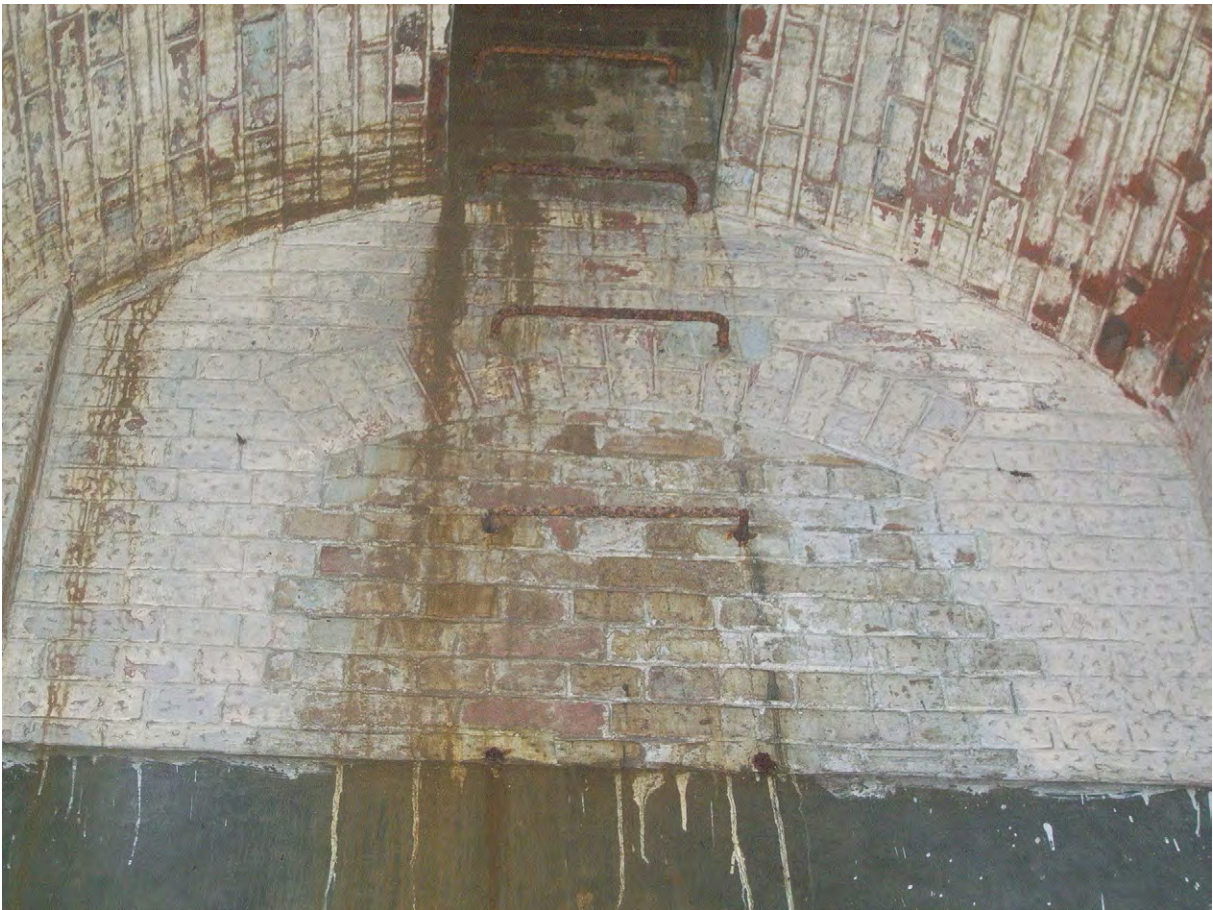
Plate C.37: Ladder and blocked arch in north wall of West Fernery Water Tank, looking north
