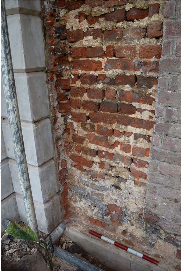
Plate A.66: Brick exposed by removal of plaster immediately east of portico
