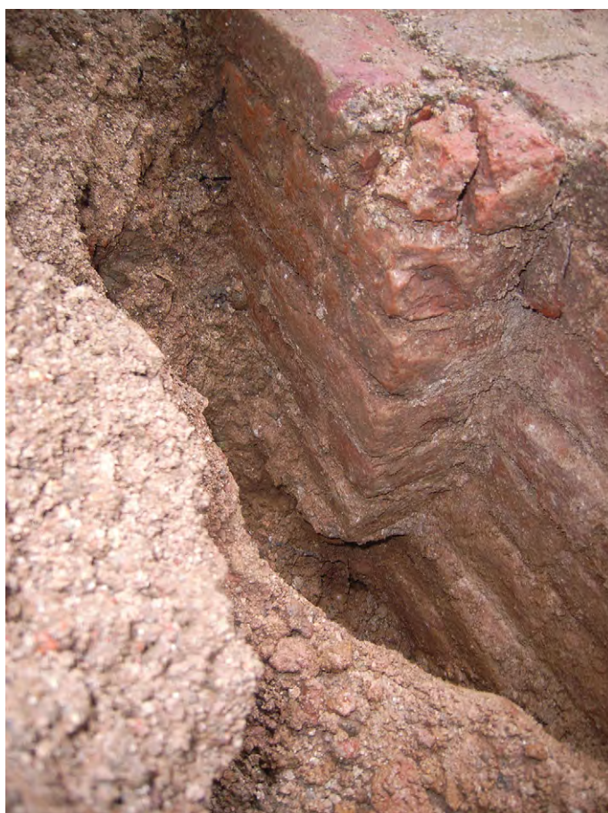
Plate G.19: Apparent pier to south face of Pit G.105, looking north-west
