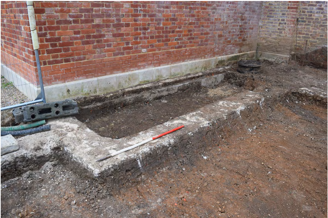
Plate G.29: Limecrete edging to east side of staircase [G.119.4], looking north-west
