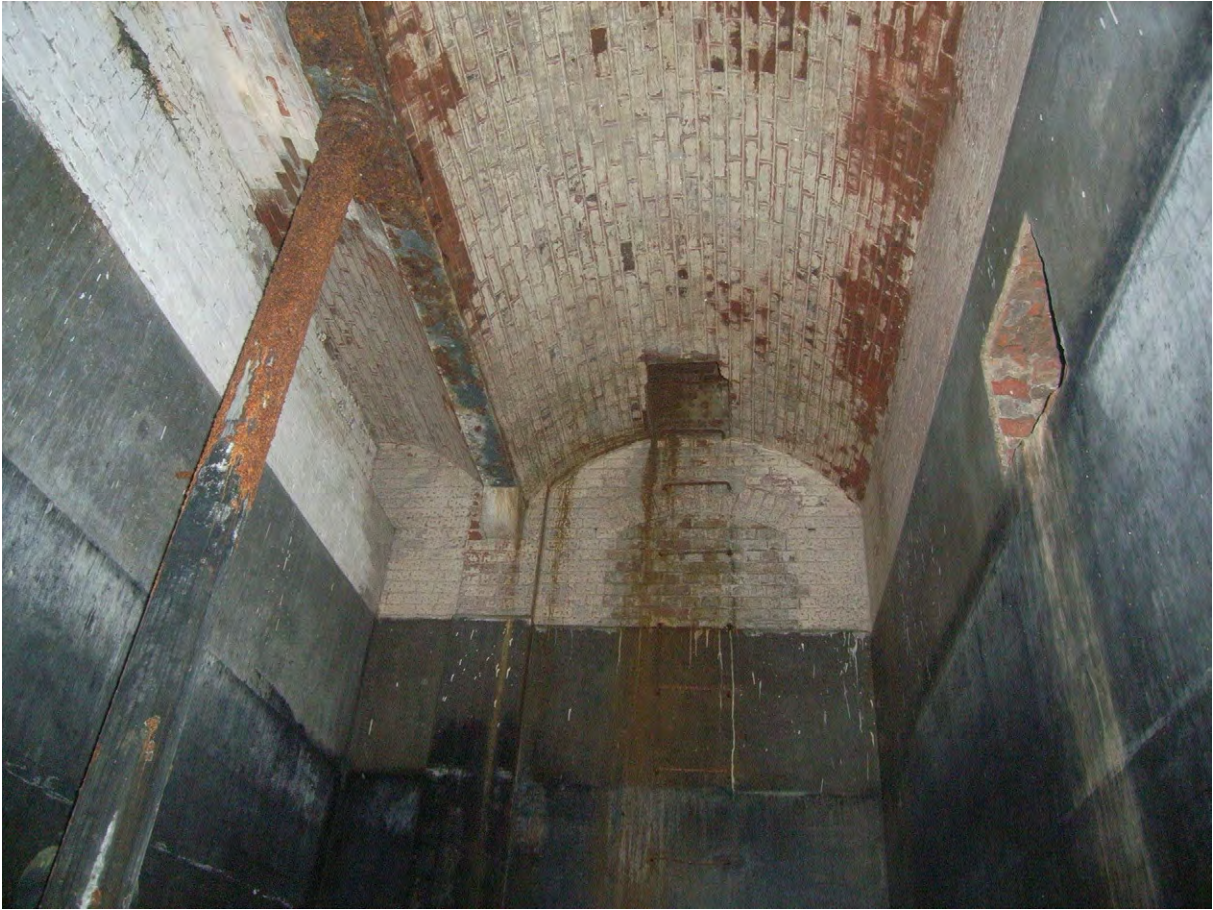
Plate C.38: West Fernery Water Tank (looking north)
