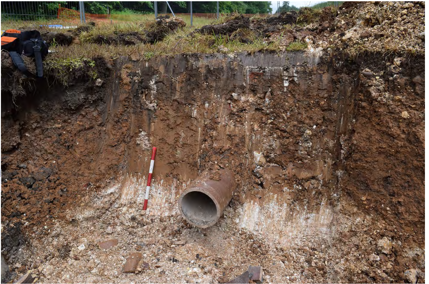
Plate J.15: Pipe exposed in excavations in Rushy Valley [J.104], looking north
