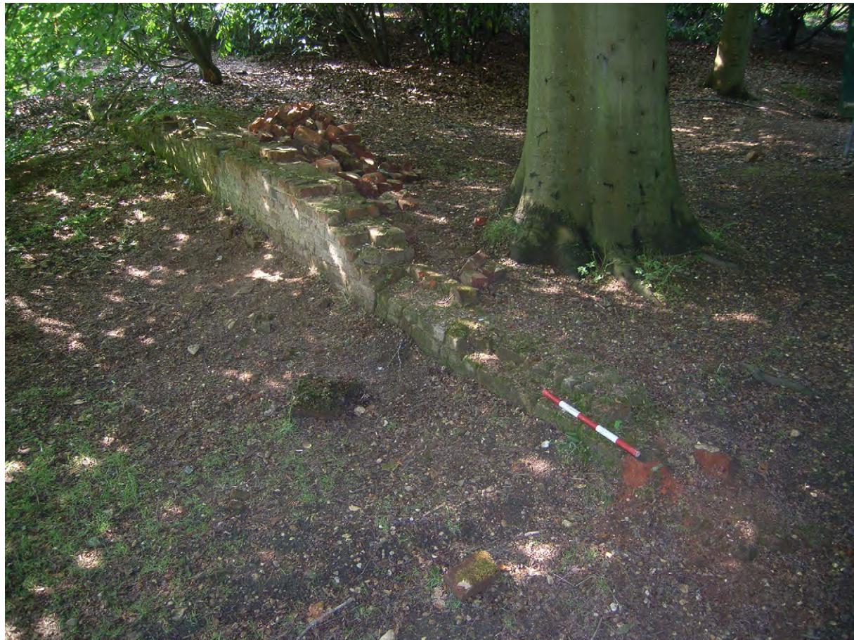
Plate J.9: Low retaining wall to east of terrace [J.1.1], looking north-west
