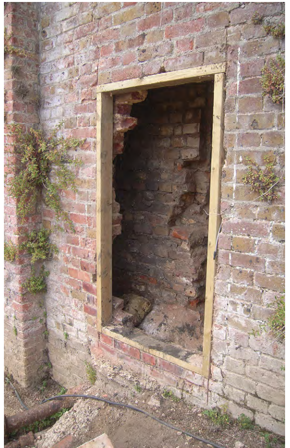
Plate E.9: Entrance formed in blind arcade to East Barrel Vaulted Chamber
