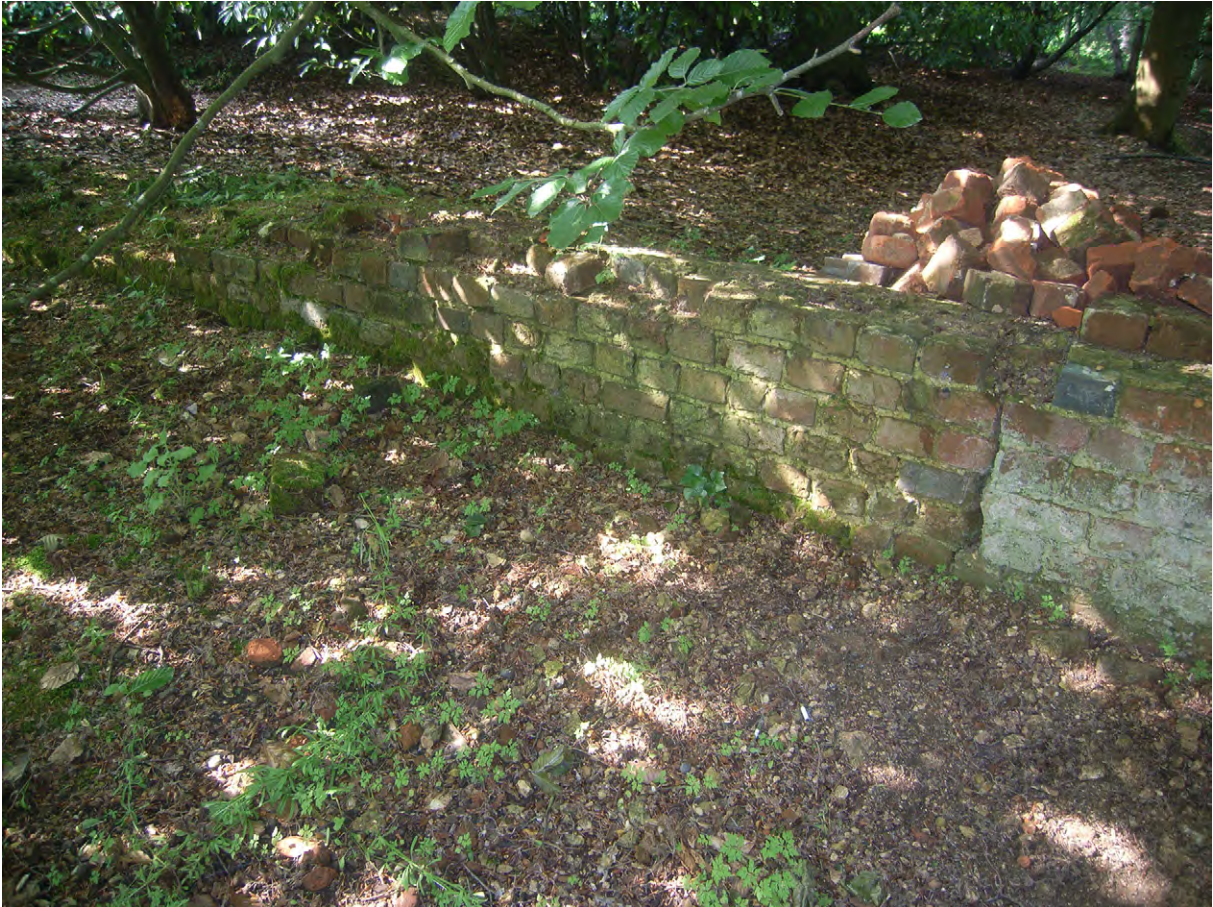
Plate J.10: Low retaining wall to east of terrace [J.1.1], looking north
