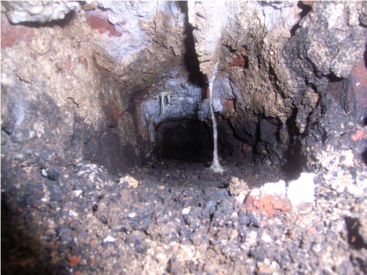
Plate C.45: E-W drainage duct exposed in excavations in East Fernery Water Tank [C.4.2], looking west
