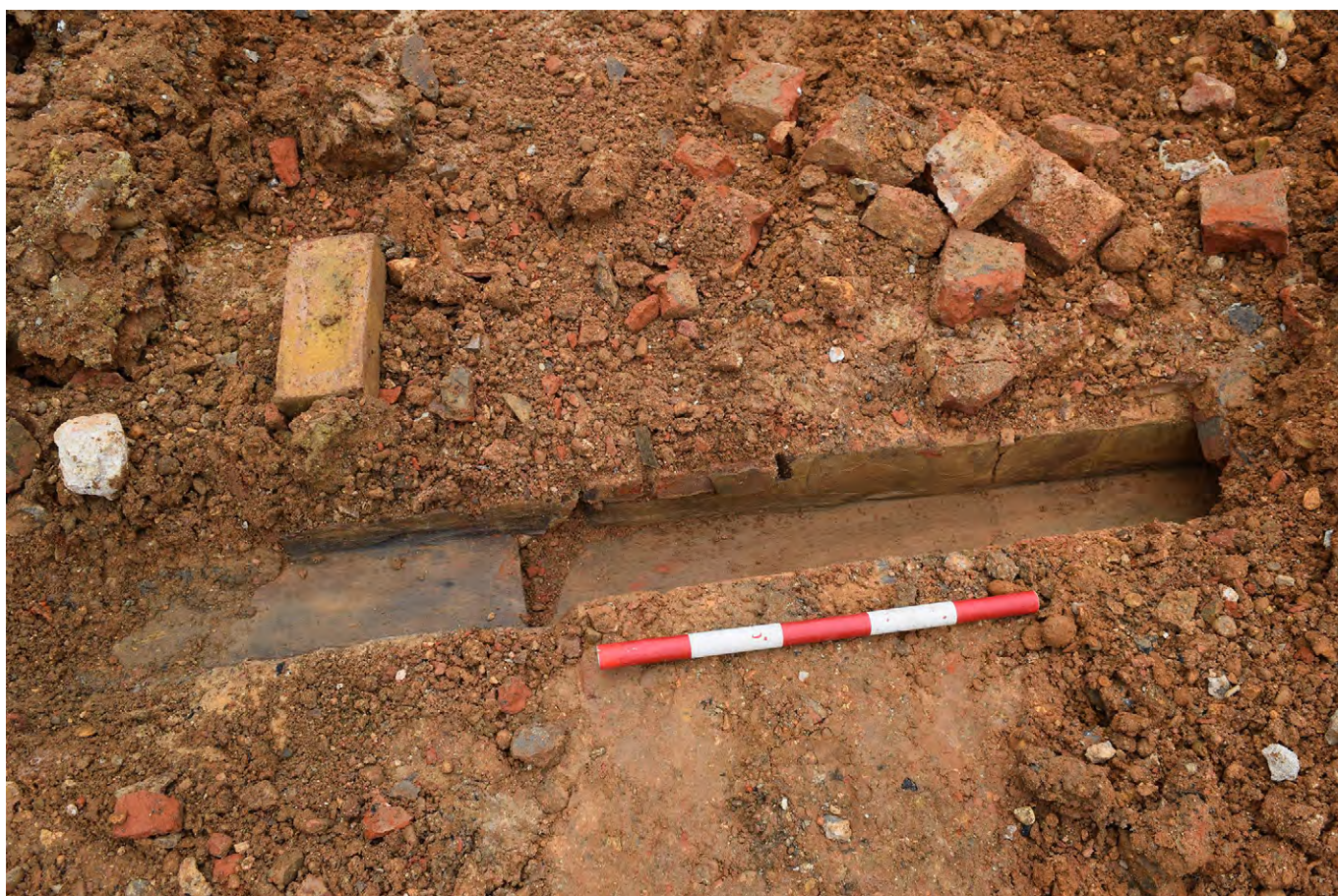
Plate F.57: Simple drainage trench in eastern third of terrace, looking west, showing drain [F.3.7]
