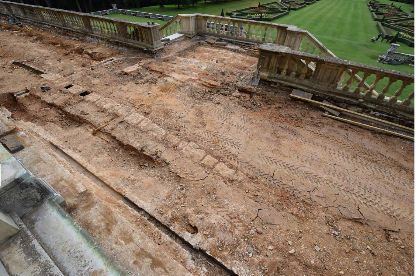
Plate F.26: Area of terrace immediately in front of mansion during works, looking south
