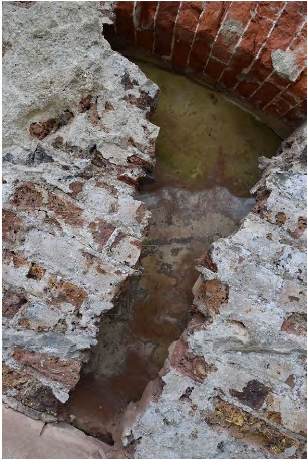
Plate B.16: Patch of removed brick in arch
