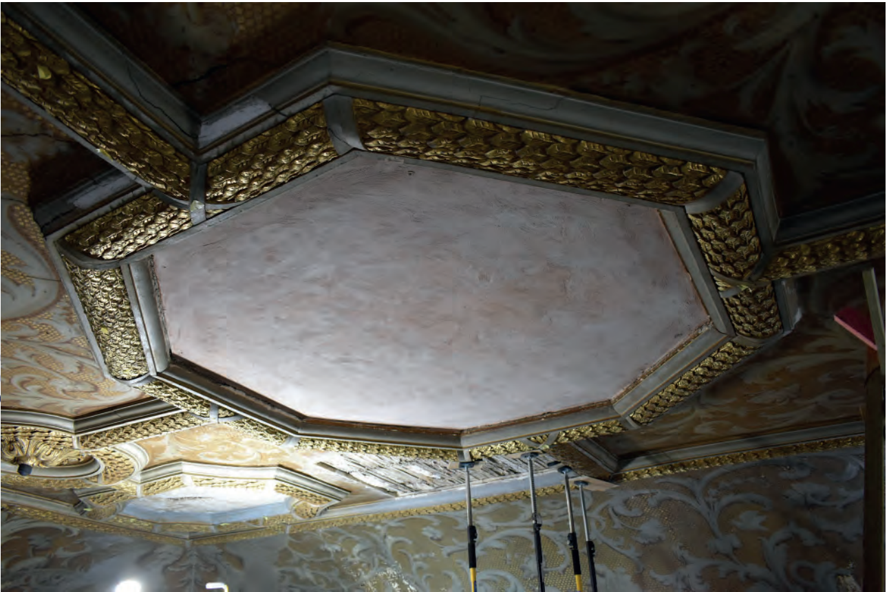
Plate 121: Dining Room, ceiling, example of earlier ceiling repair
