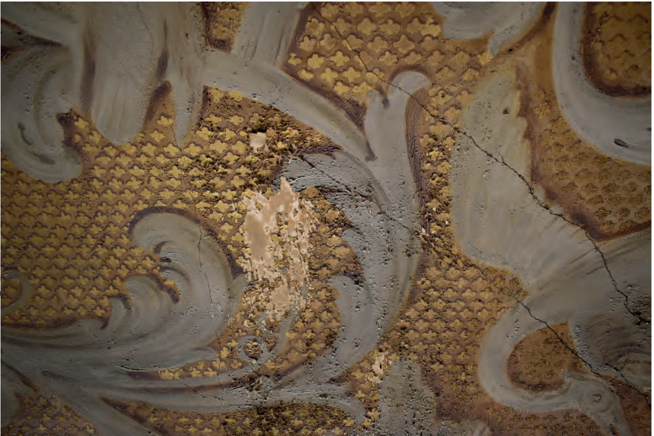
Plate 111: Dining Room, ceiling, example of flaking paint
