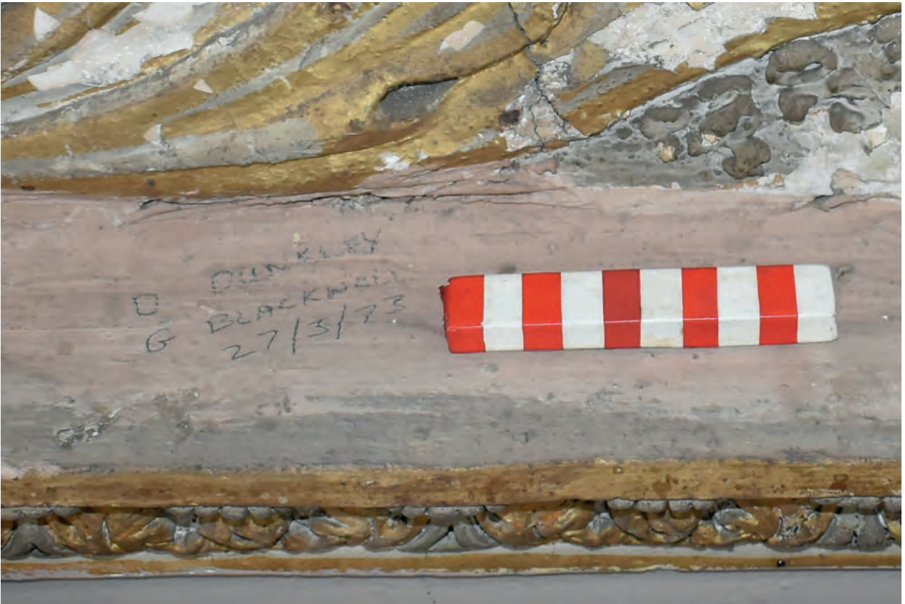
Plate 130: Dining Room, ceiling, example of graffiti
