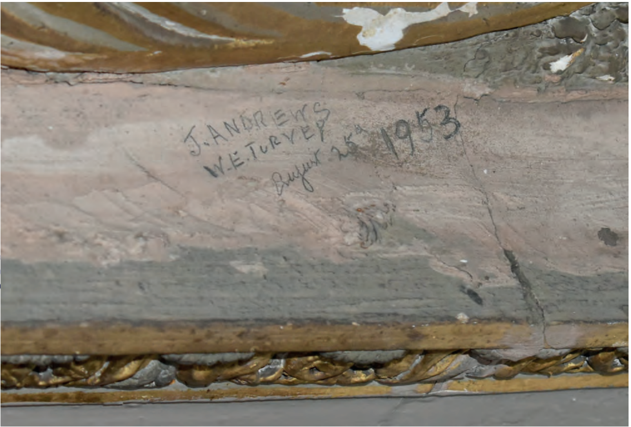
Plate 129: Dining Room, ceiling, example of graffiti
