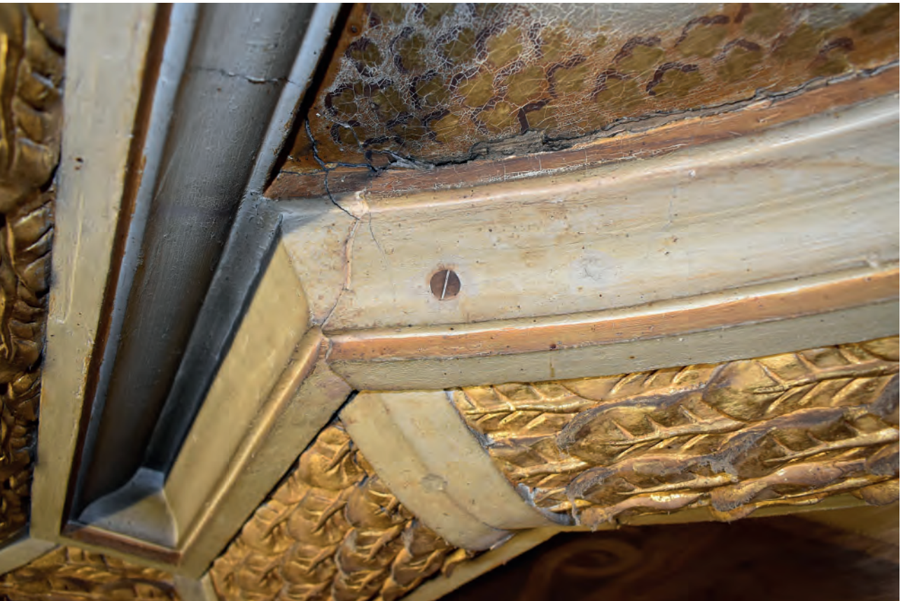
Plate 118: Dining Room, ceiling, example of poor repair of moulding
