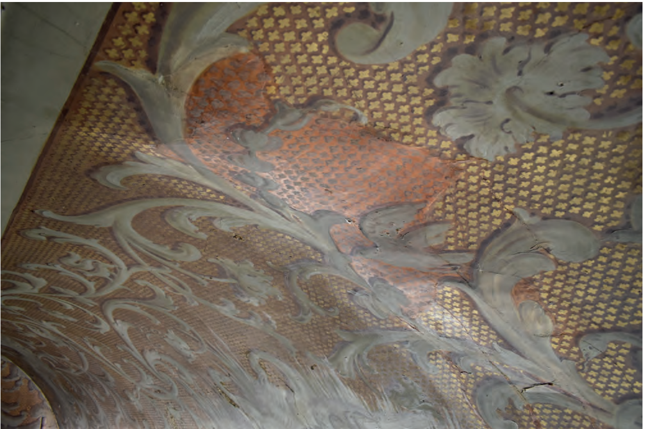
Plate 114: Dining Room, ceiling, example of poor repair and redecoration
