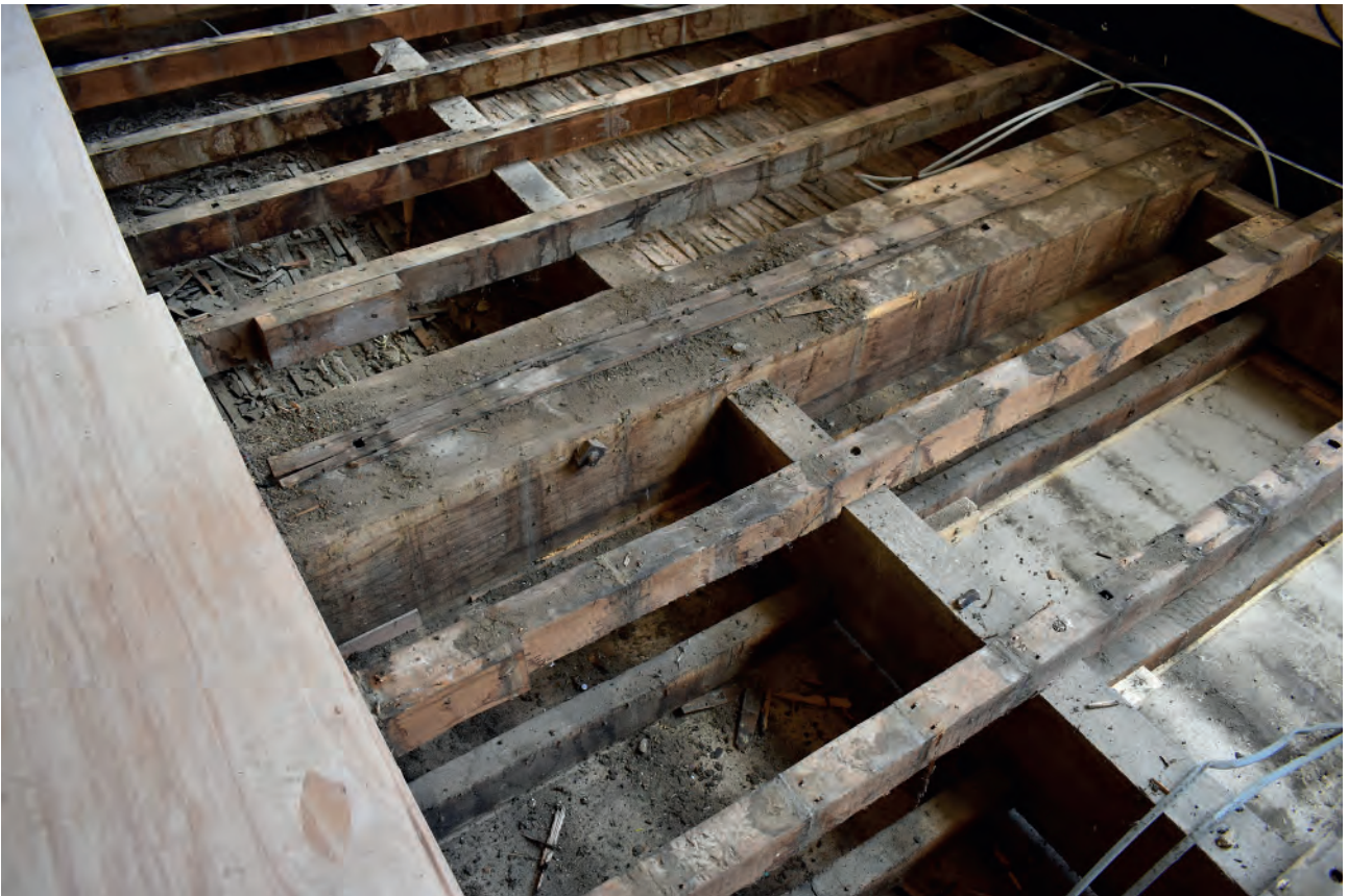
Plate 156: Dining Room, floor, example of primary and secondary beams and joists with ceiling below
