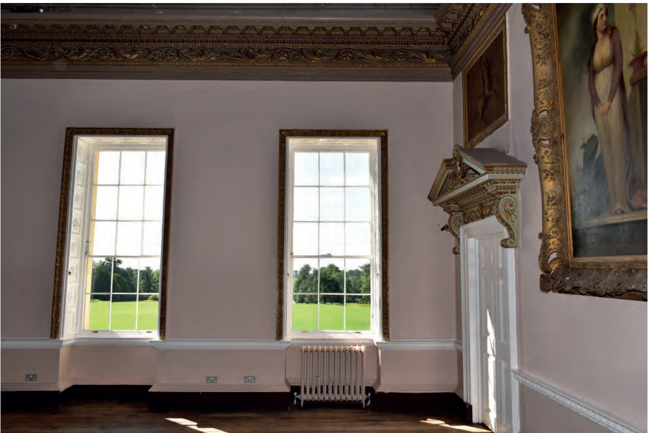
Plate 96: Dining Room, south wall, example of windows at the start of the project
