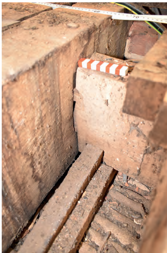
Plate 163: Dining Room, floor, example of joint between a secondary beam and joist
