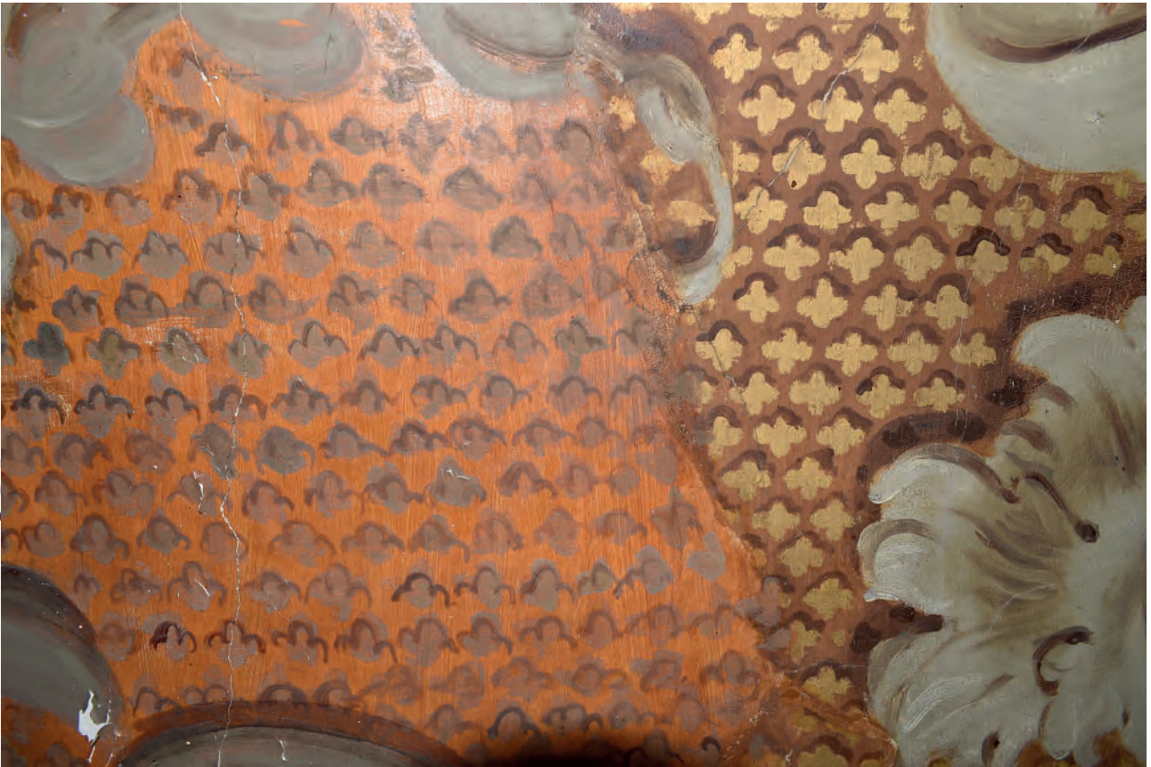
Plate 115: Dining Room, ceiling, example of poor repair and redecoration
