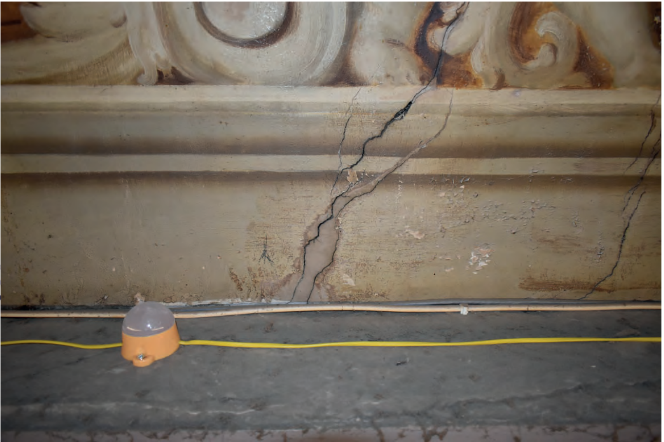
Plate 107: Dining Room, ceiling, example of poor earlier repair
