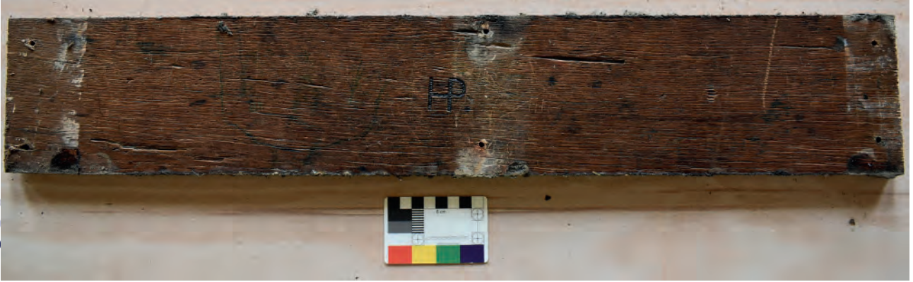
Plate 147: Dining Room, floor, example of furniture used to patch the floorboards
