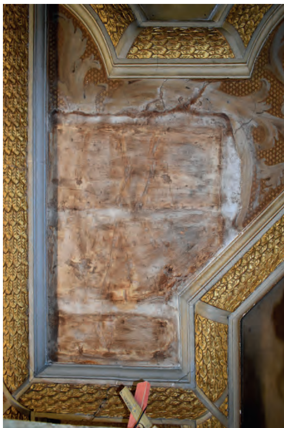
Plate 119: Dining Room, ceiling, area of damage and poor repair to the west end
