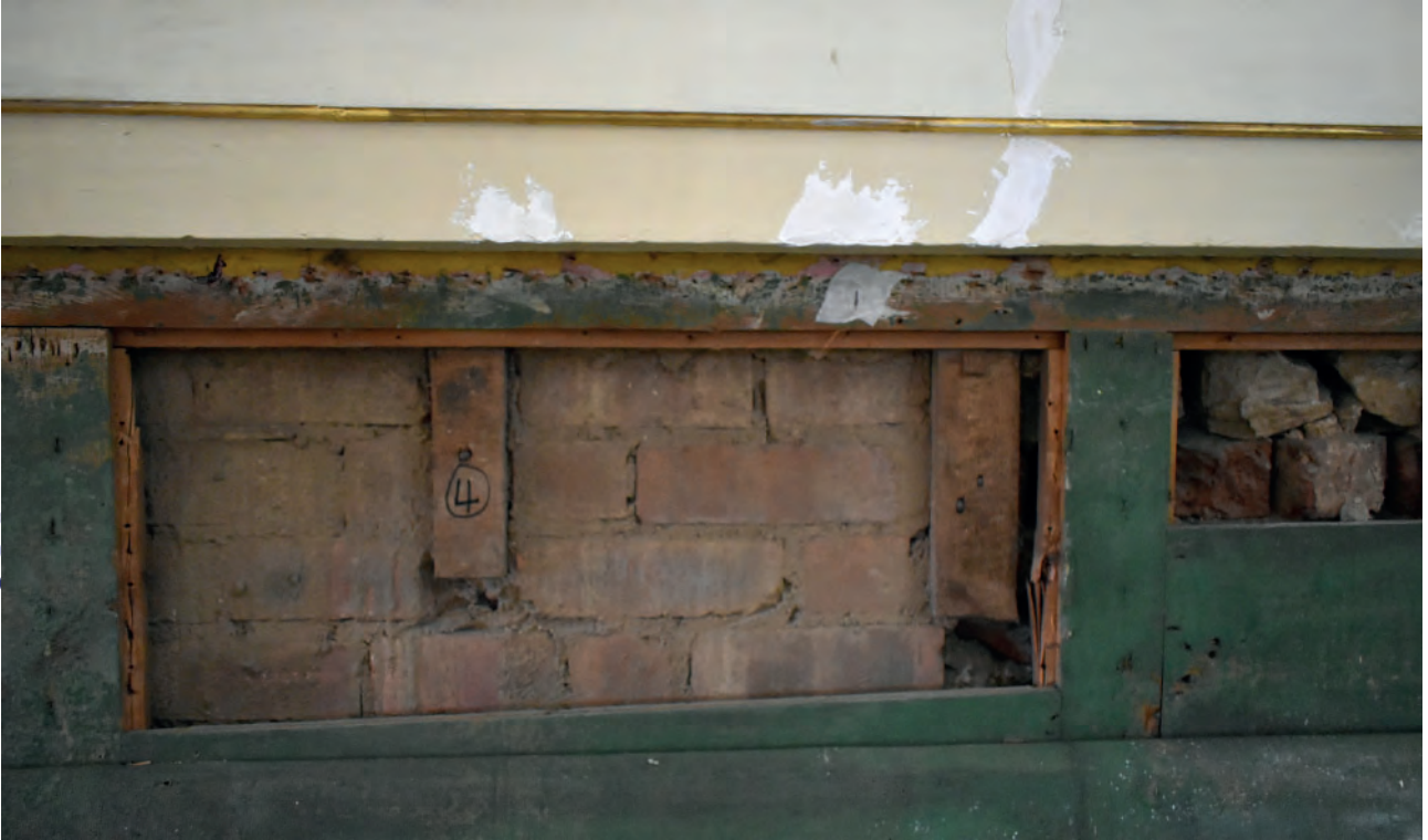
Plate 33: Temple Room, west wall, modern brickwork
