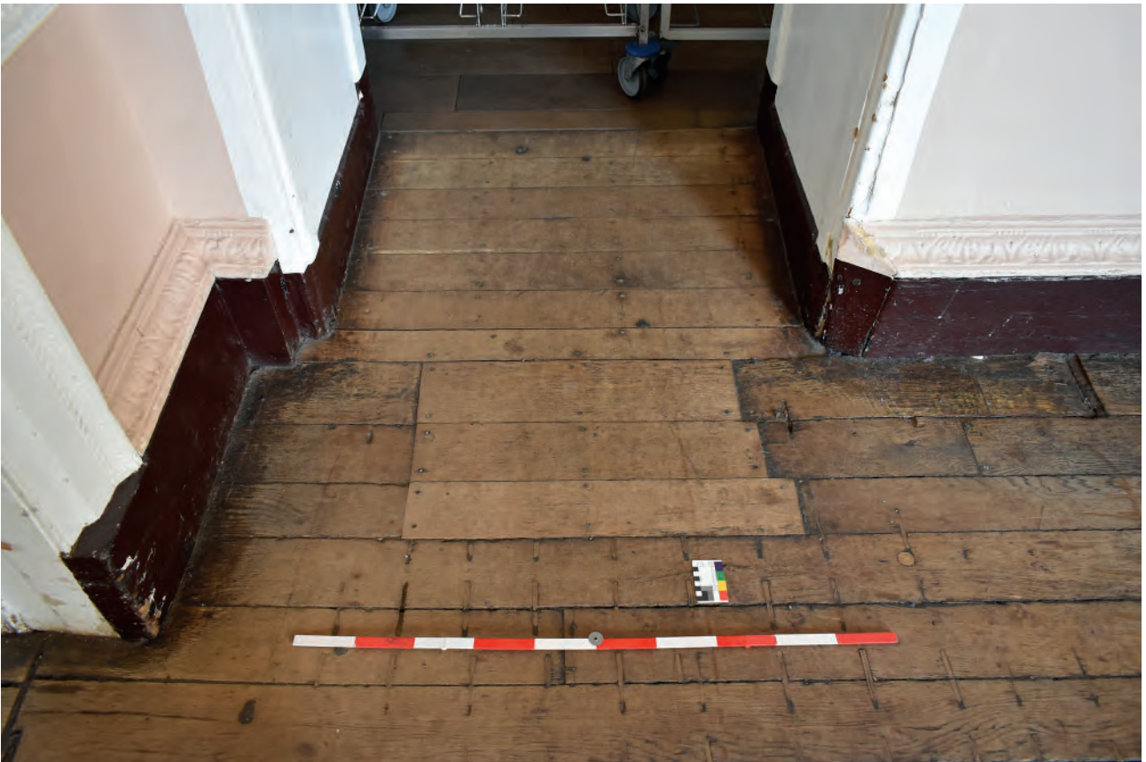
Plate 144: Dining Room, floor, example of patching of the floorboards
