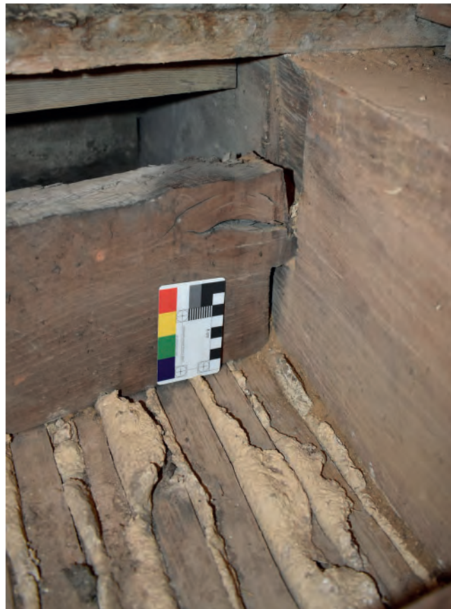
Plate 190: West Corridor, floor, example of the joint between joists and westernmost beam
