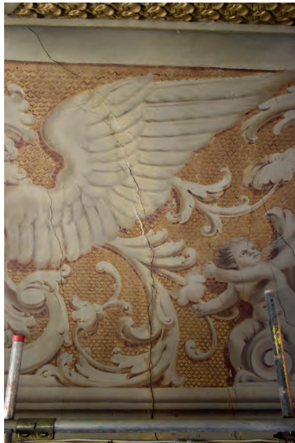
Plate 108: Dining Room, ceiling, example of cracking
