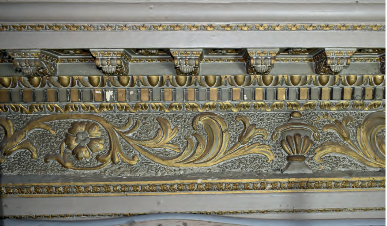
Plate 113: Dining Room, ceiling, example of dirt to decoration
