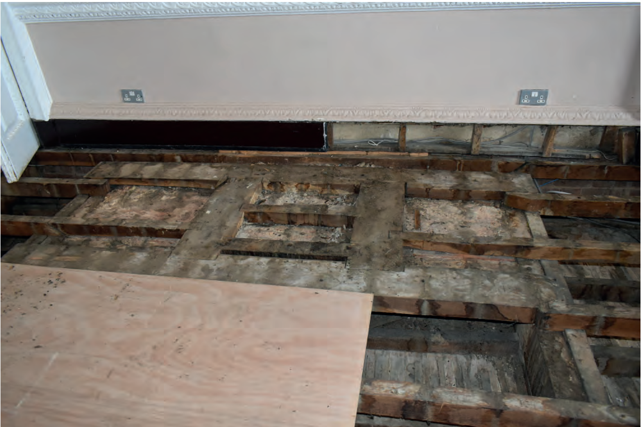
Plate 166: Dining Room, floor, strengthened feature at the east end of the room
