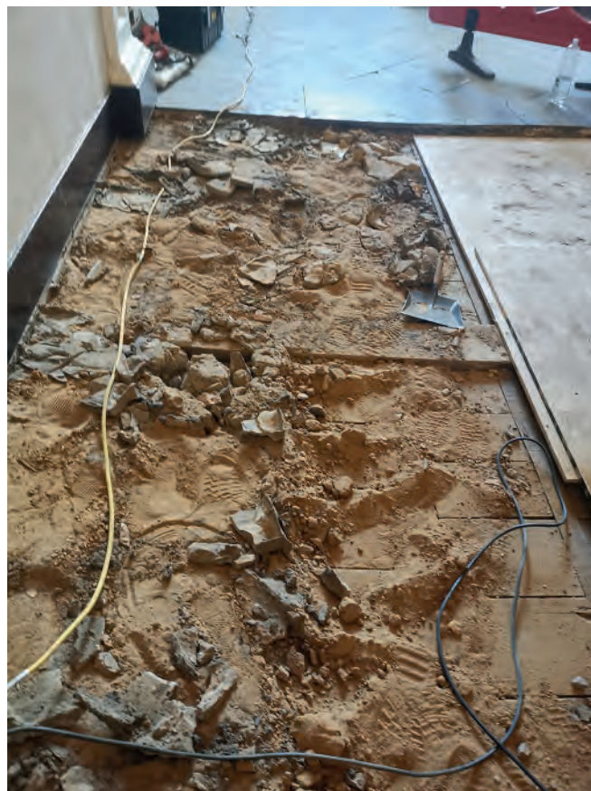
Plate 184: West Corridor, floor, sandy levelling layer (provided by Nick Jones of Messenger)
