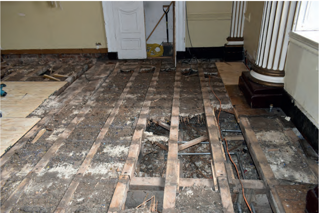
Plate 80: Temple Room, floor, area of damaged pugging exposing floor structure
