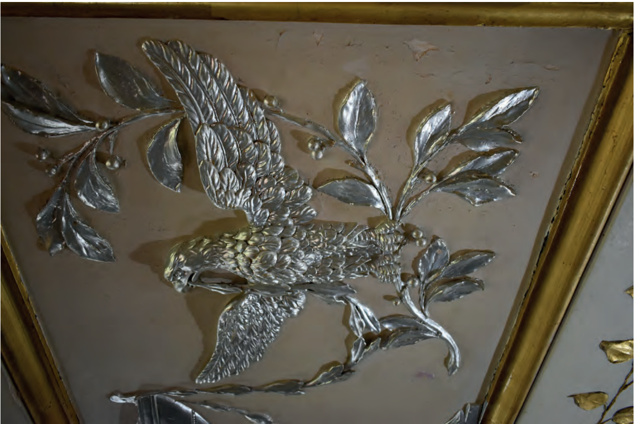
Plate 14: Temple Room, ceiling, example of flaking paint
