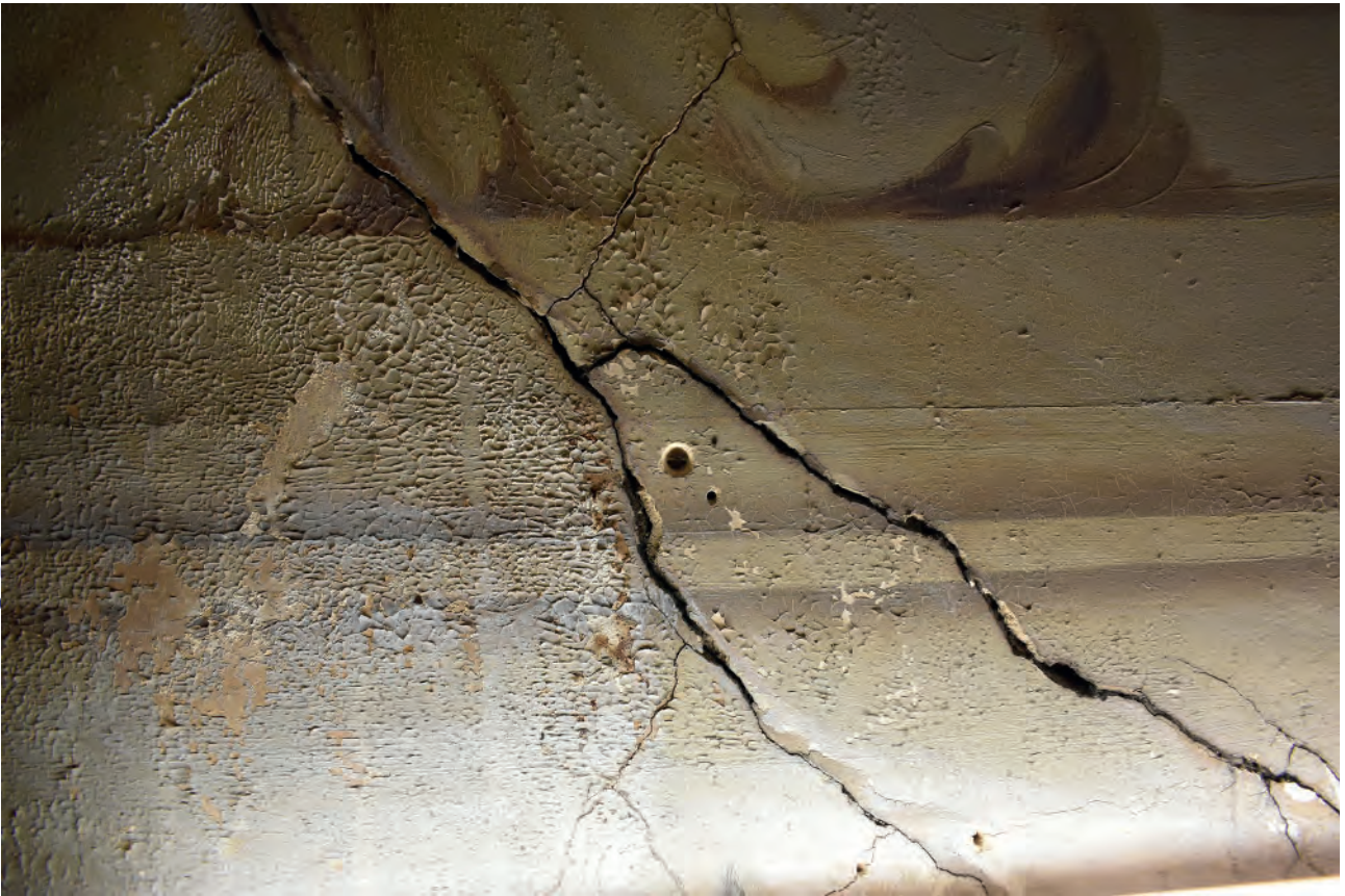
Plate 105: Dining Room, ceiling, example of poor earlier repair
