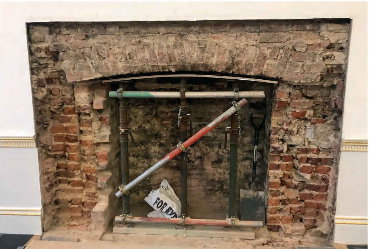
Plate 64: Temple Room, fireplace following stripping of 1922 material (provided by Nick Jones of Messenger)
