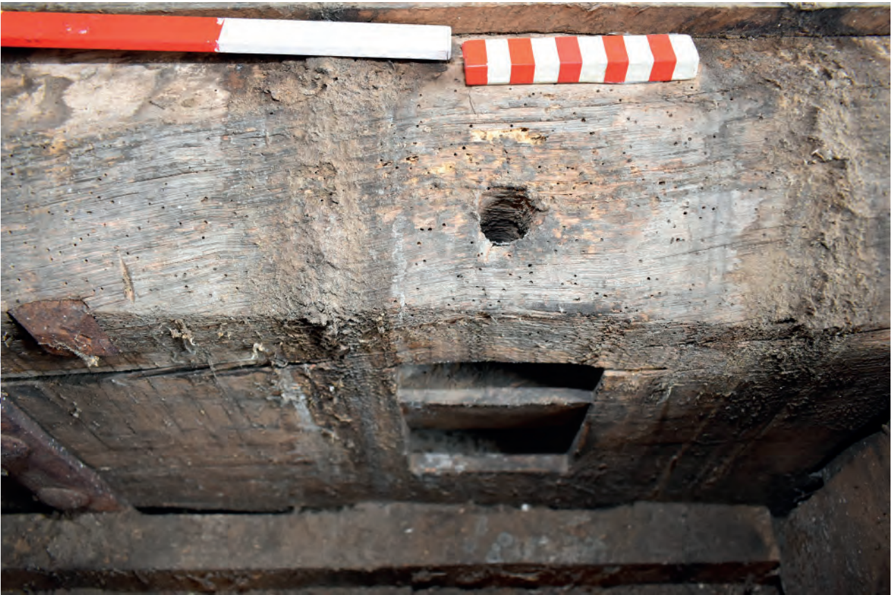
Plate 169: Dining Room, floor, redundant mortice at the west end of the room
