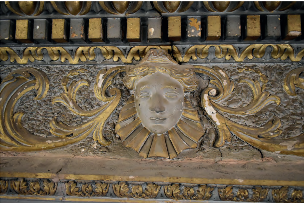
Plate 112: Dining Room, ceiling, example of dirt to decoration
