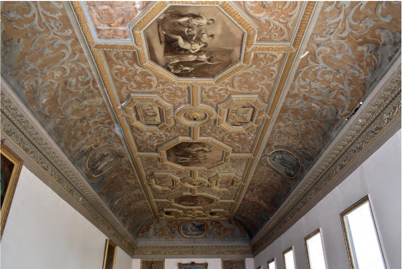
Plate 101: Dining Room, ceiling, before conservation work, looking east
