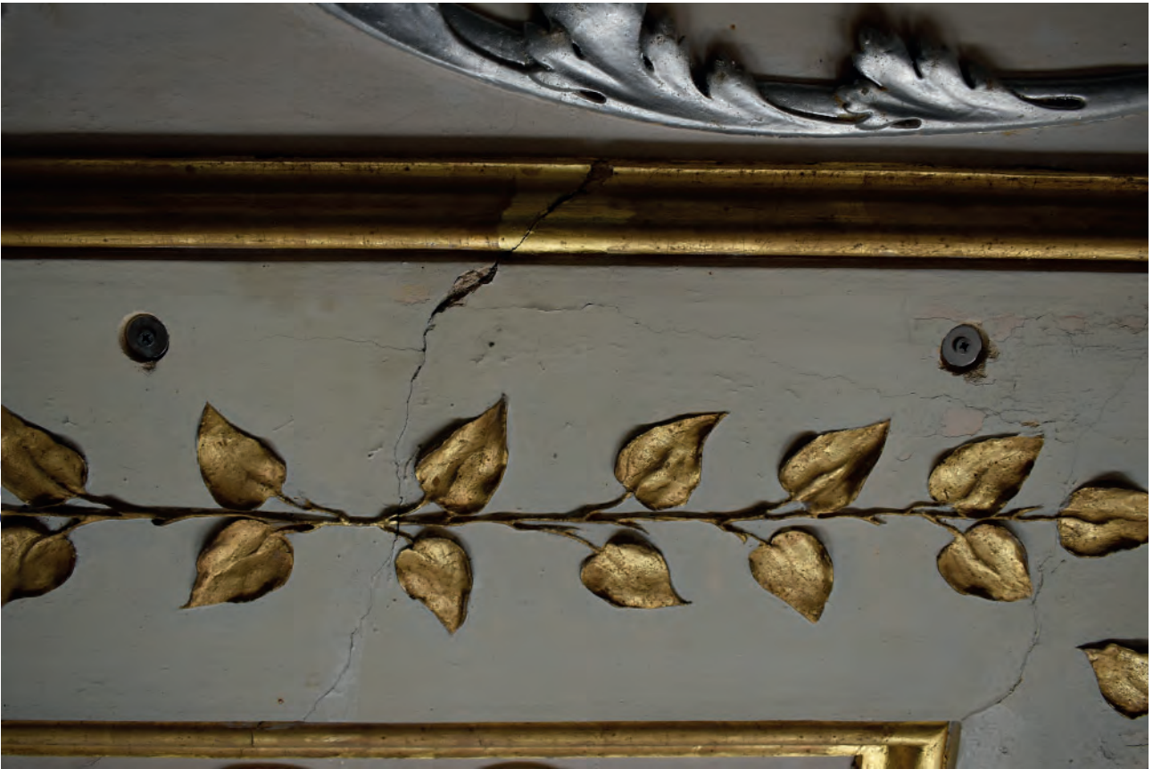
Plate 13: Temple Room, ceiling, example of cracking
