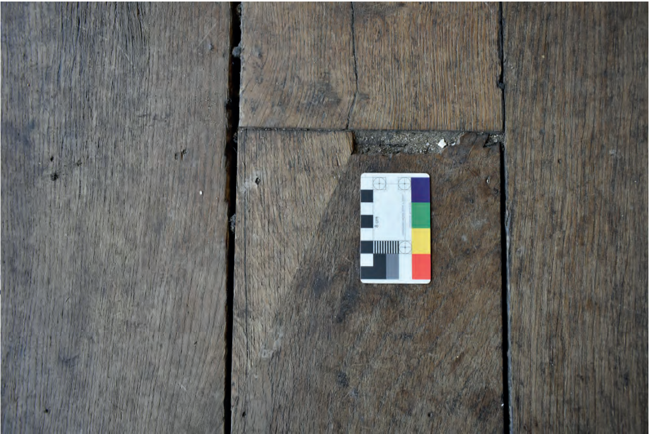
Plate 151: Dining Room, floor, example of early repair to the floorboards
