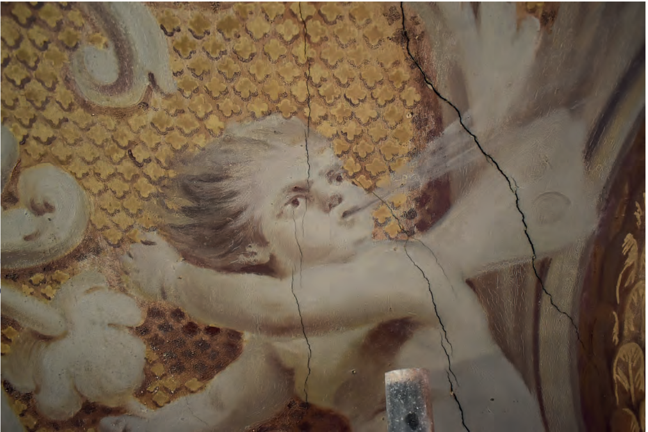
Plate 109: Dining Room, ceiling, example of cracking
