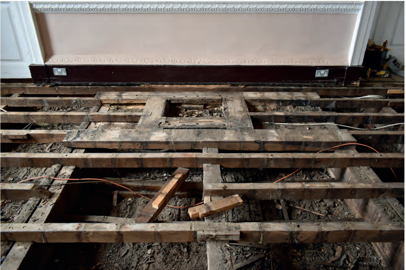
Plate 167: Dining Room, floor, strengthened feature at the west end of the room
