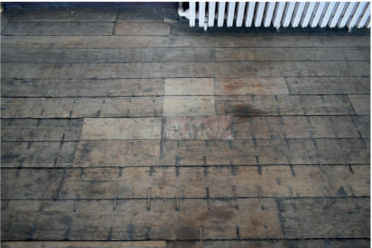
Plate 150: Dining Room, floor, example of worn floorboards
