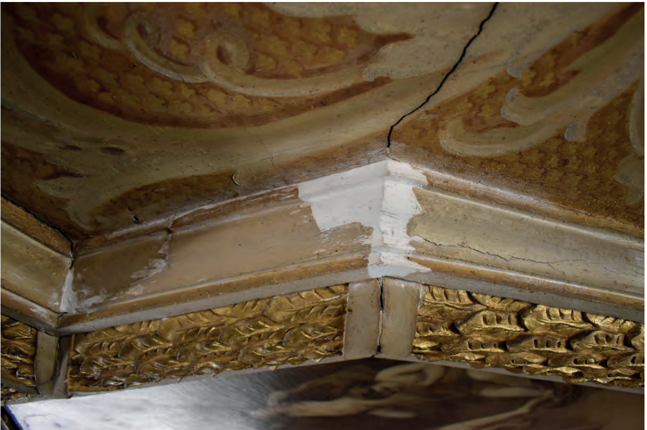
Plate 106: Dining Room, ceiling, example of poor earlier repair
