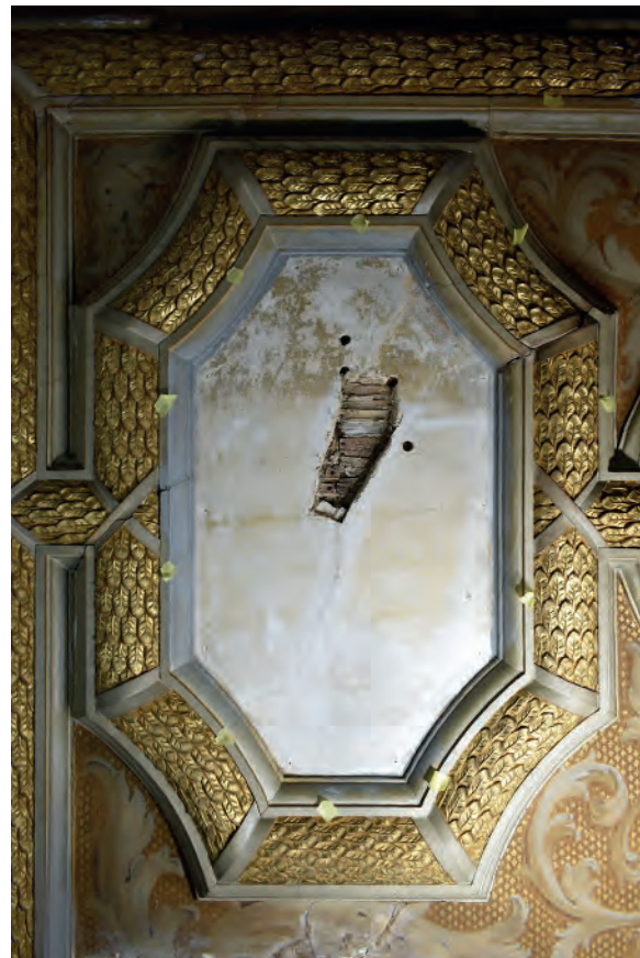
Plate 122: Dining Room, ceiling, example of earlier ceiling repair
