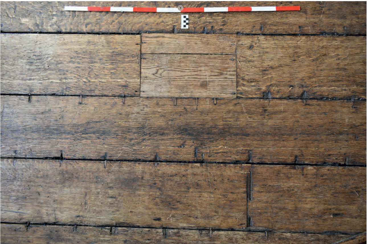
Plate 66: Temple Room, floor, example of floorboard wear
