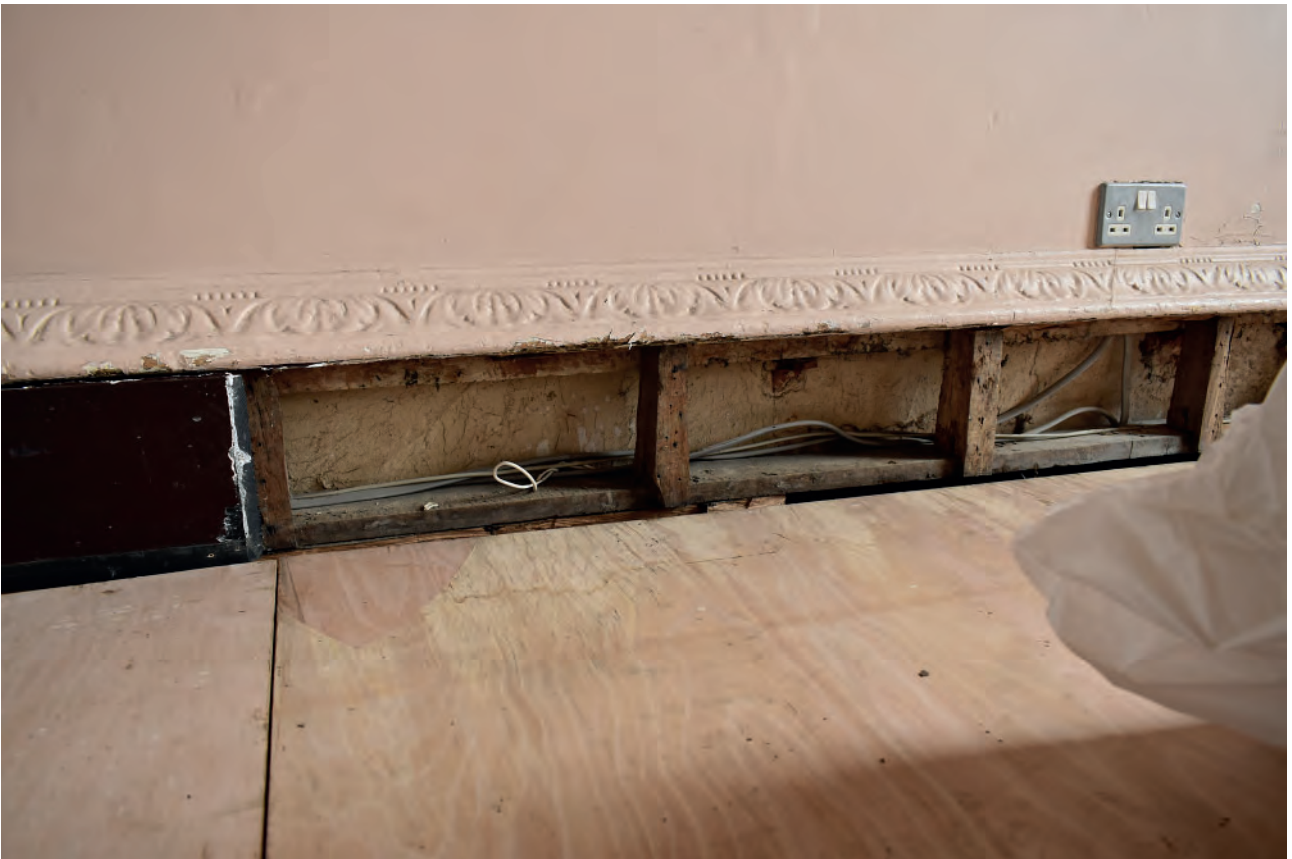
Plate 136: Dining Room, wall, example of rough plaster behind wall surface
