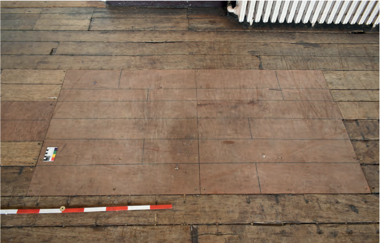
Plate 145: Dining Room, floor, example of patching of the floorboards
