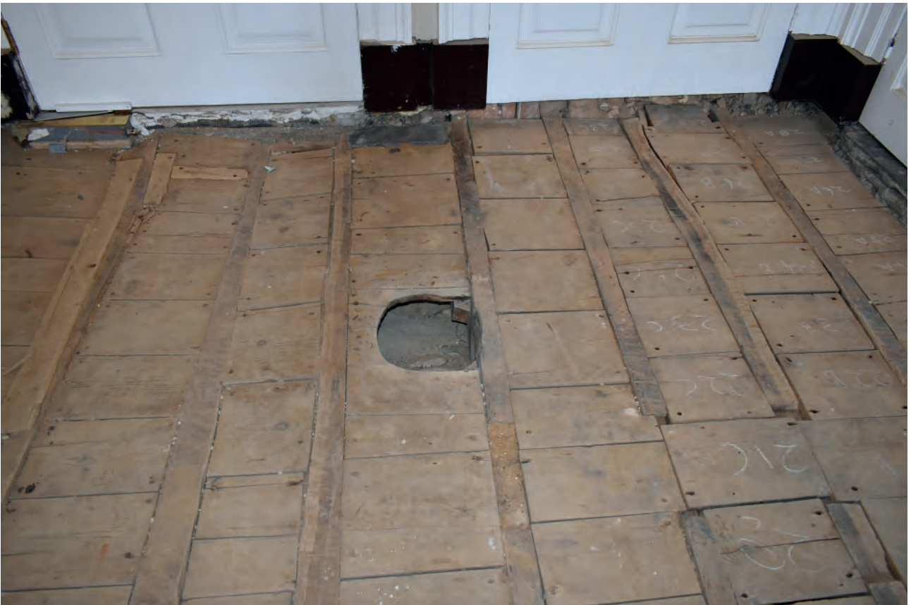
Plate 188: West Corridor, floor, hole in the east end of the pugging boards
