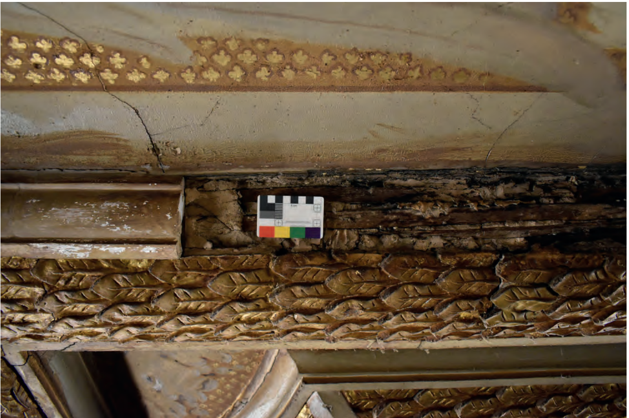
Plate 116: Dining Room, ceiling, example of poor condition of decorative beam
