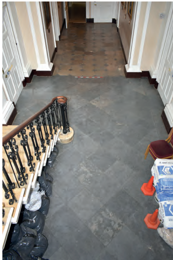
Plate 182: West Corridor, floor, later floor covering to west
