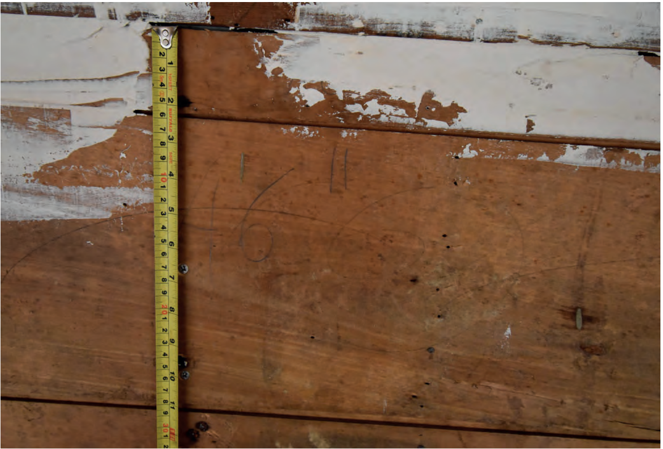
Plate 58: North wall, panel 7, example of graffiti
