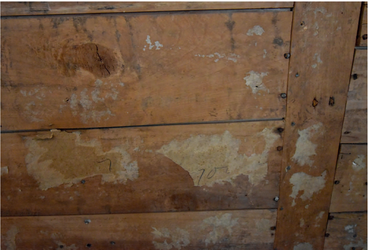
Plate 59: North wall, panel 11, example of graffiti
