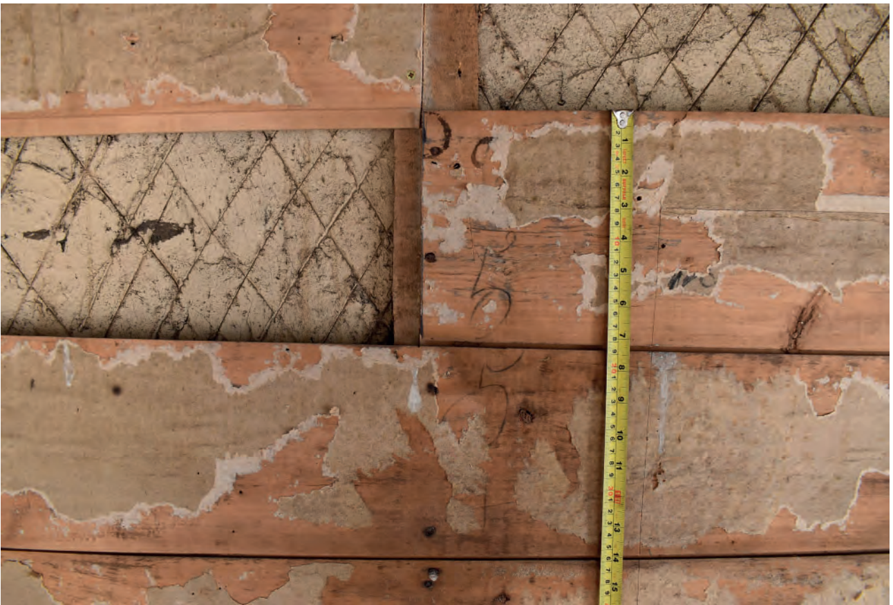
Plate 105: South wall, panel 5, example of second type of numbering
