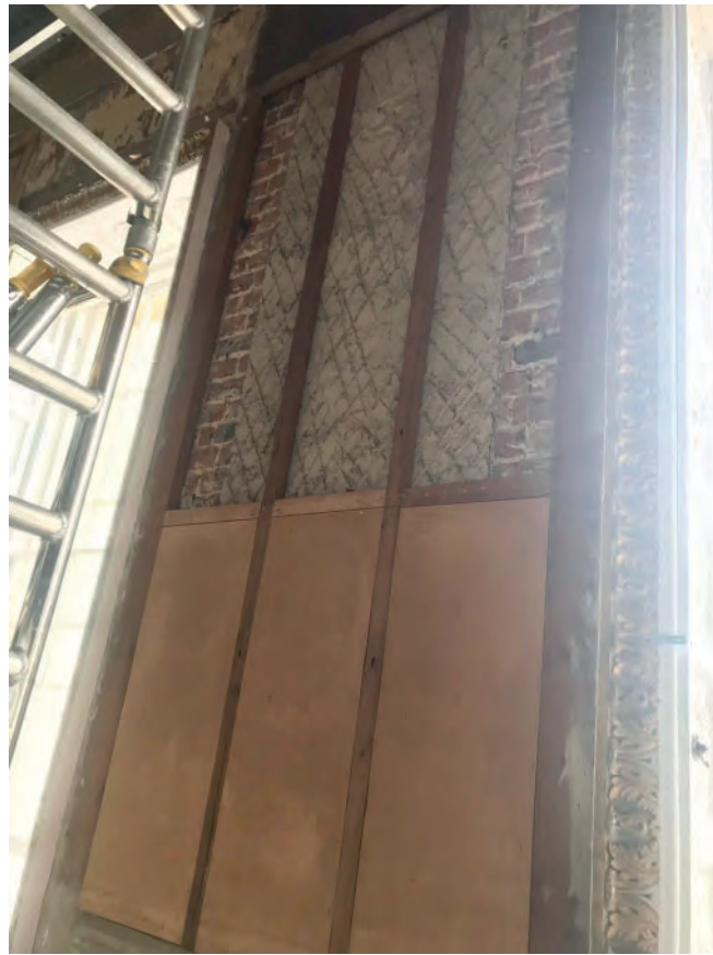
Plate 38: South wall, hardboard between windows
