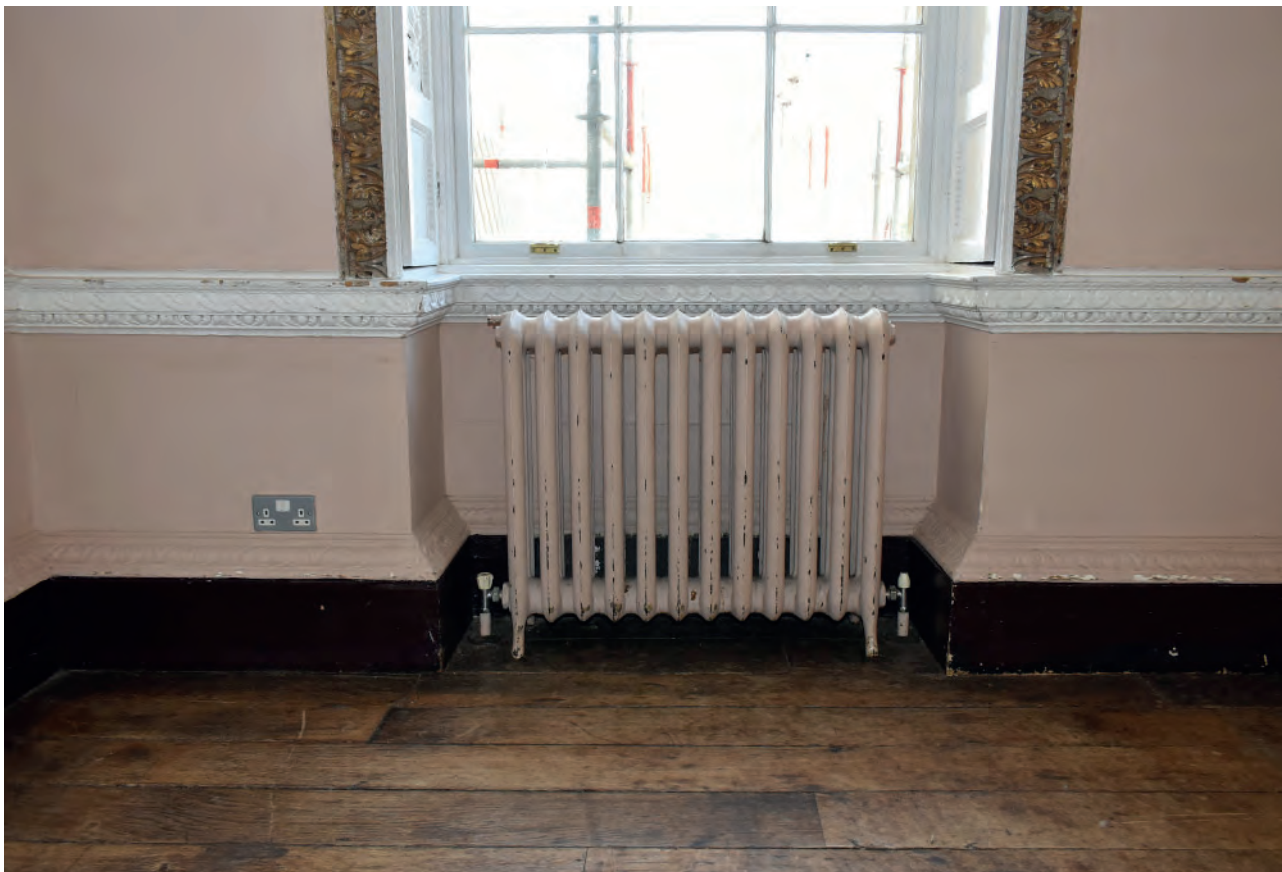
Plate 5: Example of a radiator to the south wall
