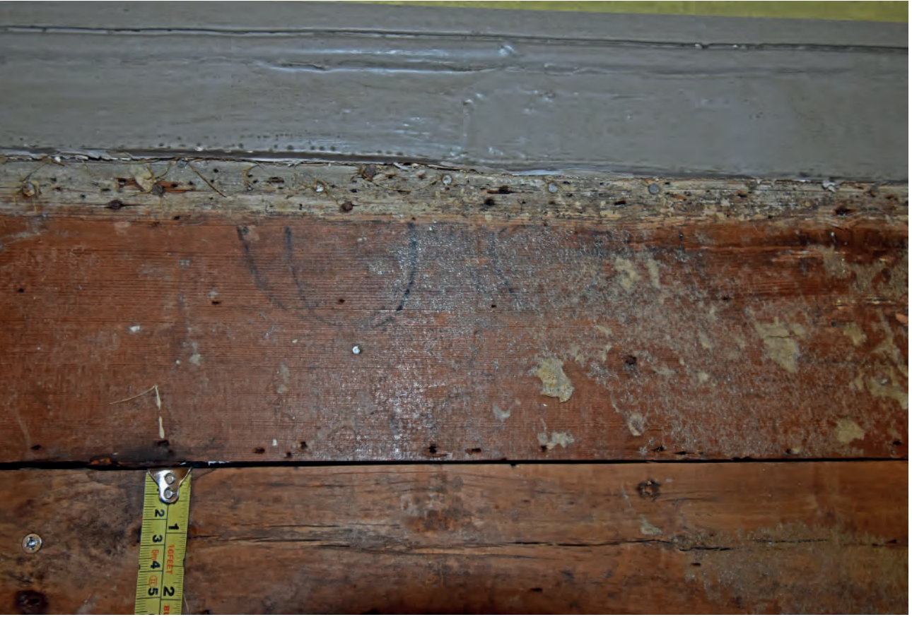
Plate 68: North wall, panel 5, example of graffiti
