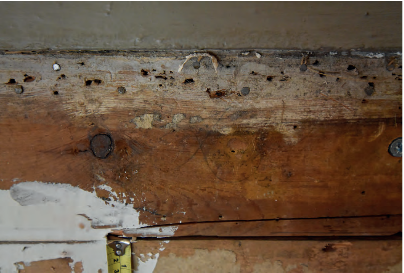
Plate 69: North wall, panel 12, example of graffiti
