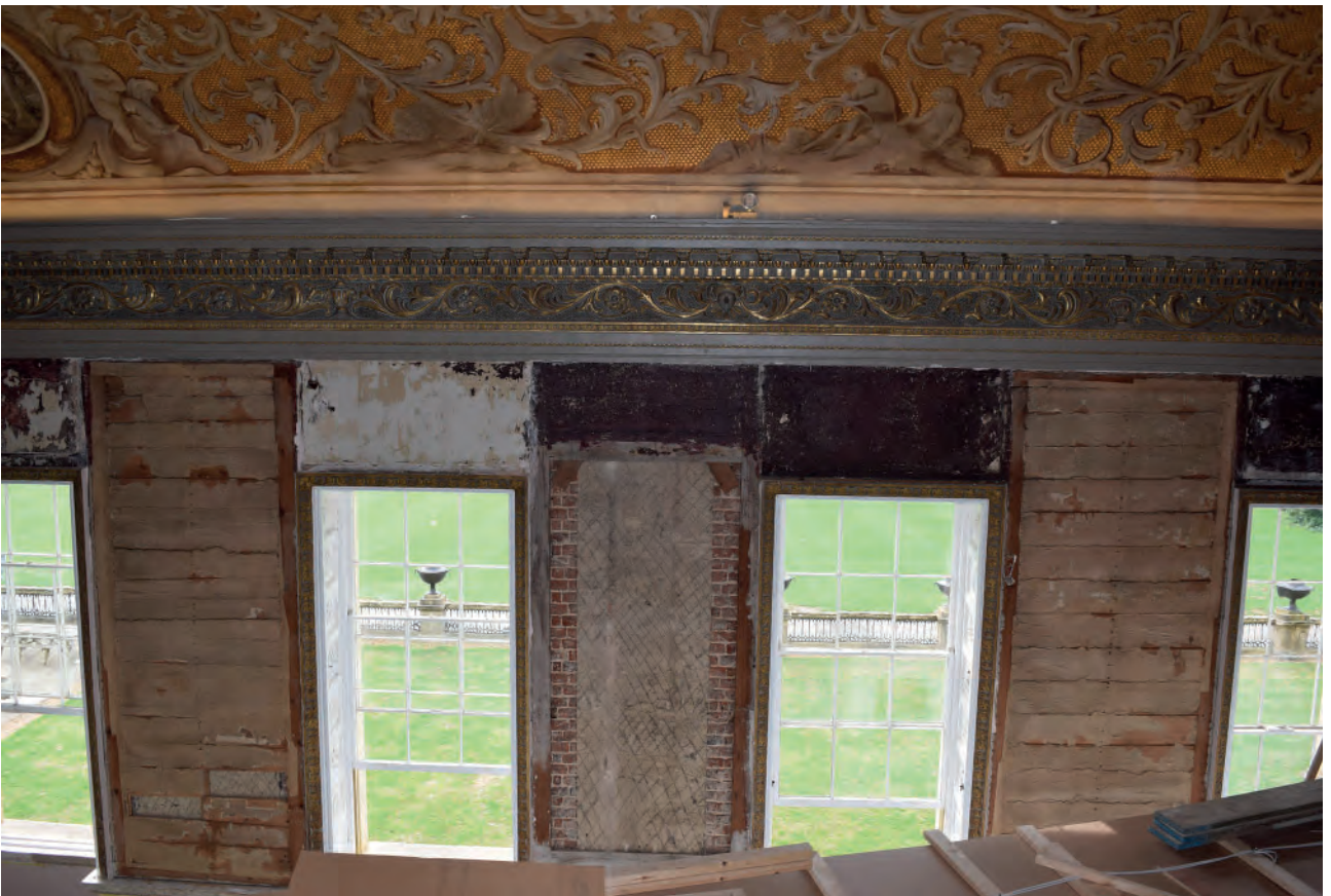
Plate 37: South wall, modern plaster between windows
