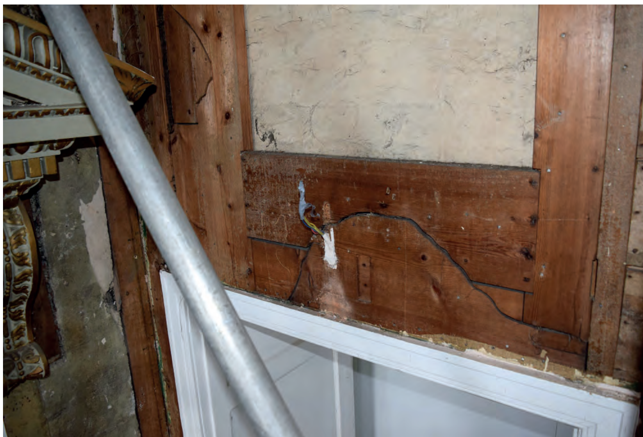
Plate 113: North wall, lower part of reused door, masked place of removal of lower hinge and irregular shape cut
