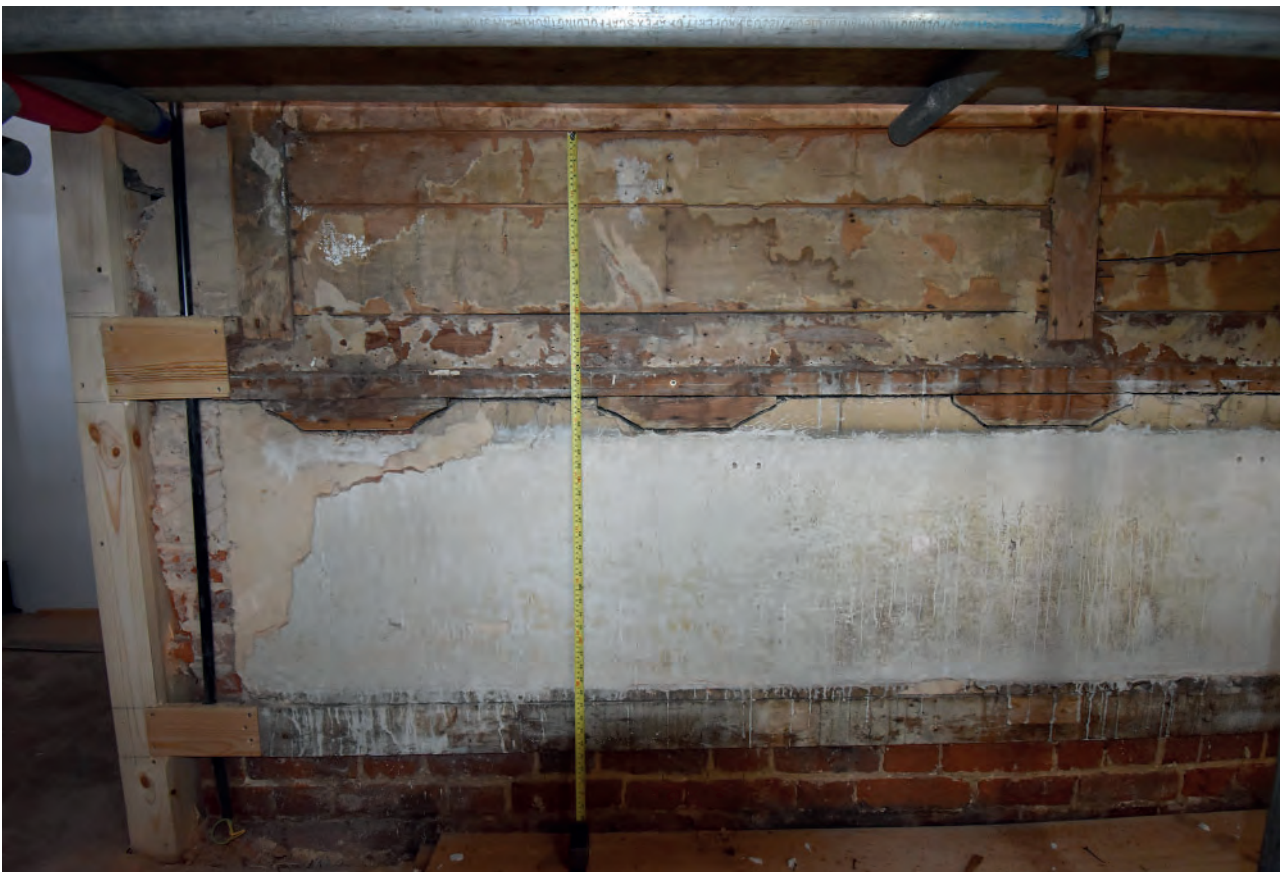
Plate 118: North wall, west part of dado between west door and west fireplace
