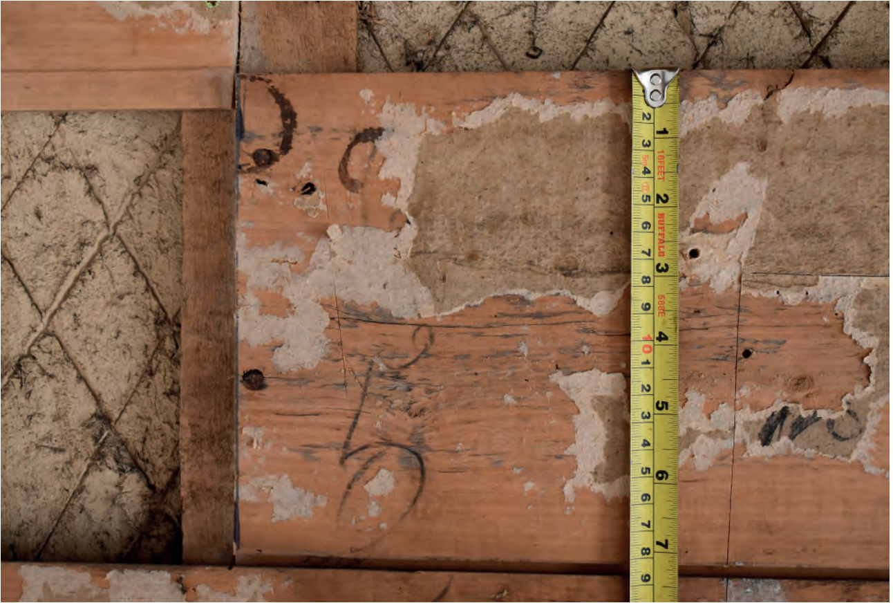
Plate 154: South wall, fifth panel, exemplar of graffiti
