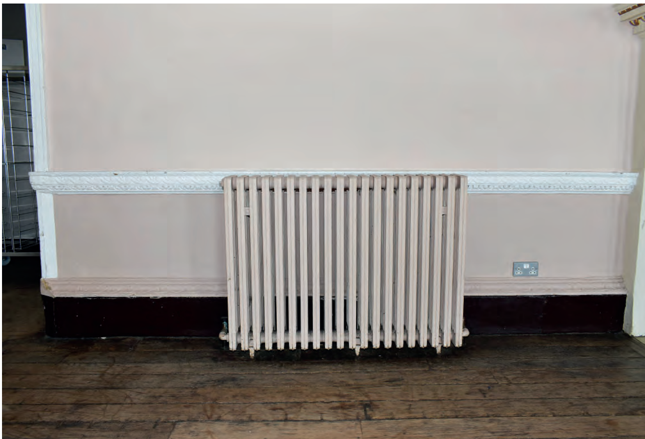
Plate 6: Example of a radiator to the north wall
