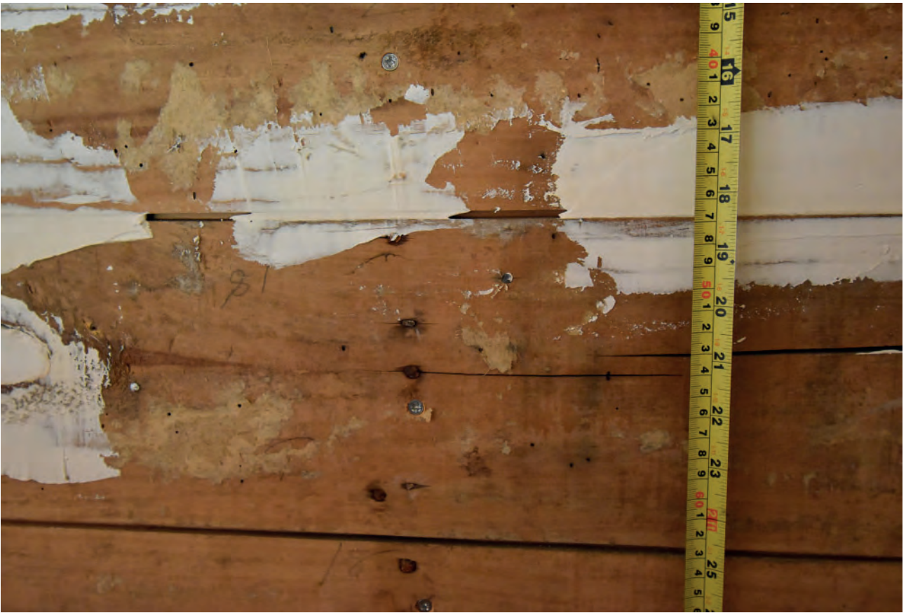
Plate 60: North wall, panel 12, example of graffiti
