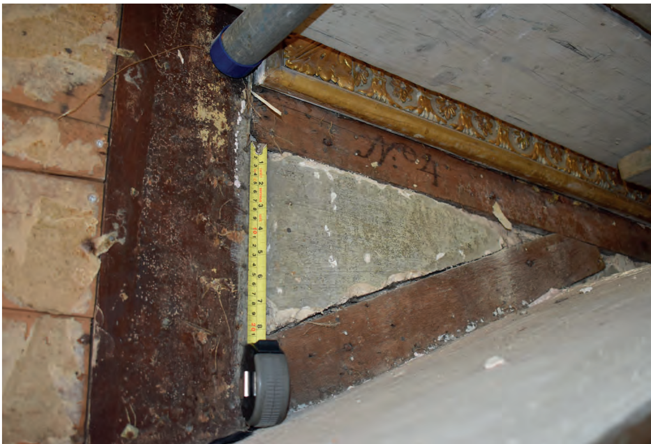
Plate 149: West wall, north door pediment, exemplar of graffiti
