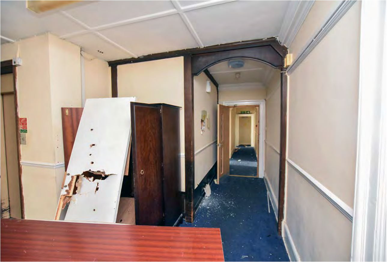
Plate 58: The hallway on the first floor of the east wing, Harecombe Manor, looking north
