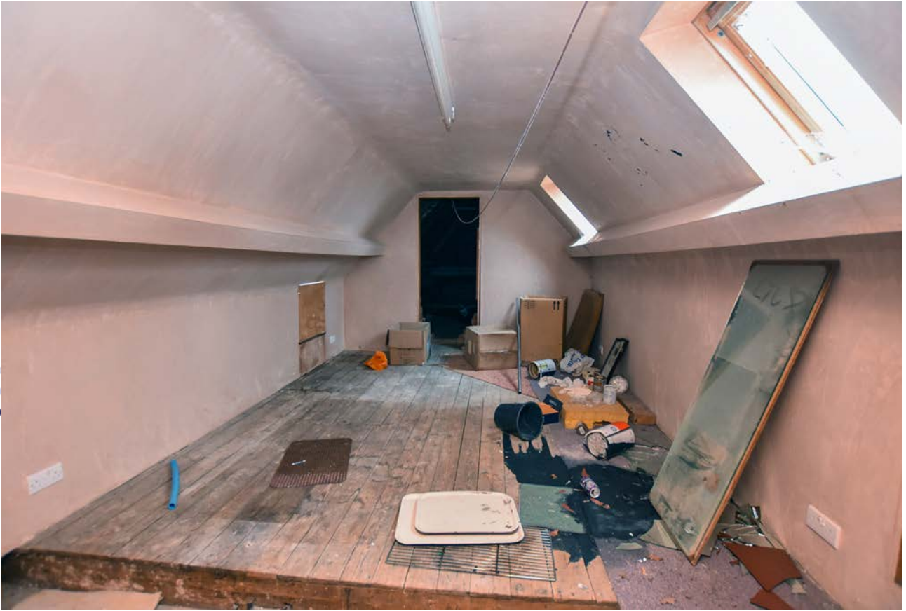
Plate 77: Large room in the east side of the loft at Harecombe Manor, looking east
