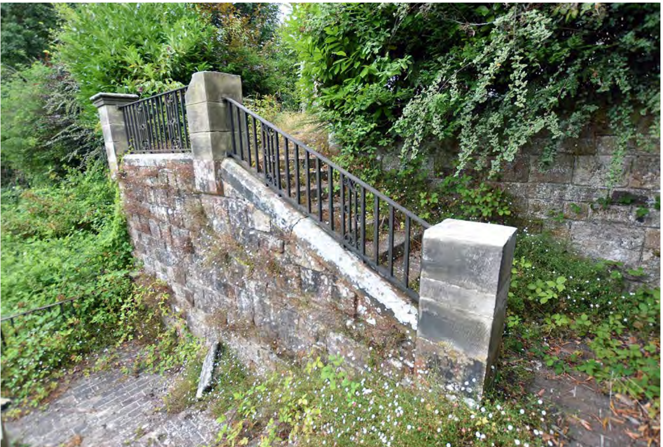
Plate 8: The stairway of the second level of the terraced garden, looking west
