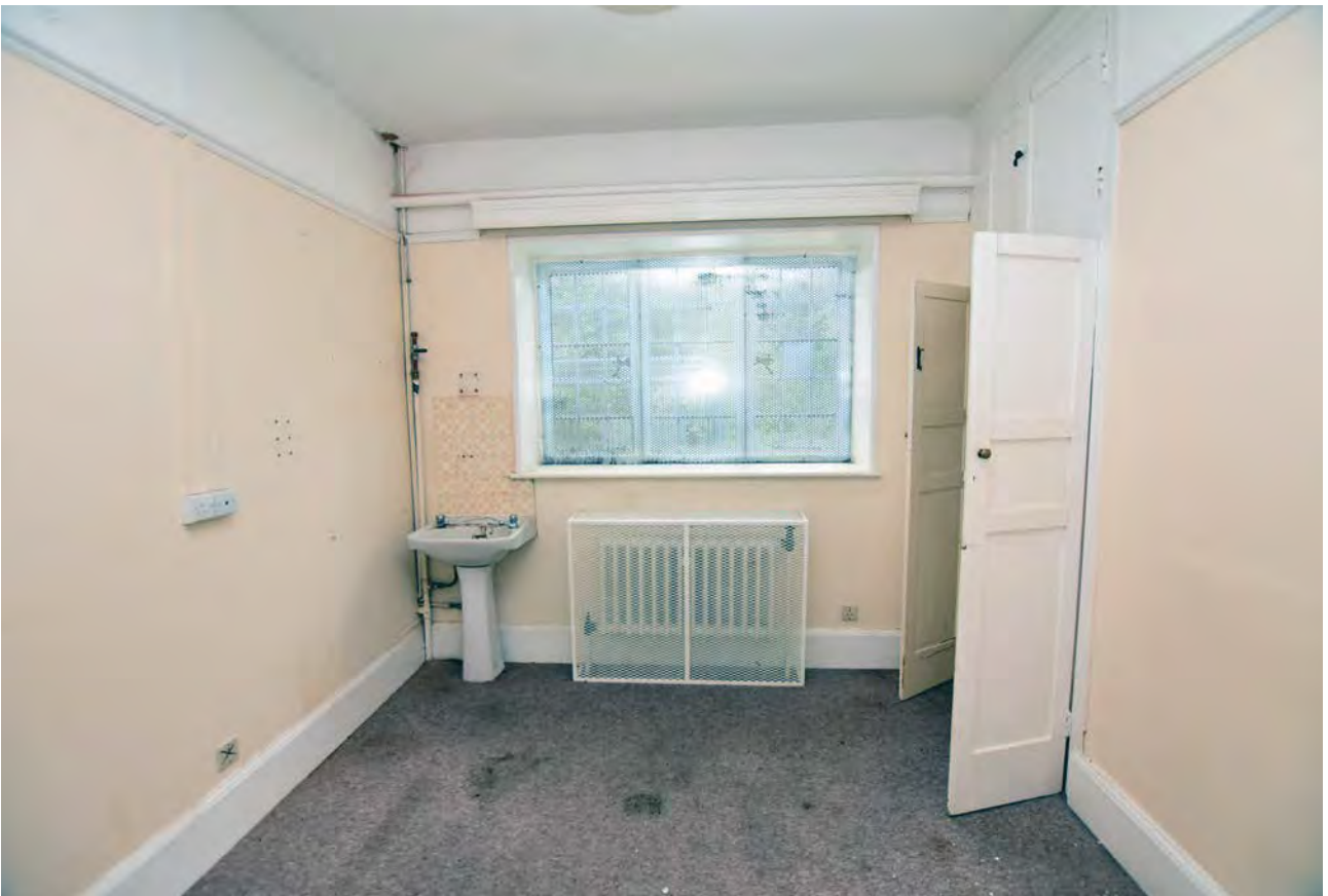
Plate 47: Room in the ground floor of the service wing in Harecombe Manor, looking north-west
