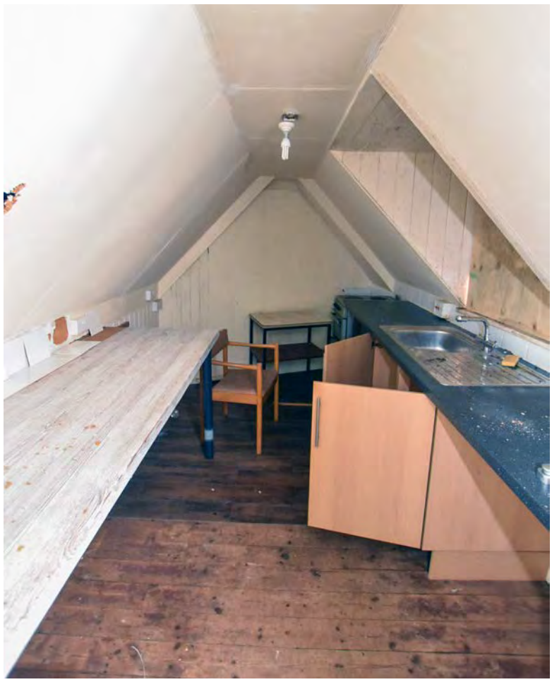
Plate 75: Small kitchen off the south room in the loft of Harecombe Manor, looking west
