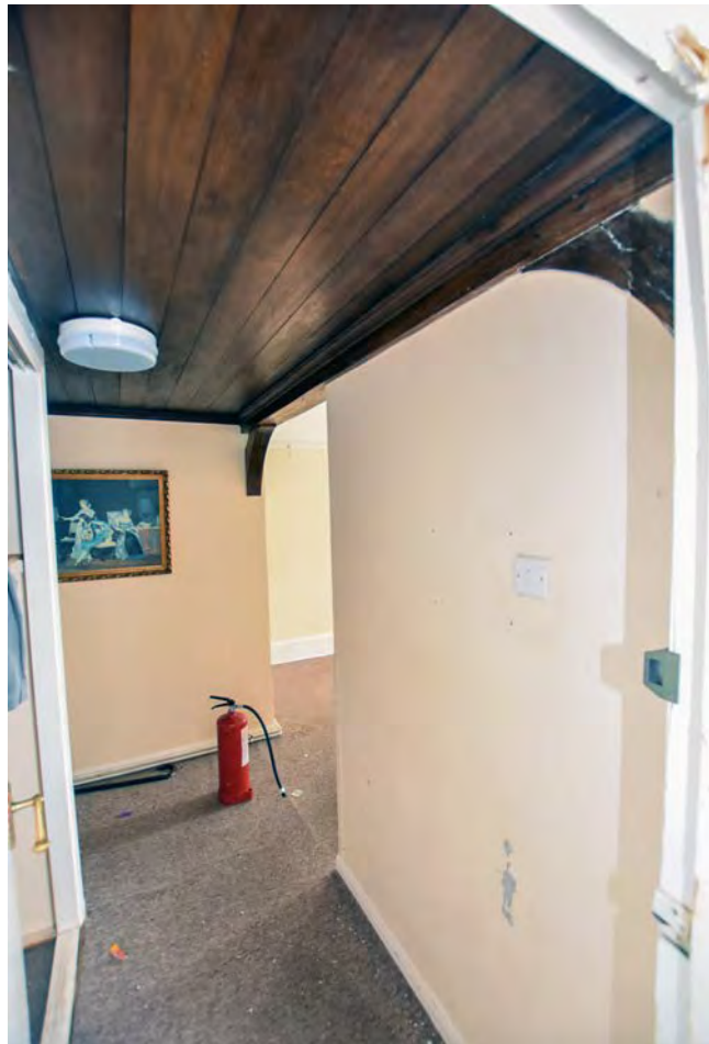
Plate 54: Storage space converted into a passage into the subdivided west bedroom on the first floor of the main axis, Harecombe Manor, looking south-east
