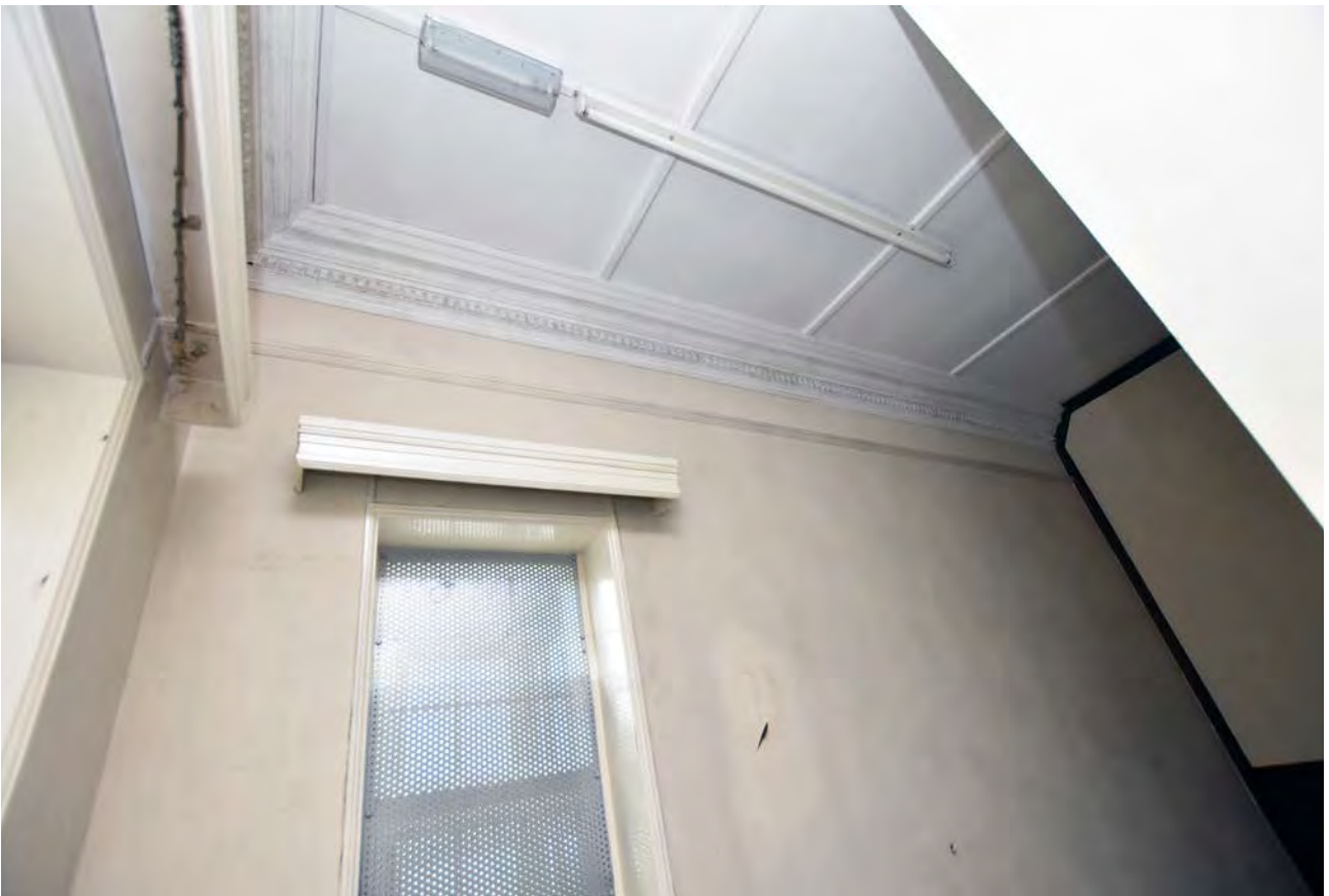
Plate 49: Architectural detailing in the main stairway from the ground to the first floor
