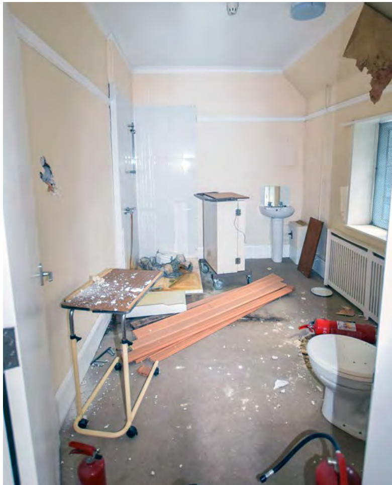
Plate 60: Wet room off the lounge on the first floor of the east wing, Harecombe Manor, looking north
