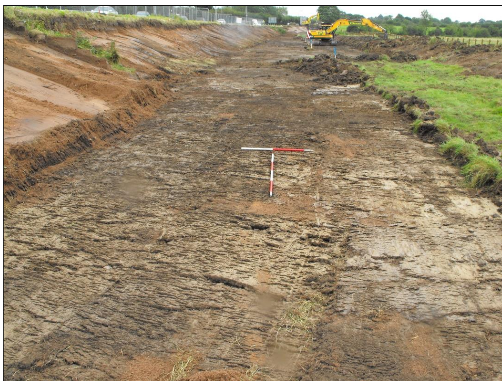
Plate 4: East side of Area 2 after topsoil stripping, looking east, 1 and 2m scales
