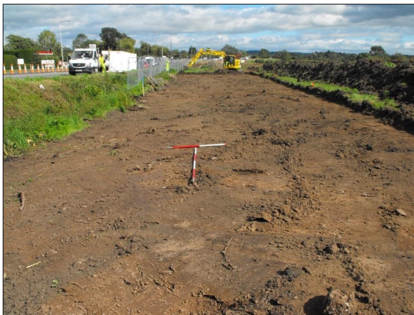
Plate 5: West end of Area 2 being topsoil stripped, looking east, 1 and 2m scales
