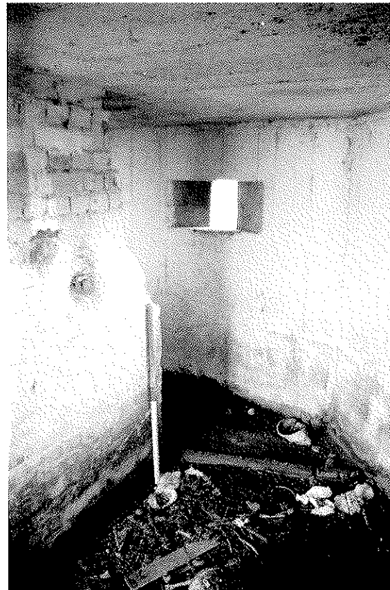
Plate 3: Partially demolished brick baffle in Pill Box A
