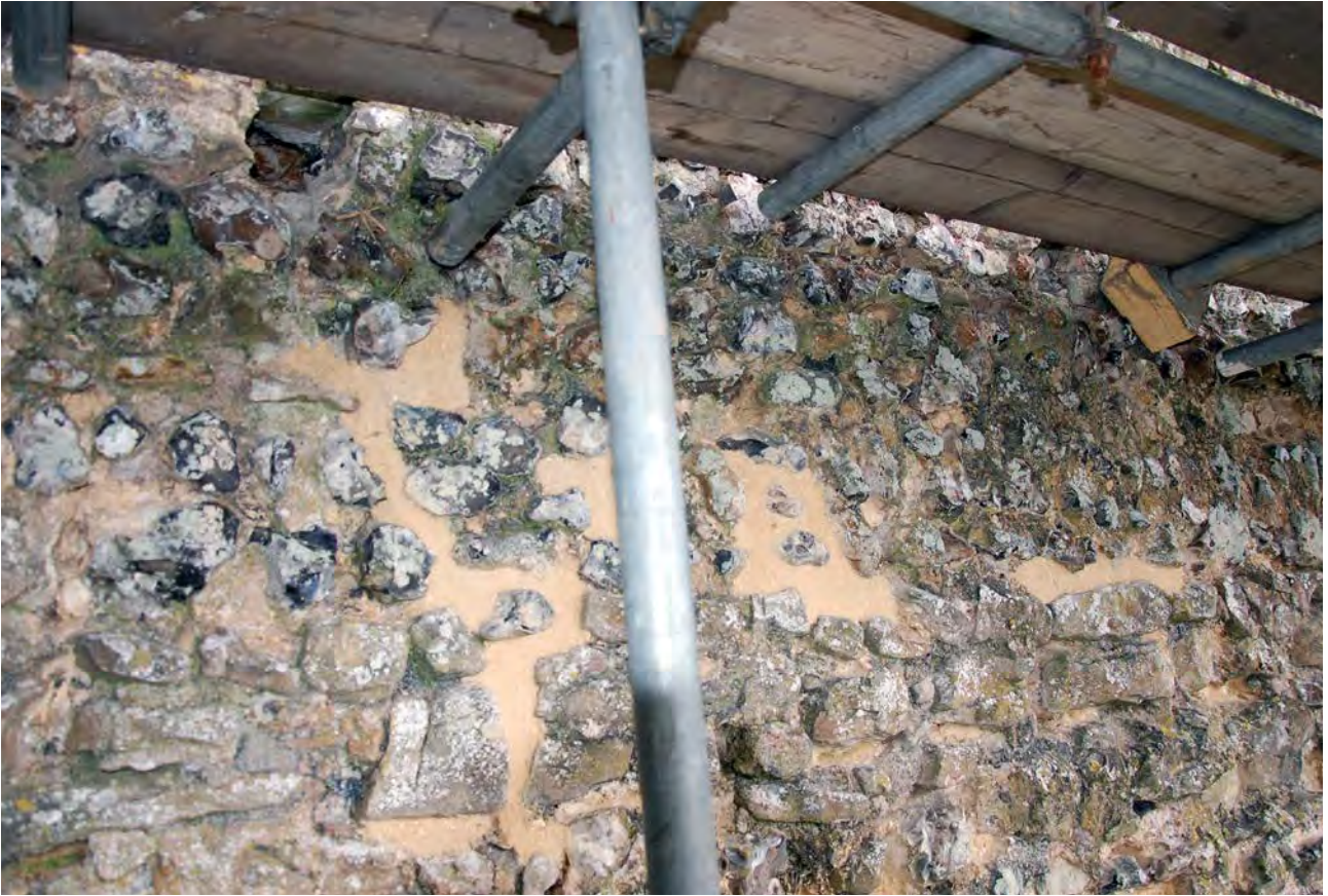
Plate 14: Voids A1 & A2, level 2 curtain wall
