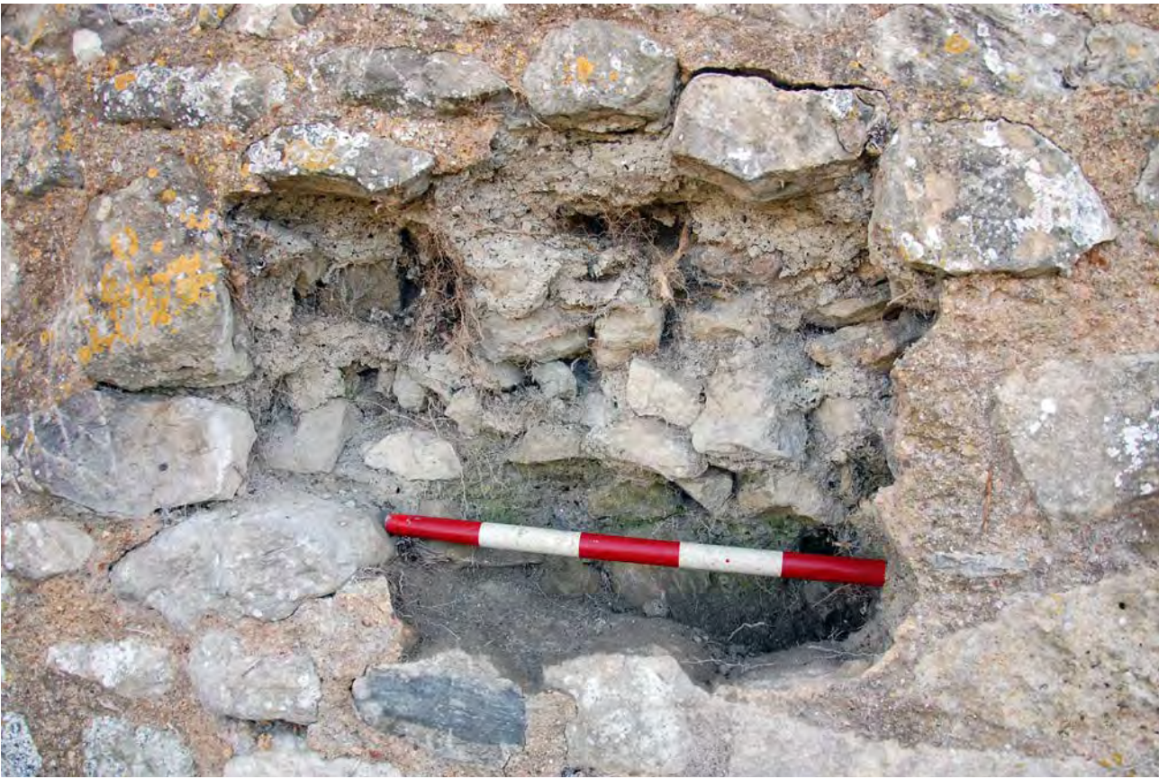
Plate 30: Void C at level 4
