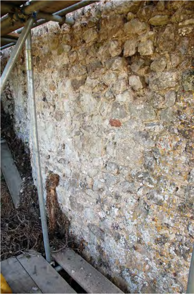
Plate 41: Void at level 6
