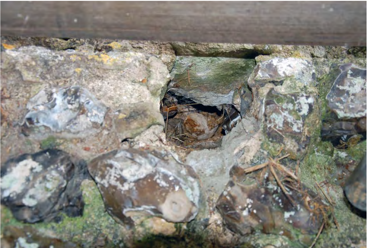
Plate 15: Void A1 at level 2
