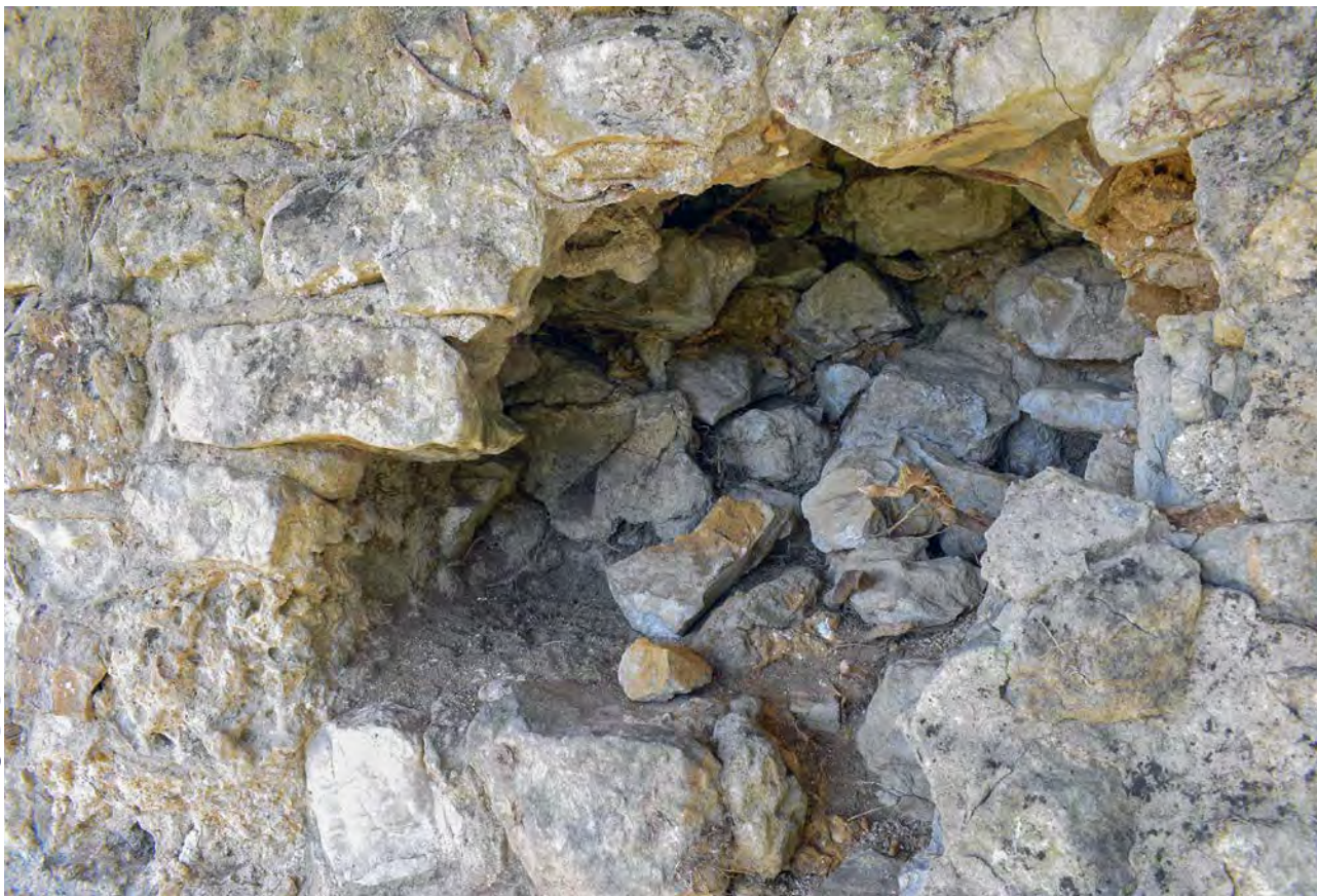
Plate 35: Void D1 (former putlog that has expanded)
