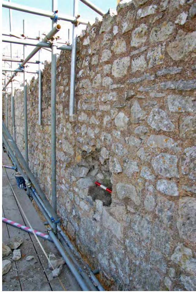
Plate 29: Void C at level 4
