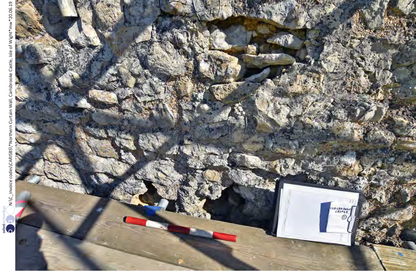
Plate 37: Void D4 at level 5
