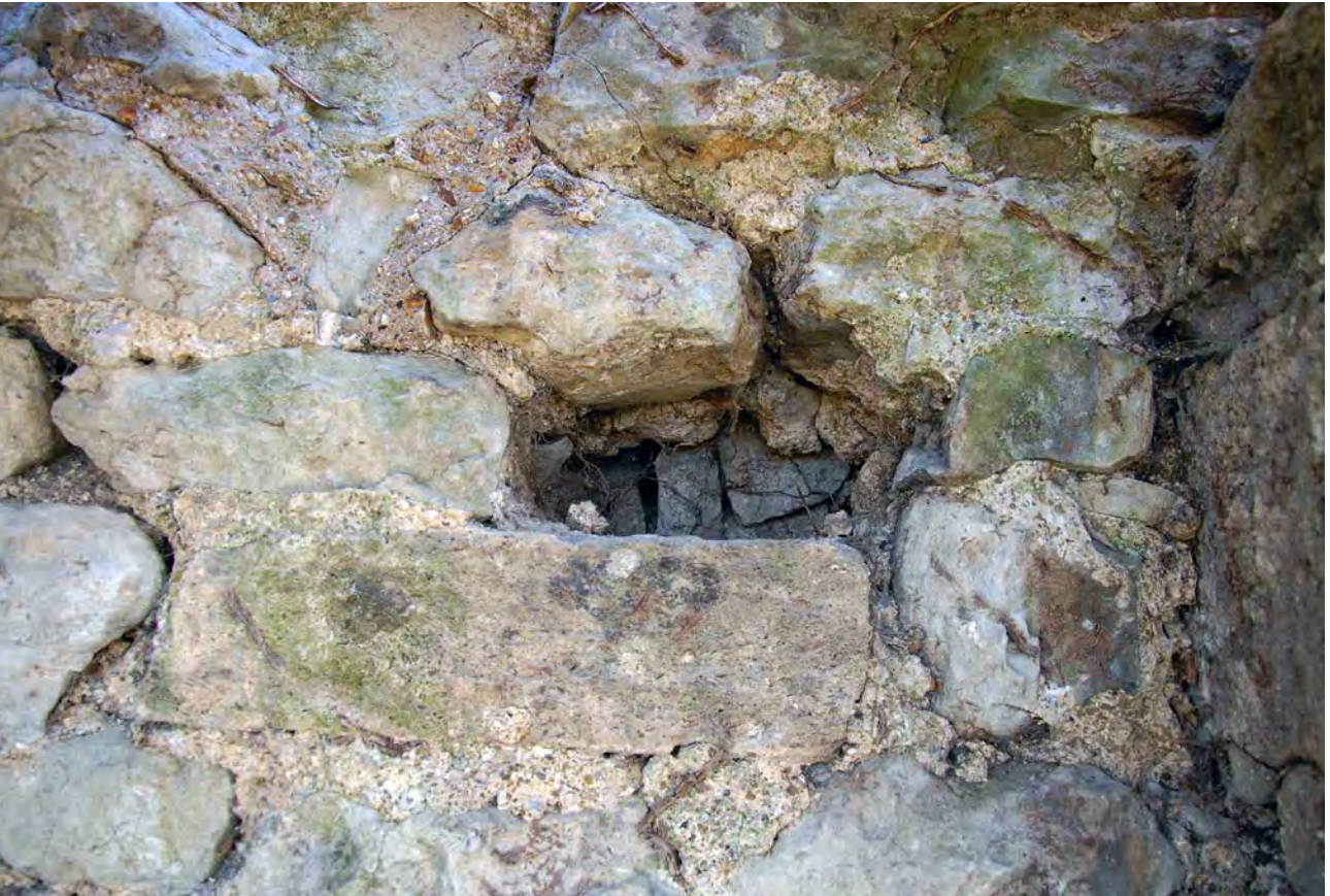
Plate 43: Small void at level 7
