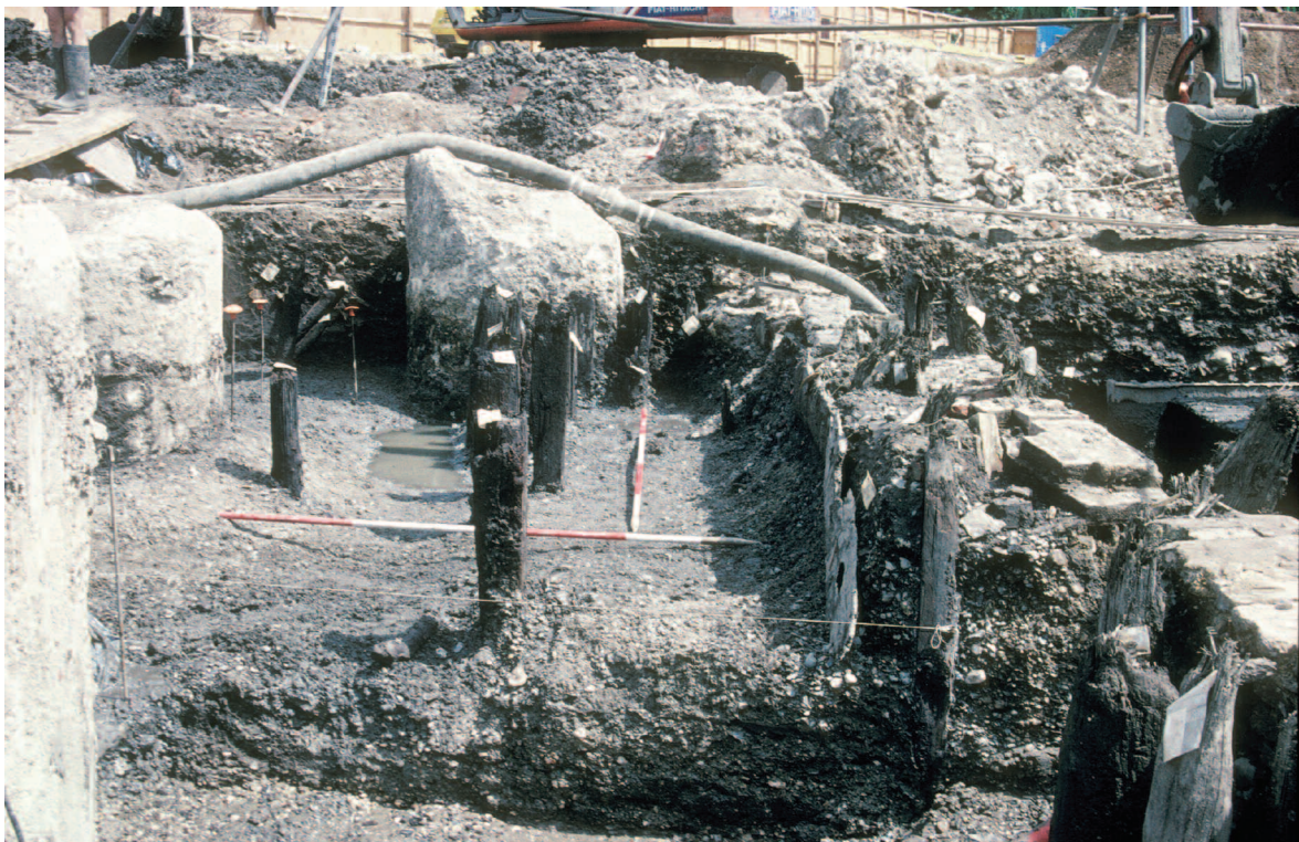
Plate 2.35 Site 101: view looking NE of 16th-century revetments of the northern bank of the Back Brook (Project Phase 6)
