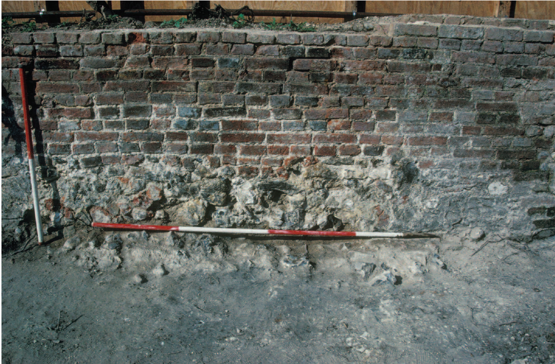
Plate 3.9 Site 29: view looking SW at the west wall (3967) of the west range of the workhouse (Project Phase 7)
