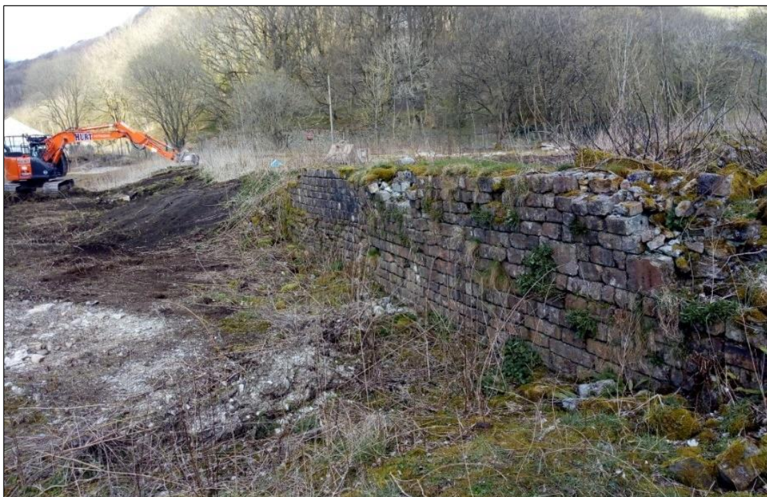
Plate 14: The extant element of the loading bay wall, showing removal of overburden
