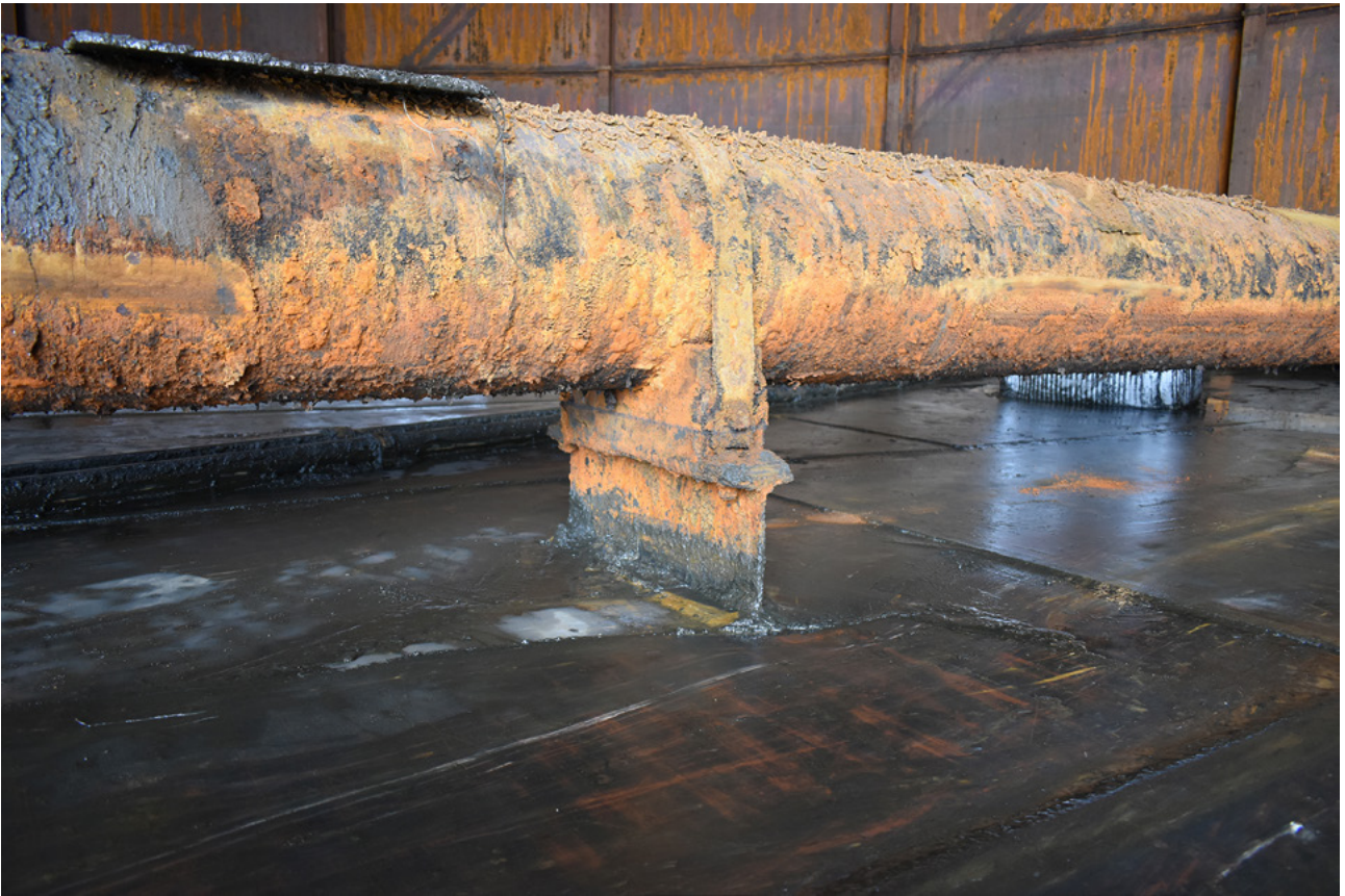
Plate 24: The inlet/outlet pipe support
