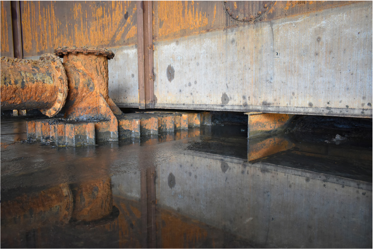
Plate 23: The inlet/outlet pipe in the interior of the gasholder
