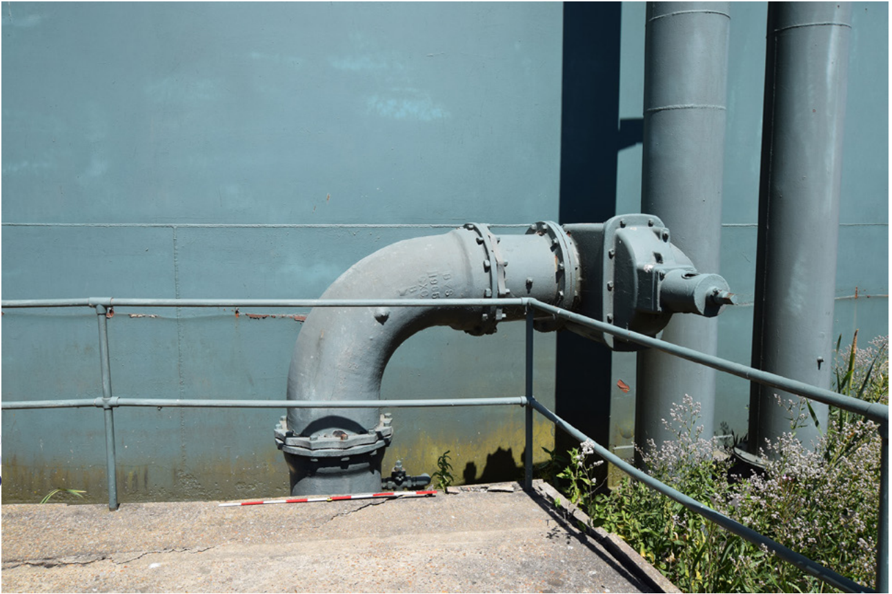
Plate 13: The inlet and outlet pipes, detail
