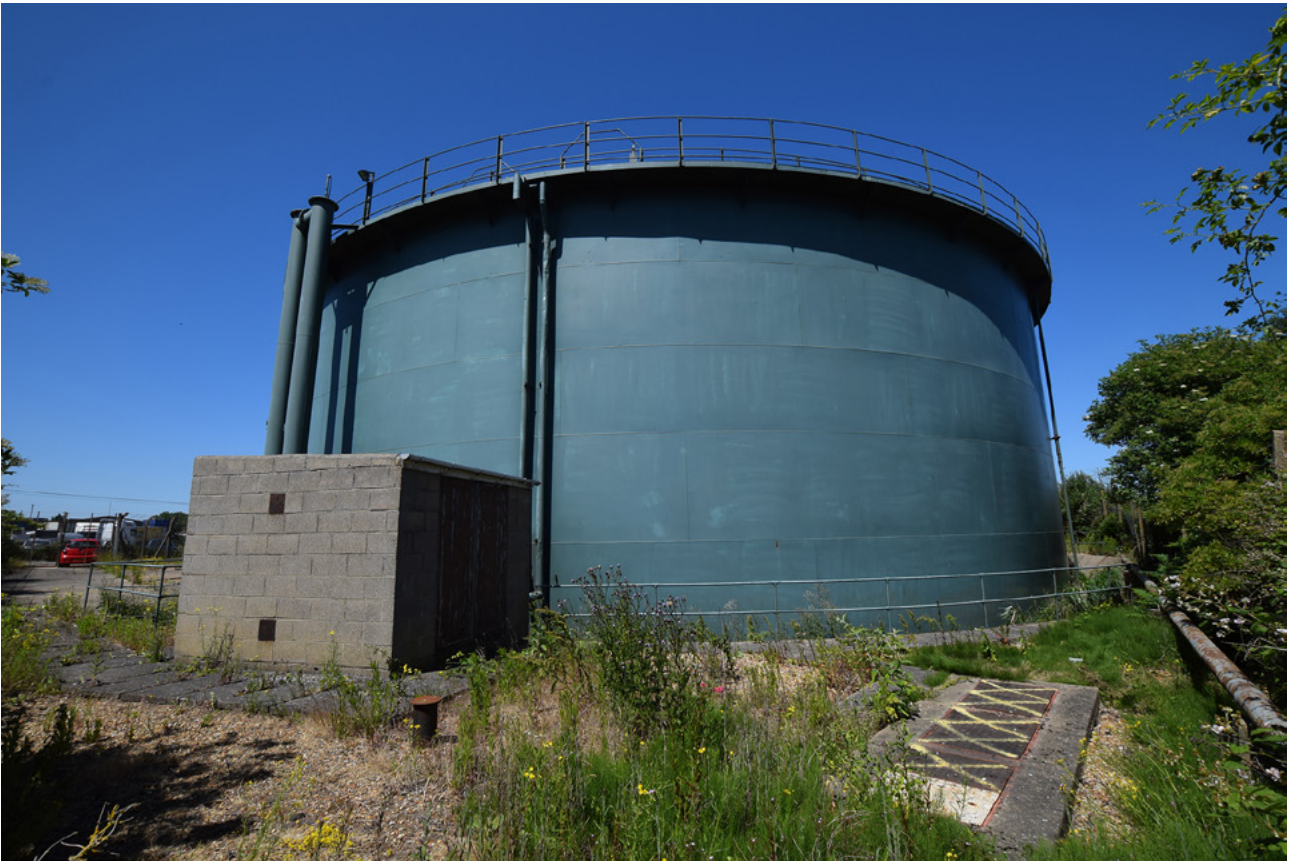
Plate 36: The concrete block building in relation to the gas holder, looking north
