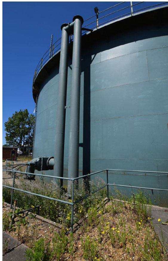
Plate 12: The inlet and outlet pipes
