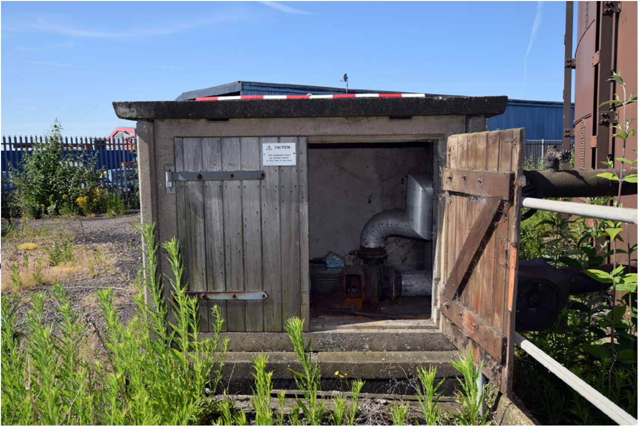
Plate 25: The doors of the concrete cabinet and the pump within
