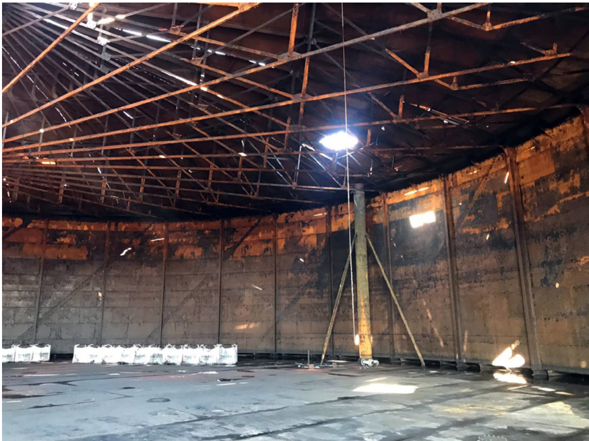
Plate 20: An inlet/outlet pipe and inner lift. Photograph provided by Erith Contractors Ltd
