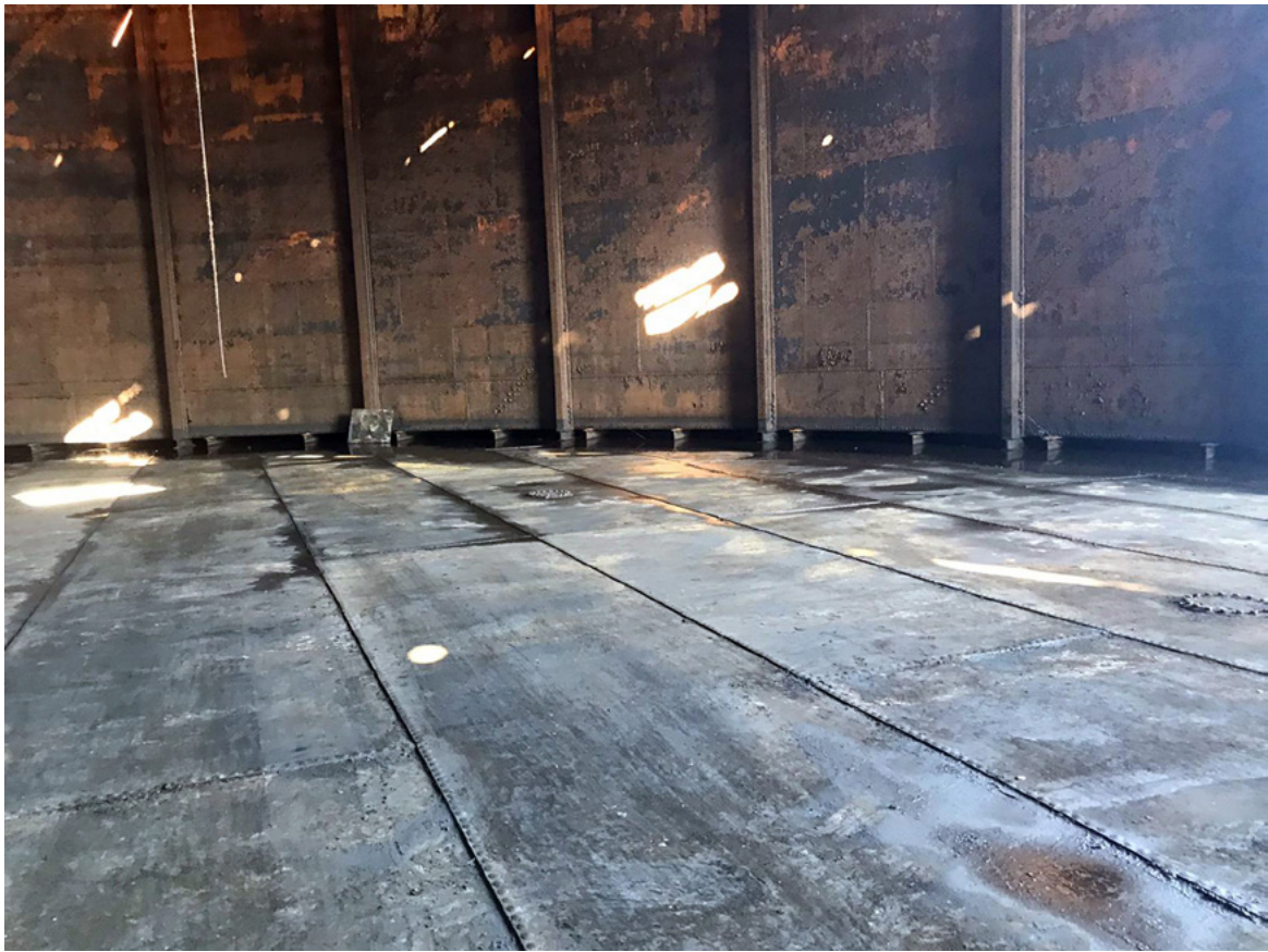
Plate 19: The base of the tank and inner lift. Photograph provided by Erith Contractors Ltd
