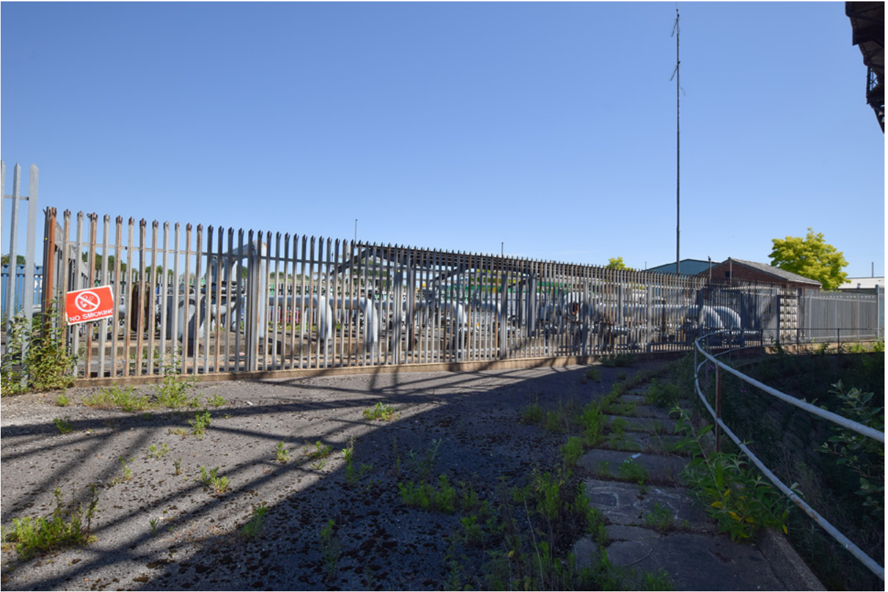
Plate 3: Gas Distribution Station
