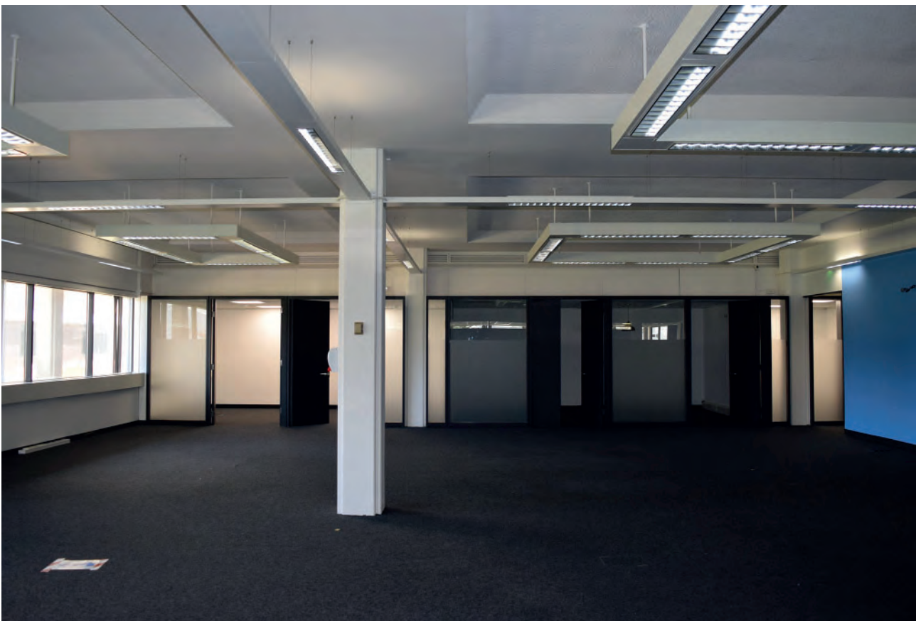
Plate 125: West wing of Building 6000, south office space, office cubicles set, looking north.
