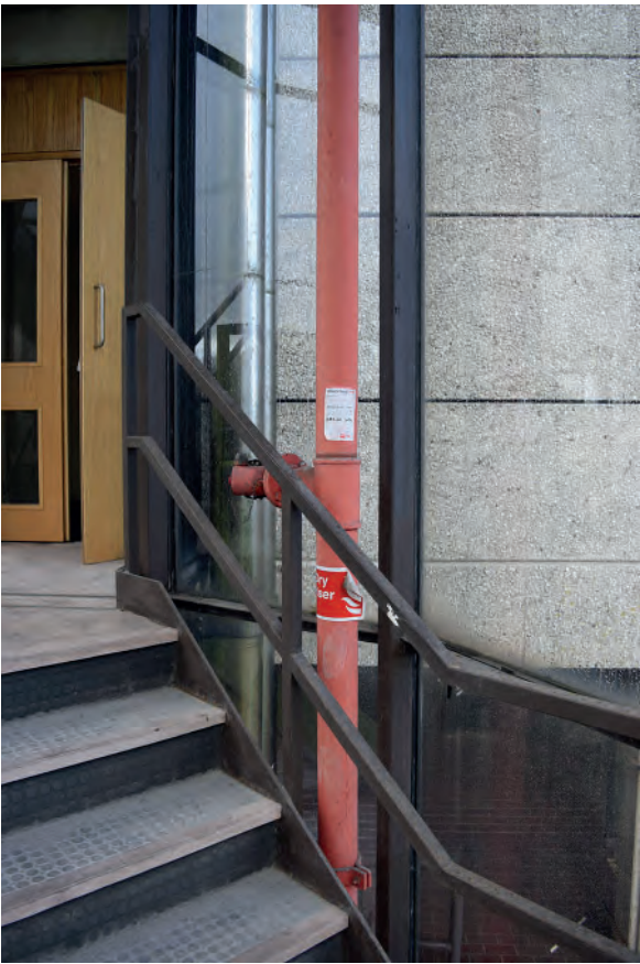
Plate 464: First Floor, hydrant, looking west.
