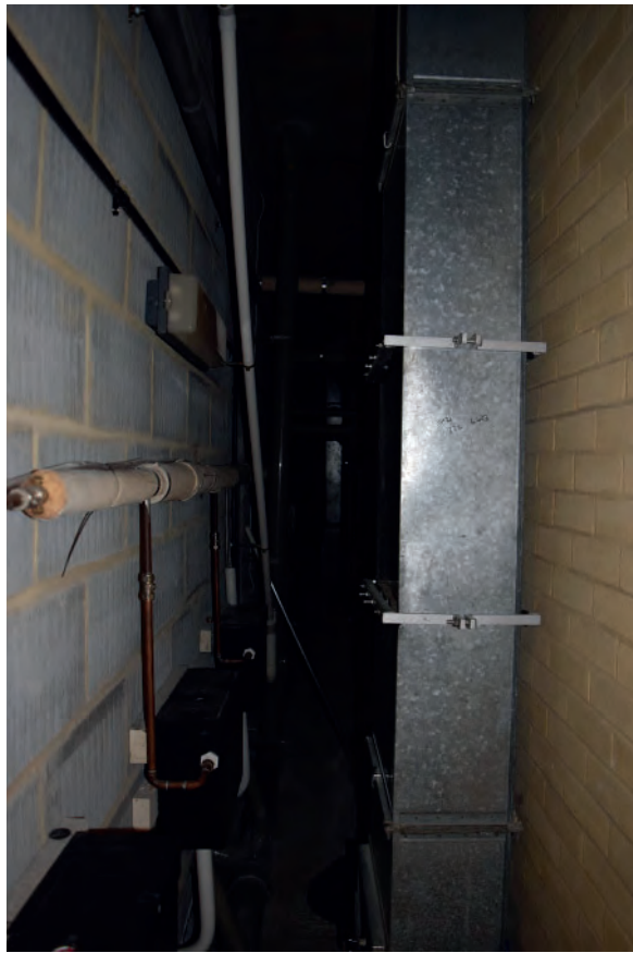
Plate 335: South part of Building 6000, west corridor, substation room, looking east.
