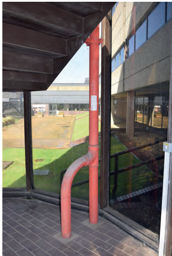
Plate 477: Ground Floor, hydrant, looking north.
