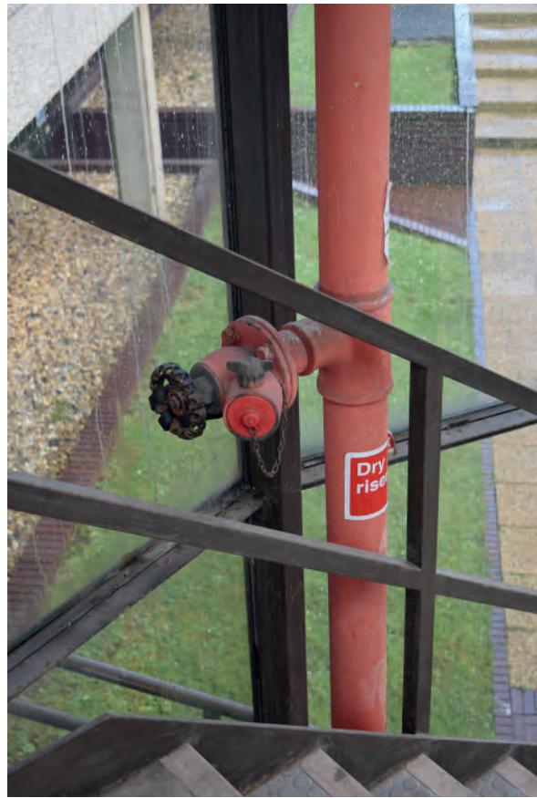
Plate 465: First Floor, hydrant, looking north.
