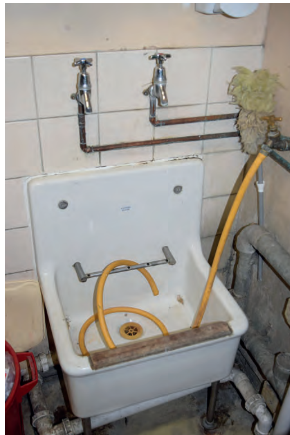
Plate 282: North part of Building 6000, north corridor, utility room, original sink, looking south- east.
