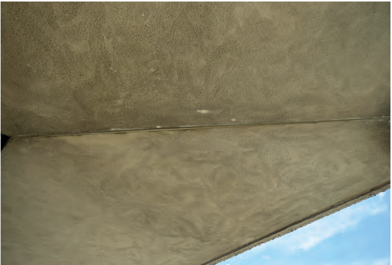
Plate 67: Southeast corner of Building 6000, detail of the concrete portico ceiling, looking north- east.
