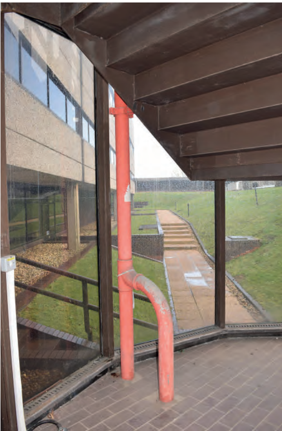
Plate 462: Ground Floor, hydrant, looking north.
