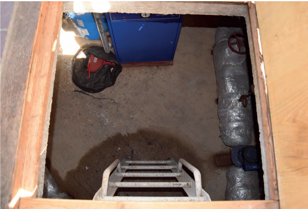
Plate 460: Technical room under ground floor.
