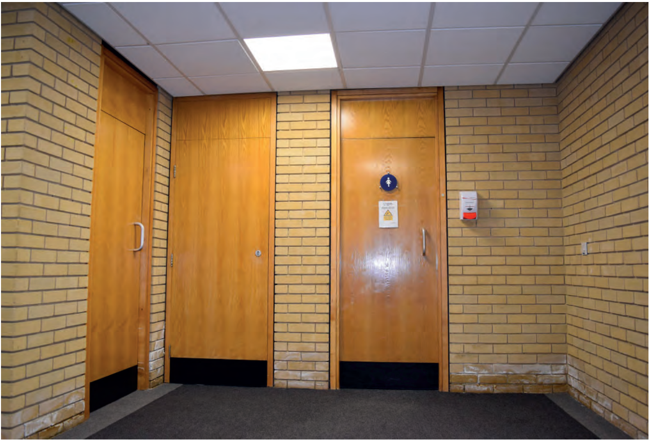
Plate 79: South part of Building 6000, west corridor, door to the women's toilet, looking east.
