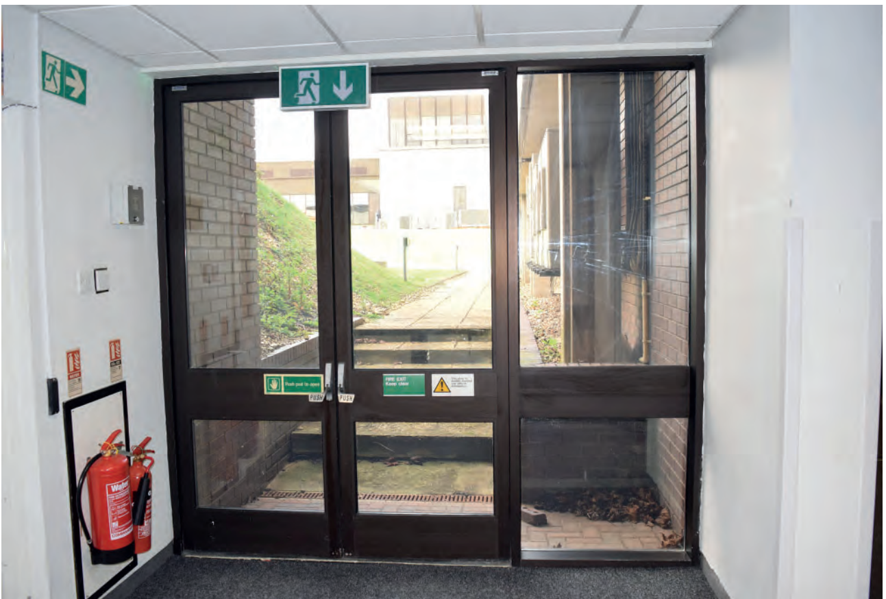
Plate 153: North part of Building 6000, connection between Buildings 6000 and 4000, eastern emergency door, looking east.
