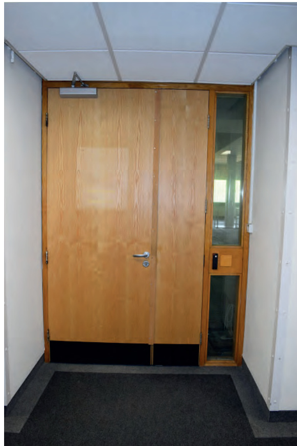
Plate 92: South part of Building 6000, east corridor, example of door to one of the offices, looking east.
