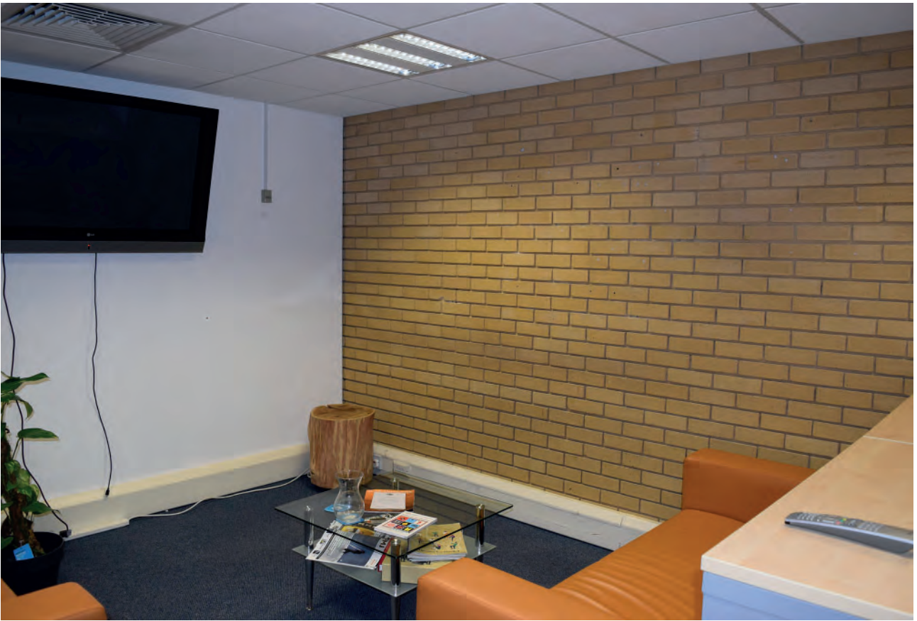
Plate 177: North part of Building 6000, office space along the north side of the courtyard, looking north-west.
