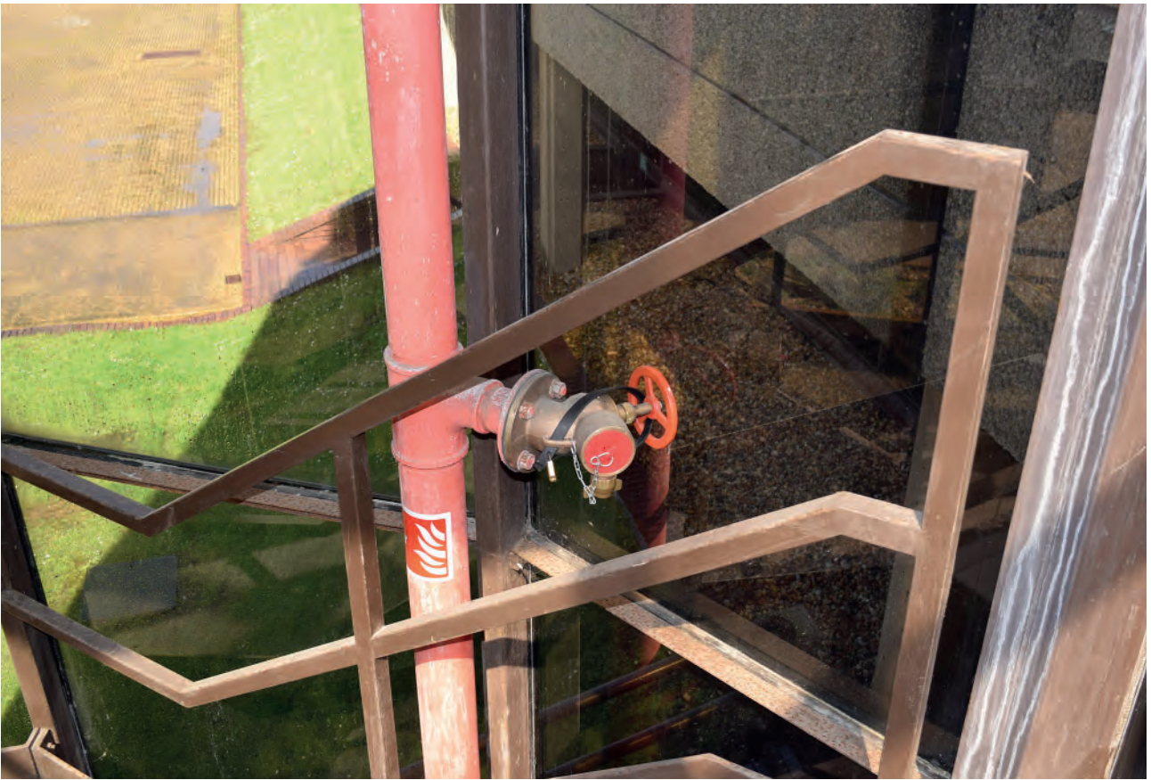
Plate 483: First Floor, hydrant, looking north.
