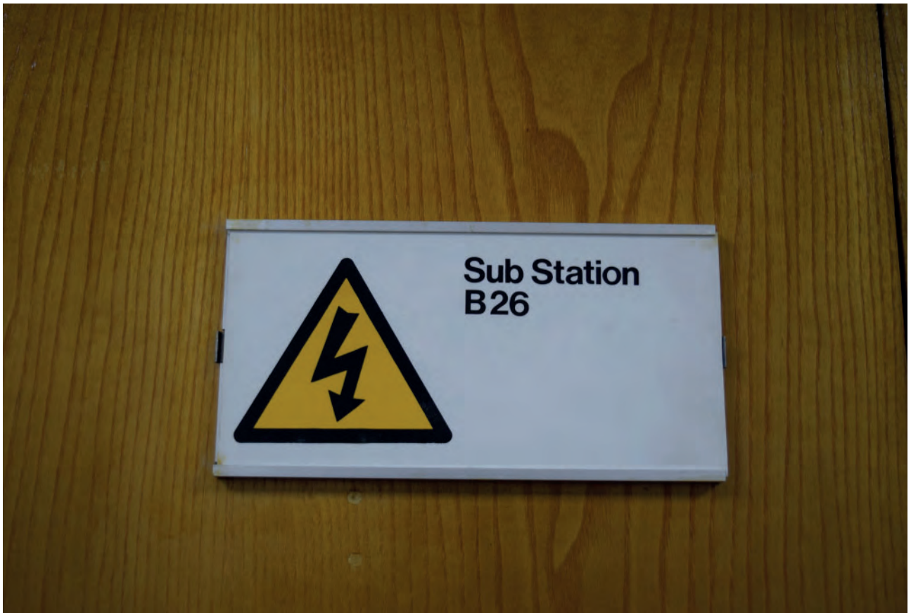
Plate 161: North part of Building 6000, sign on the door to the substation room, looking west.
