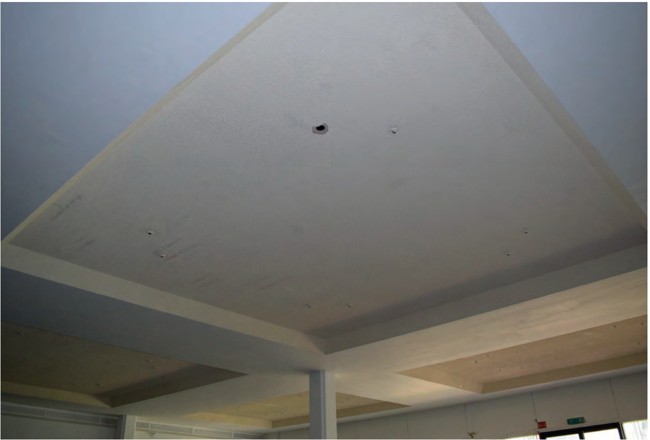
Plate 98: East wing of Building 6000, south office south office space, ceiling detail, looking north- west.
