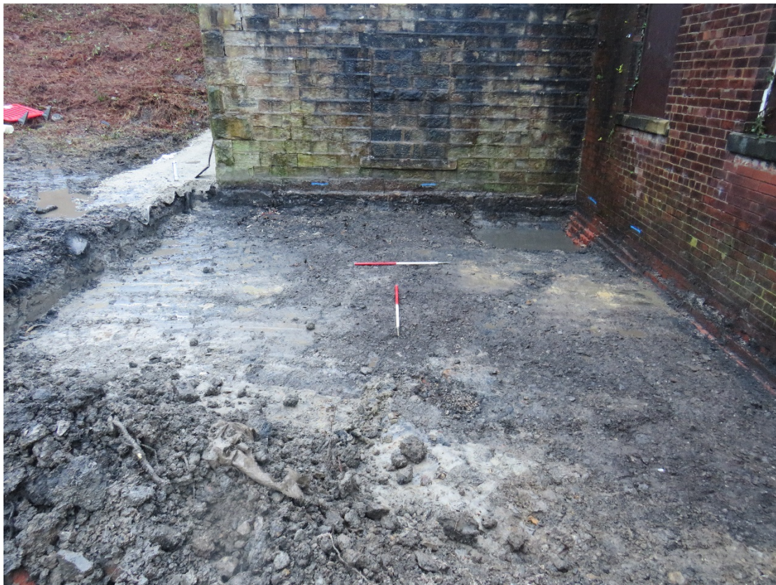
Plate 4. Reduced ground levels to the south and rear of Buildings 7-9. Viewed facing west.
