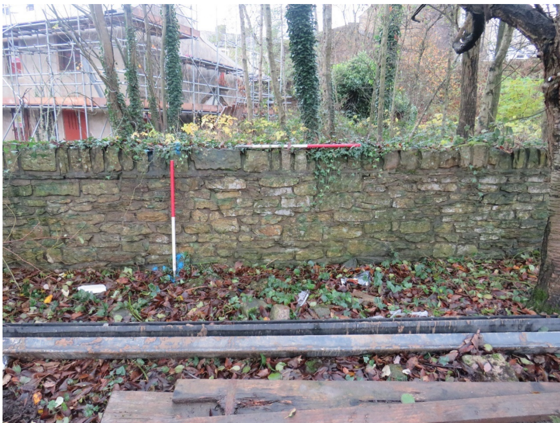
Plate 14. Continuation of retaining wall 202 north-east of the forge (Building 5), forming an external wall associated with Building 1 (distance).
