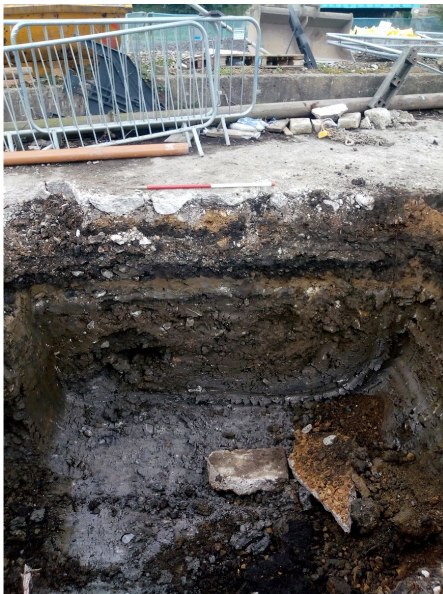
Plate 18. General shot of manhole 2 within the newly excavated service trench to the north of Buildings 7-9, showing general soil matrix encountered. Viewed facing east.
