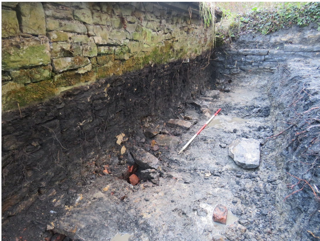
Plate 15. Culvert 202 exposed at the base of the southern wall of the forge (Building 5). Viewed facing east towards wall 201 .
