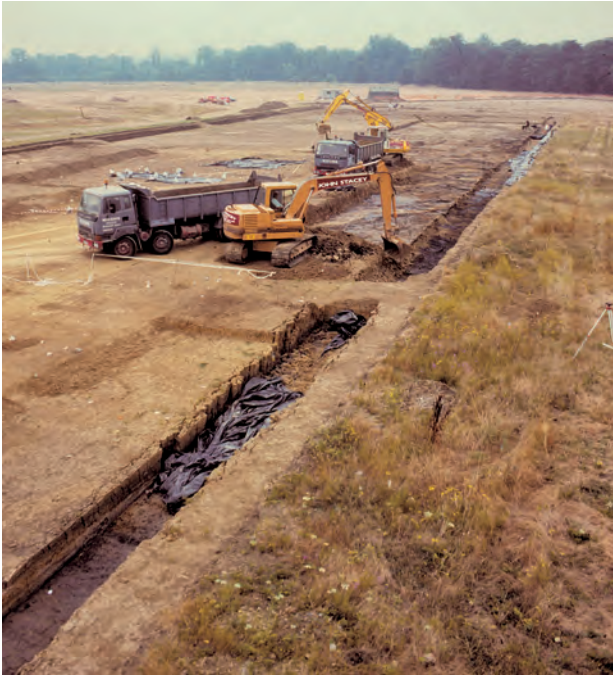
Plate 3.4 View of machine excavation on the floodplain in Area Ex1, looking south from above the palaeochannel (not in picture). The hut in the background is close to the edge of the gravel terrace.
