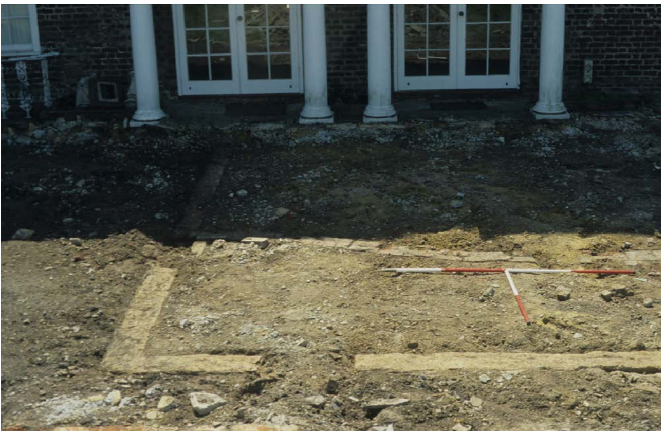
Plate 2: Ground reduction showing the foundations of the orangery, view to the south
