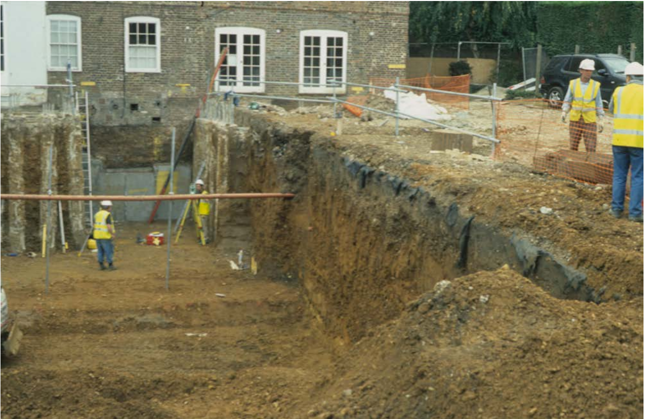
Plate 1: Basement construction to the rear of Clarence House, view to the south
