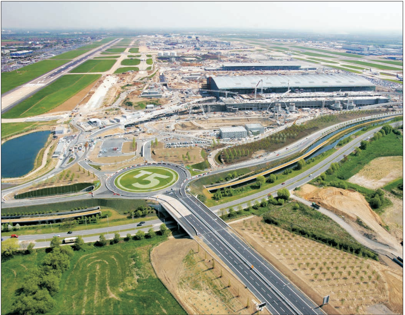
Plate 1.1: Heathrow Airport, aerial view of T5 construction site, May 2006 (© BAA Limited see www.baa.com/photolibrary )
