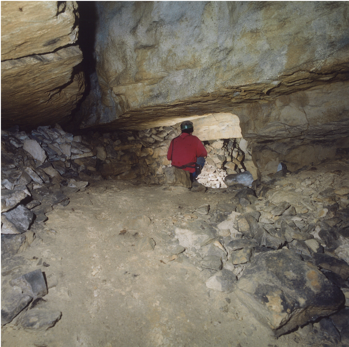
Fig. 7.3 Horsecombe Quarry, showing a large open joint or 'gull' which is parallel to the side of the escarpment resulting from cambering or land-slipping of the strata
