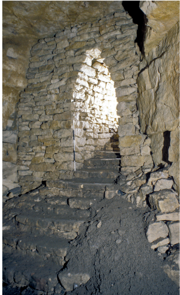
Fig. 7.11 Corbelled stone arch over the Hadley Arms steps. The stone pack was part of that supporting the North Road and the patina suggests it was built later than the steps (Photo by Paul Deakin)
