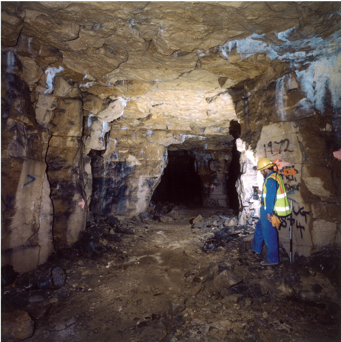
Fig. 7.4 Cartway within an adit or level entry (Allen's east cartway, central Firs) before stabilisation (Photo, Paul Deakin)
