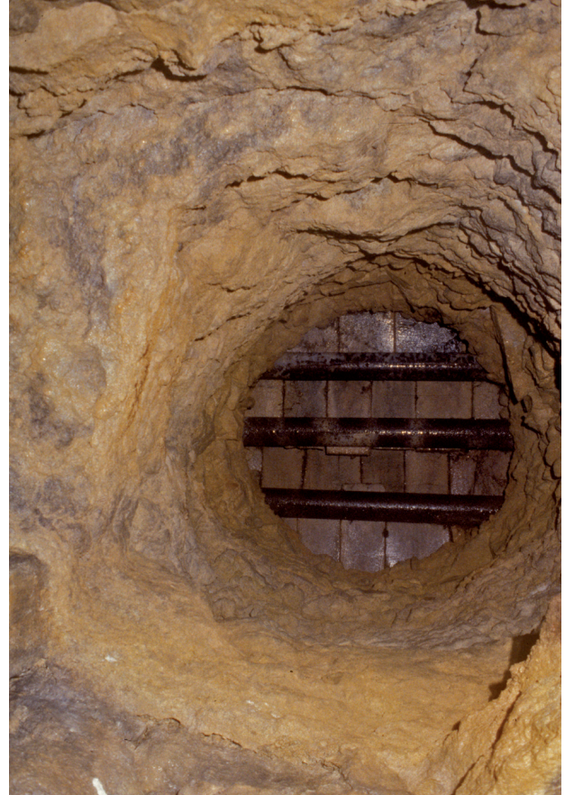
Fig. 7.9 Small ventilation shaft in the roof of the workings, with cap formed of stone slabs over timber supports, Central Firs
